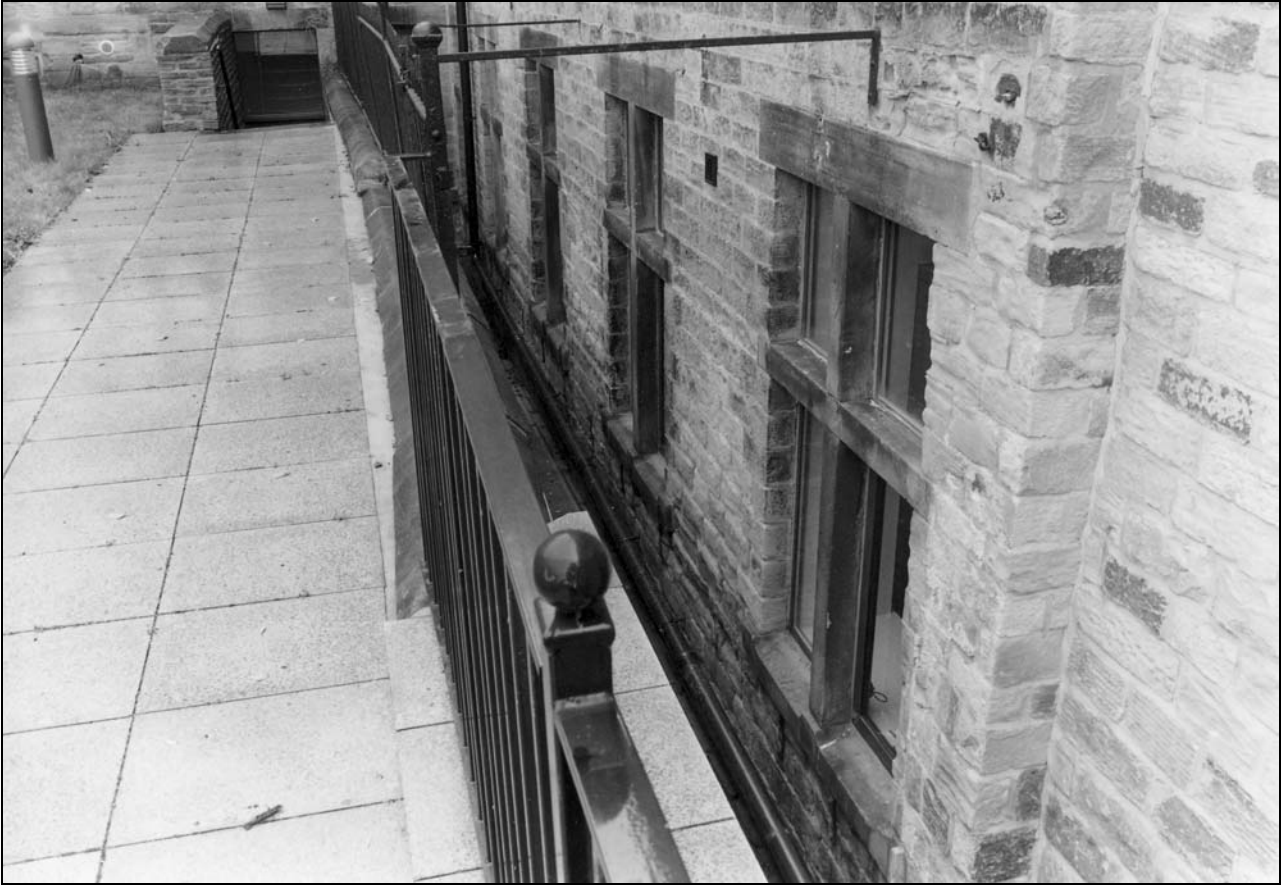
Photo 36: Light well along south side of north wing, from the east (film 3, frame 6)
