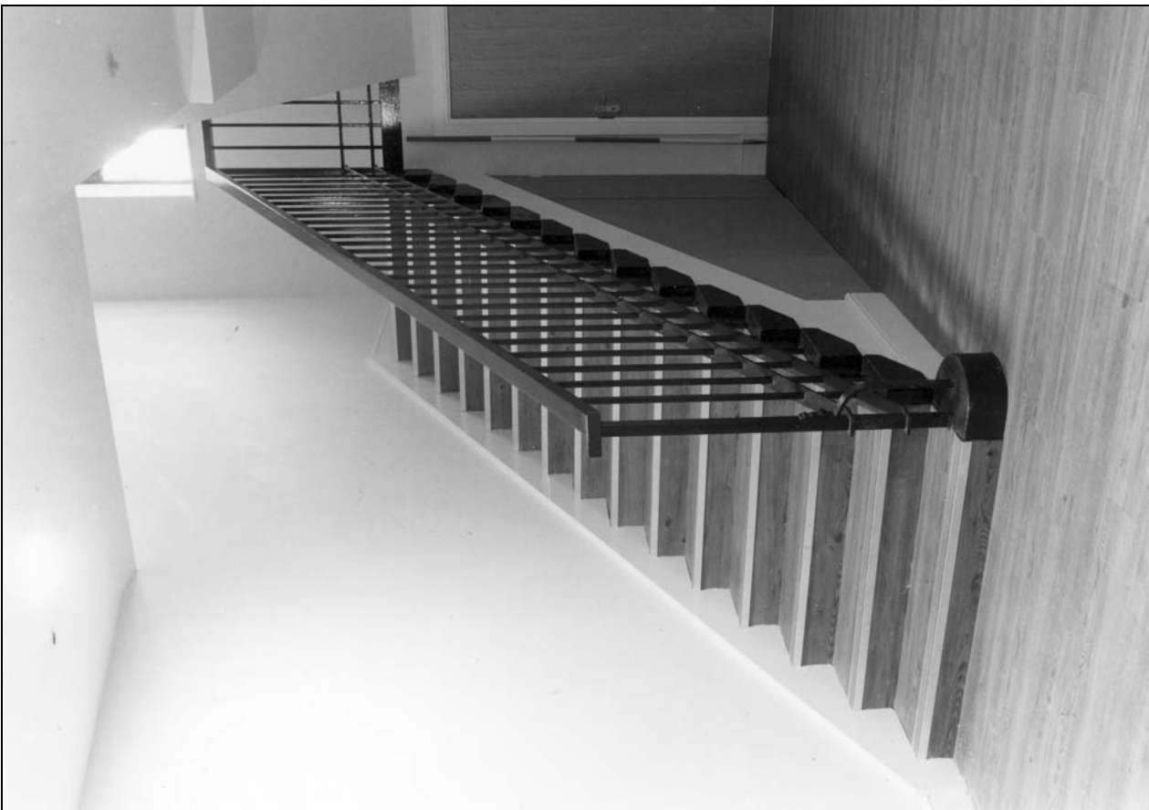
Photo 41: Staircase on ground floor of boys' end of school, from the north-east (film 4, frame 1)
