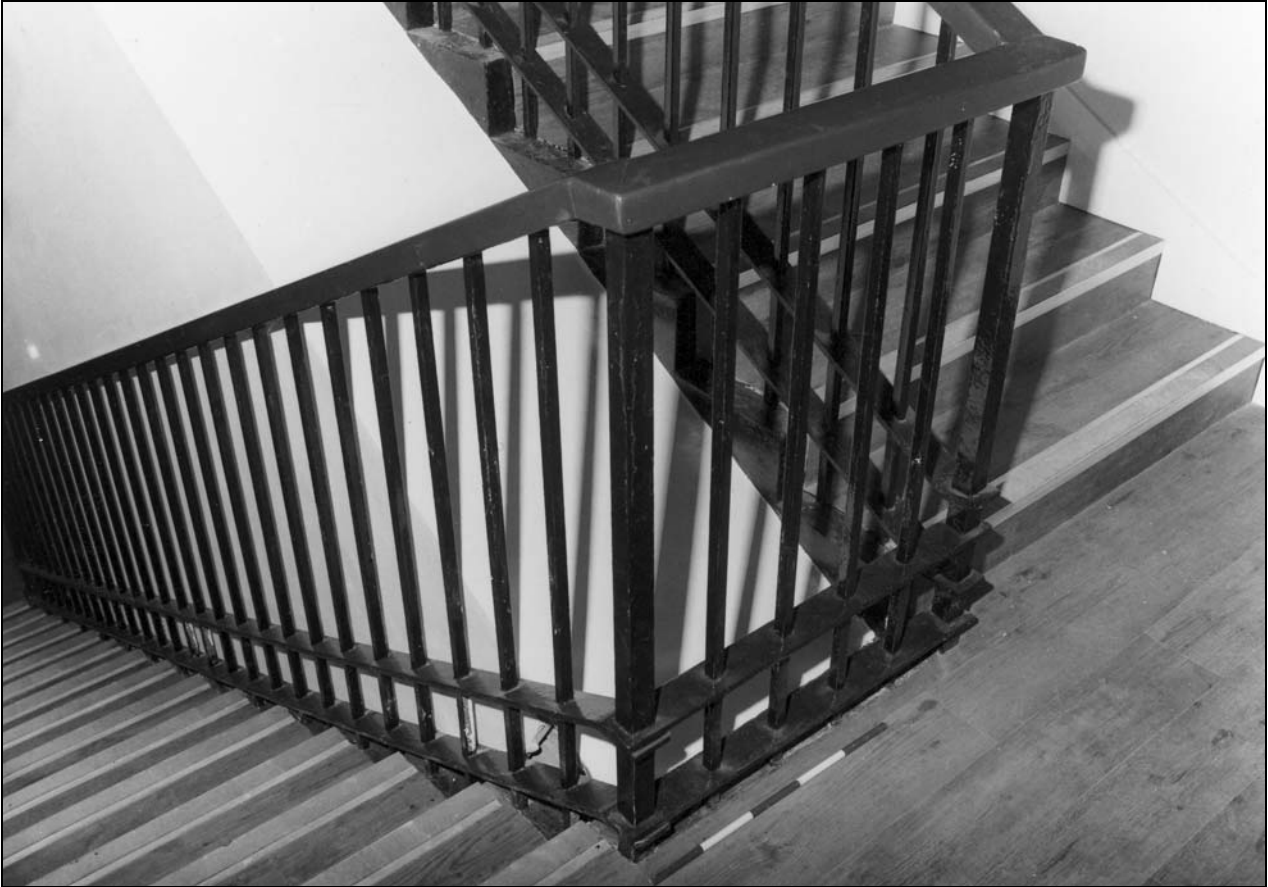
Photo 43: Staircase landing in girls' end of school, from the north-west (film 4, frame 3)
