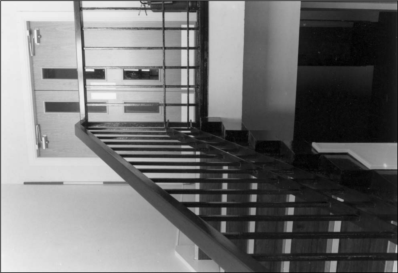
Photo 42: Staircase up to ground floor of boys' end, from the north (film 4, frame 2)
