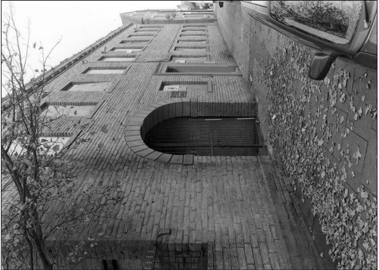
Photo 4: Front elevation of the two storey block, from the west (film 1, frame 12)
