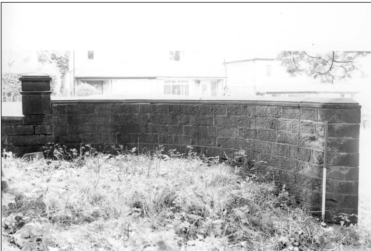
Photo 8: Quadrantic boundary wall at north side of entrance, looking east (film 1, frame 14)
