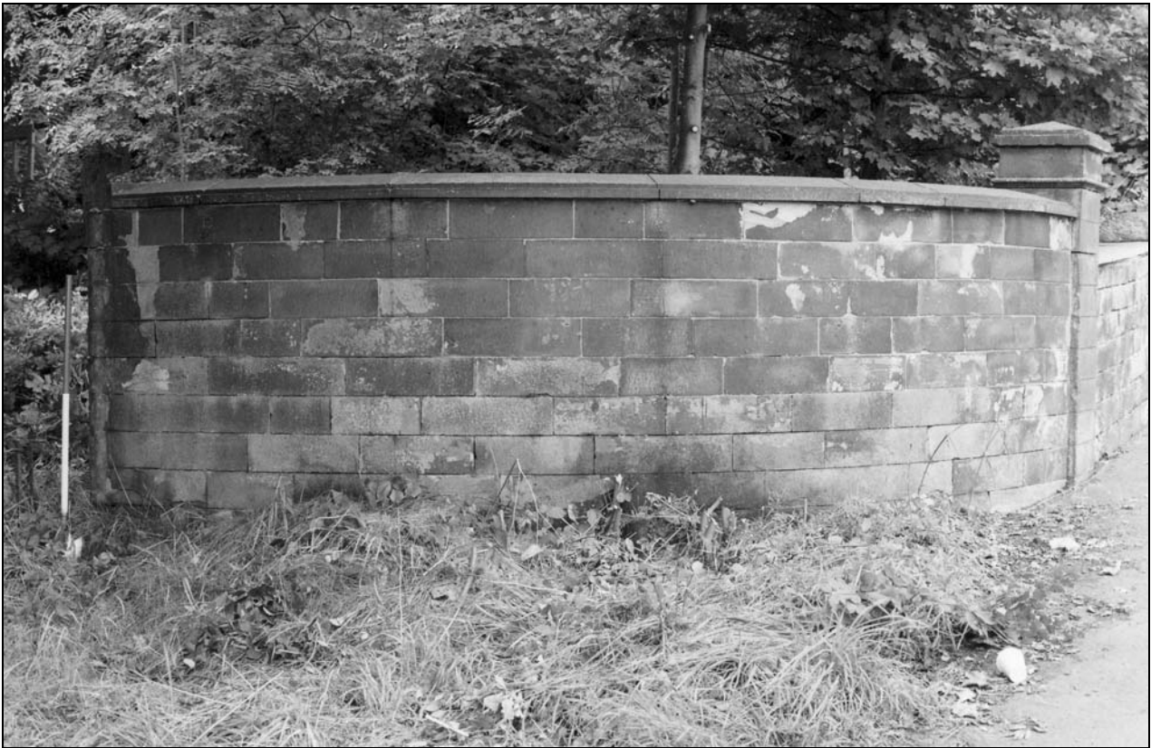
Photo 7: Quadrantic boundary wall at north side of entrance, looking north-west (film 1, frame 8)
