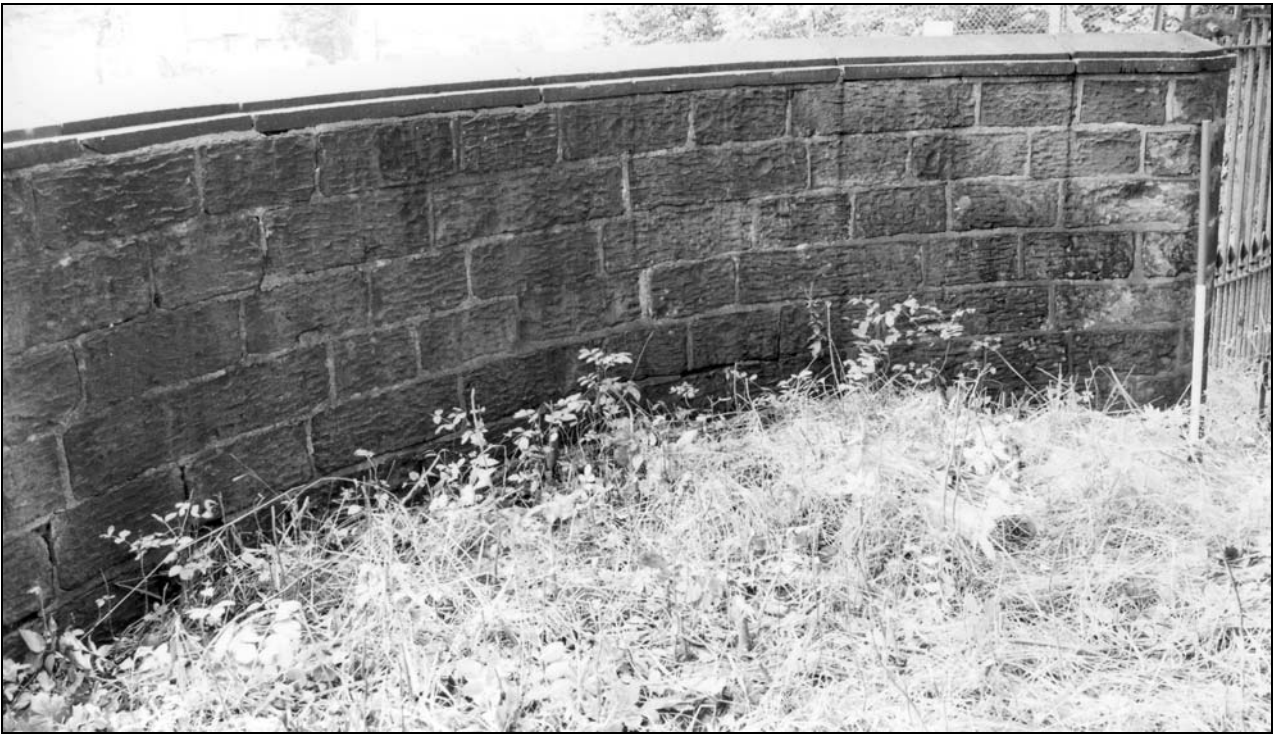
Photo 9: Quadrantic boundary wall at north side of entrance, looking south-east (film 1, frame 17)
