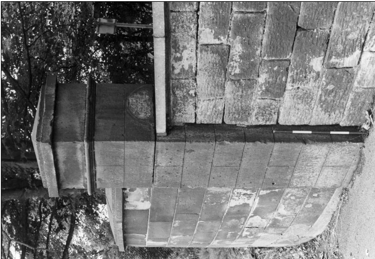
Photo 3: Stone boundary wall and gate pier at north end of entrance, looking south-west (film 1, frame 10)
