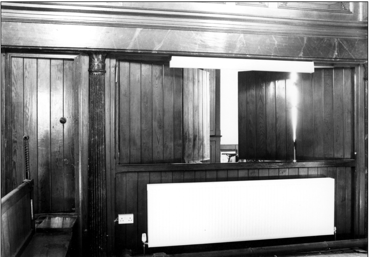
Photo 23: Partition with shutters in east side of main room, looking east (film 2, frame 2)
