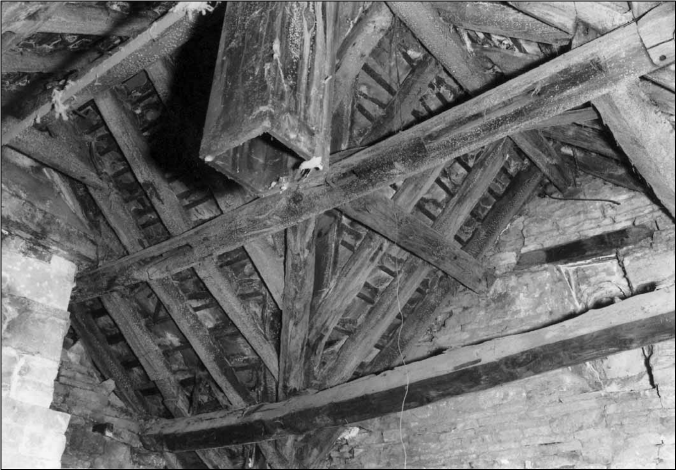
Photo 46: Underside of roof in north bay of 17th century wing, looking north-east, showing reused timbers (film 3, frame 6)
