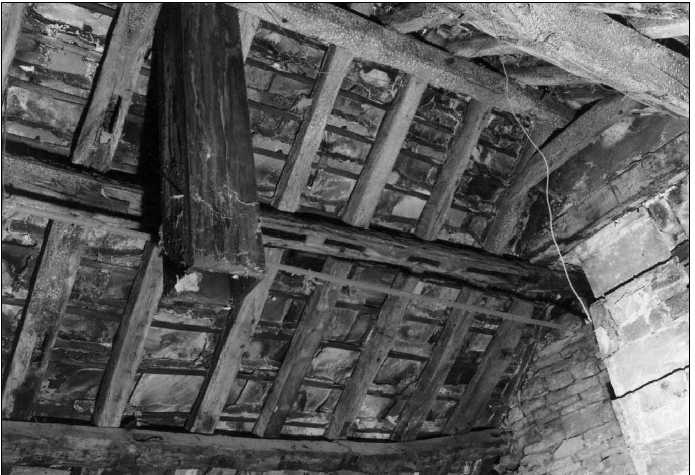
Photo 45: Underside of roof in north bay of 17th century wing, looking north-west, showing reused timbers (film 3, frame 5)
