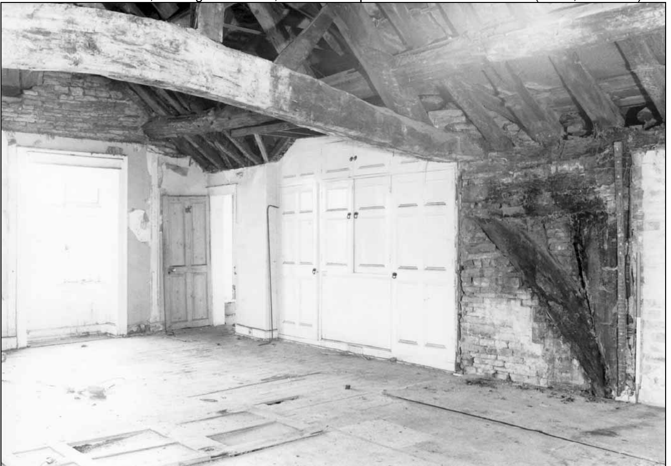
Photo 32: First floor, looking south-west, with arcade post and arch brace visible (film 3, frame 13)
