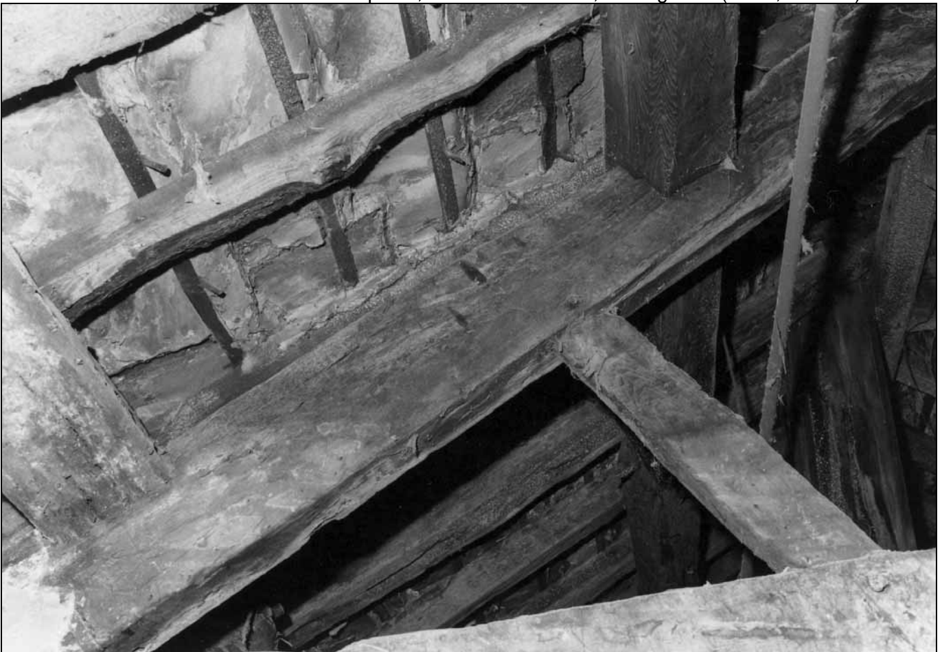
Photo 49: Candle soot marks on south side of west principal rafter, north truss (film 4, frame 12)
