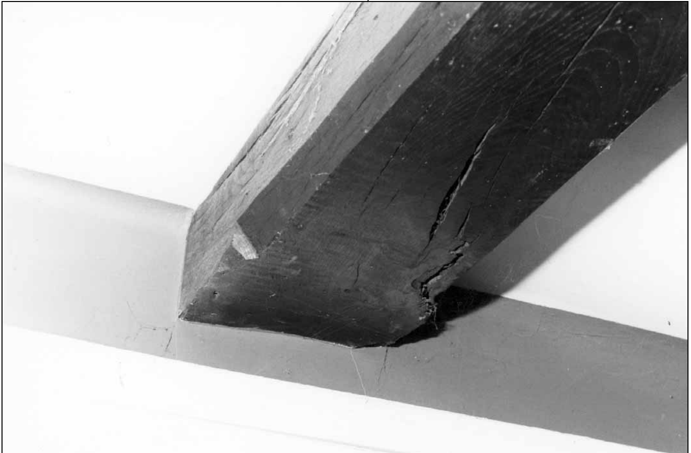
Photo 13: Stop-chamfered ceiling beam, ground floor of east wing, south room (17th century dining room) (film 1, frame 7)
