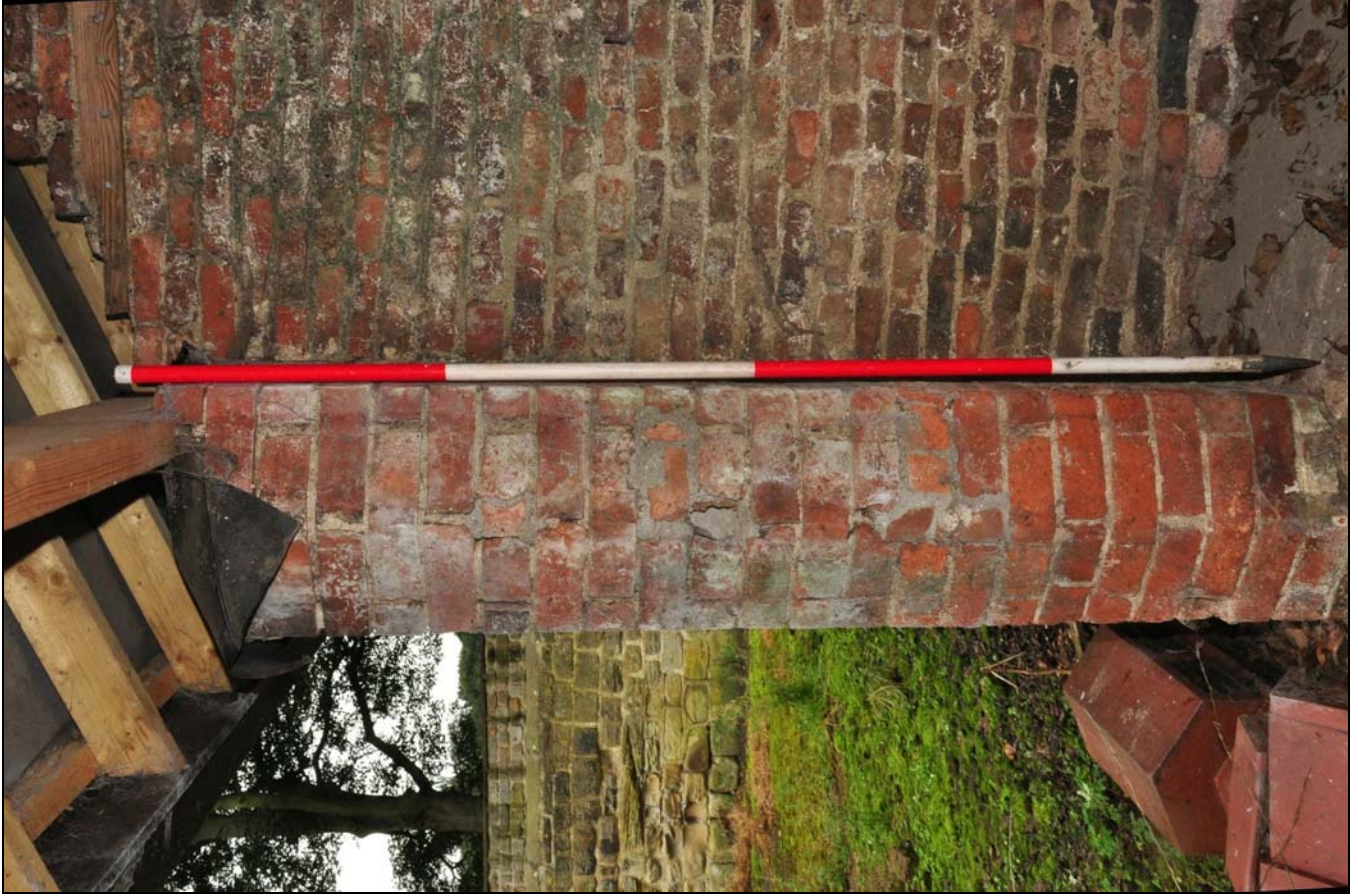
Photo 53: Detail of brick pier between bays 2 and 3 of rear lean-to, looking south-east
