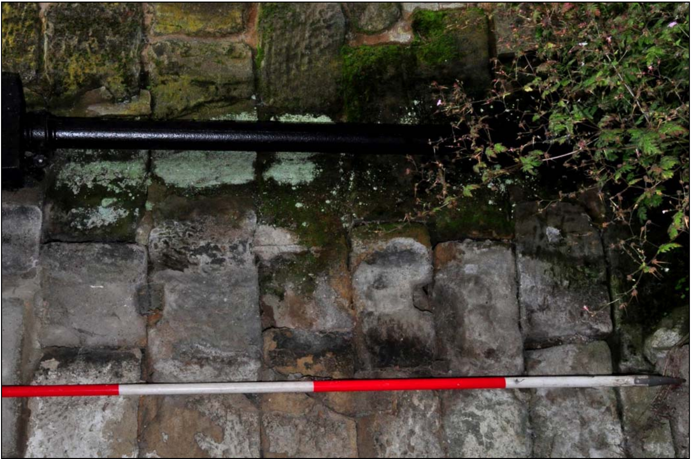
Photo 54: Detail of sockets for horizontal poles in yard wall next to bay 3 of rear lean-to, looking north-west
