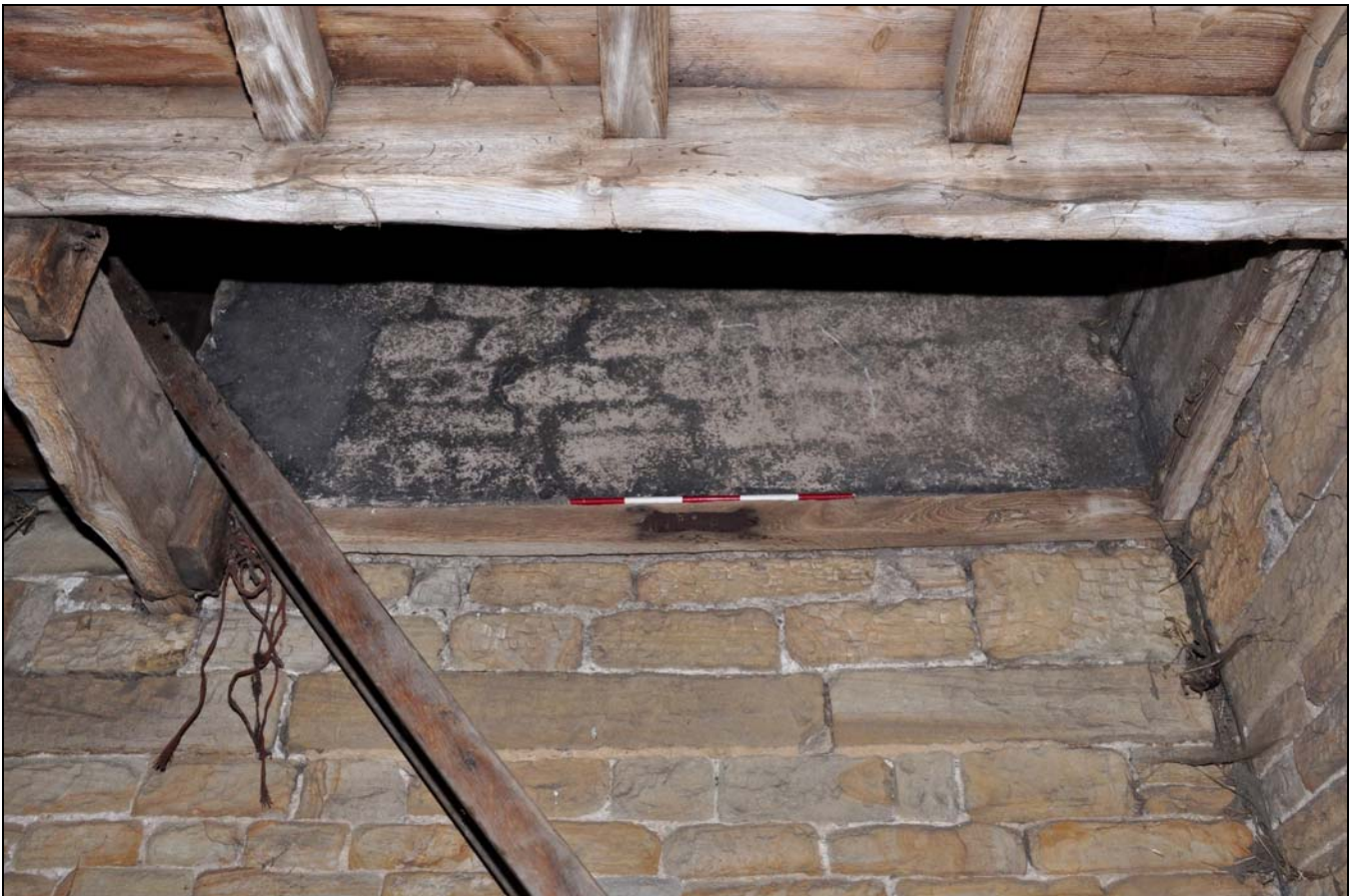
Photo 20: Trap over ground floor (access to first floor, formerly with door), looking south-east
