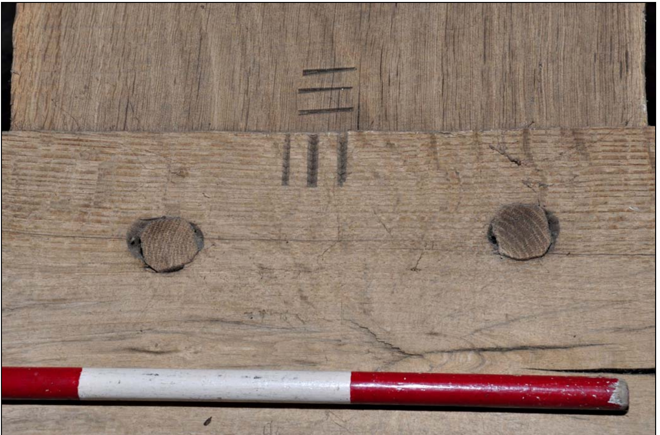
Photo 46: Detail of joint numbering on collar at foot of king-post, south-east truss
