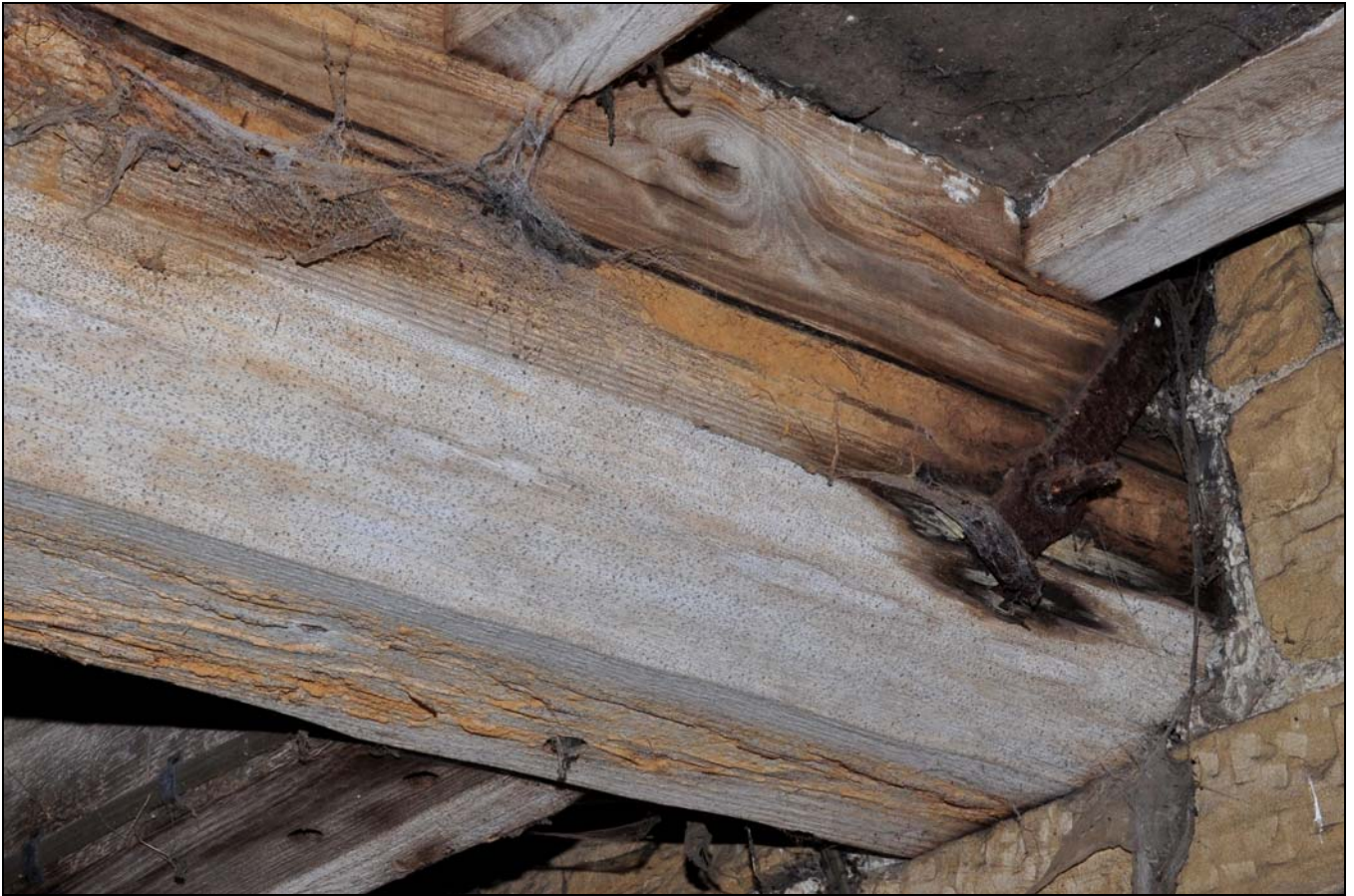
Photo 25: Detail of iron strap at end of ceiling beam, south-west side of ground floor
