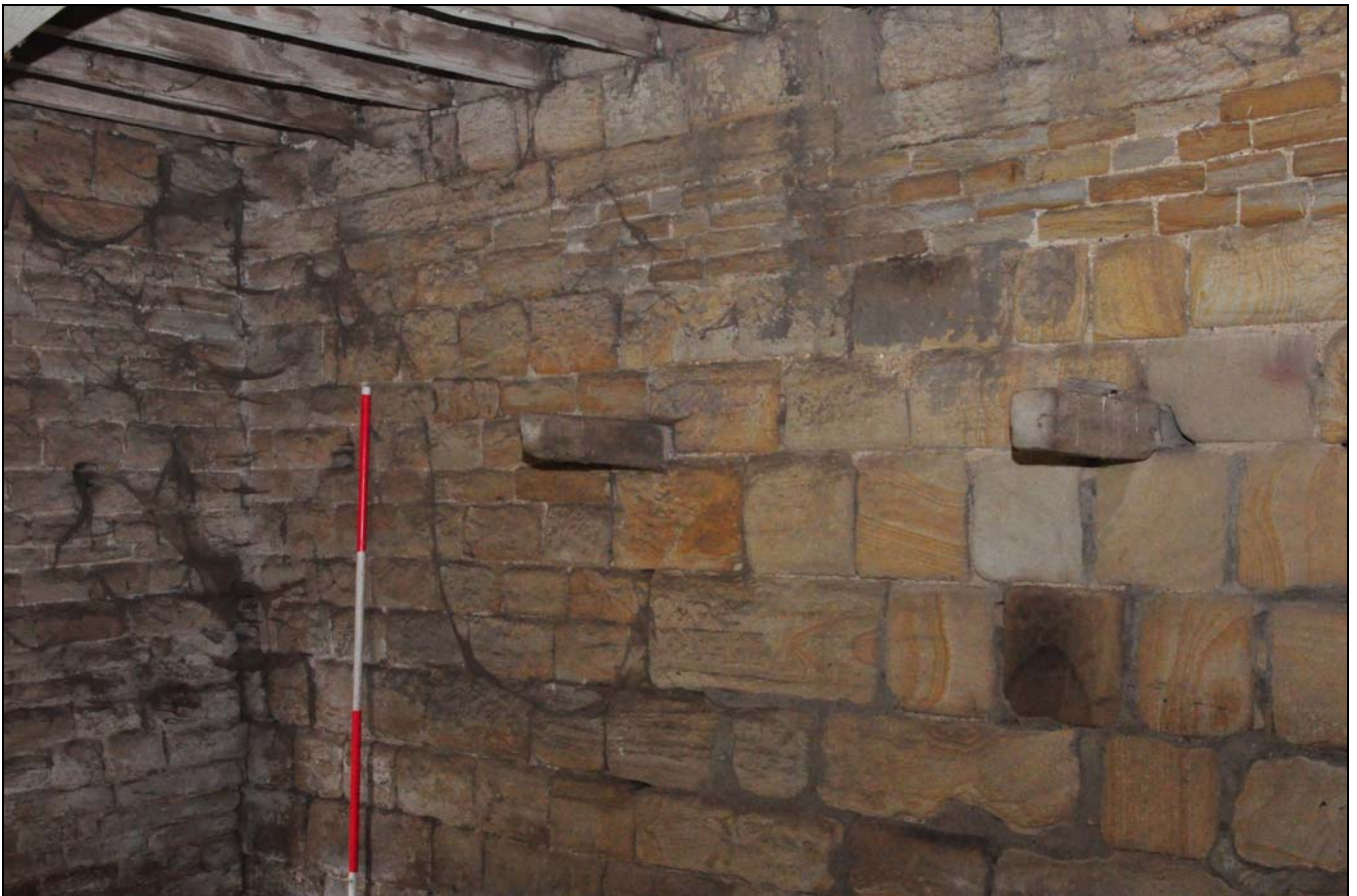
Photo 22: Ground floor of cart-shed, looking towards west corner, with oak brackets in wall
