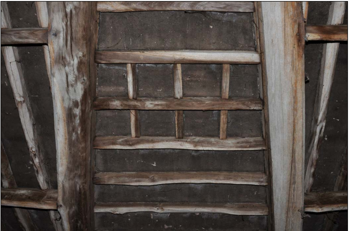
Photo 26: Underside of first floor in centre of building, with reinforcement for gangway
