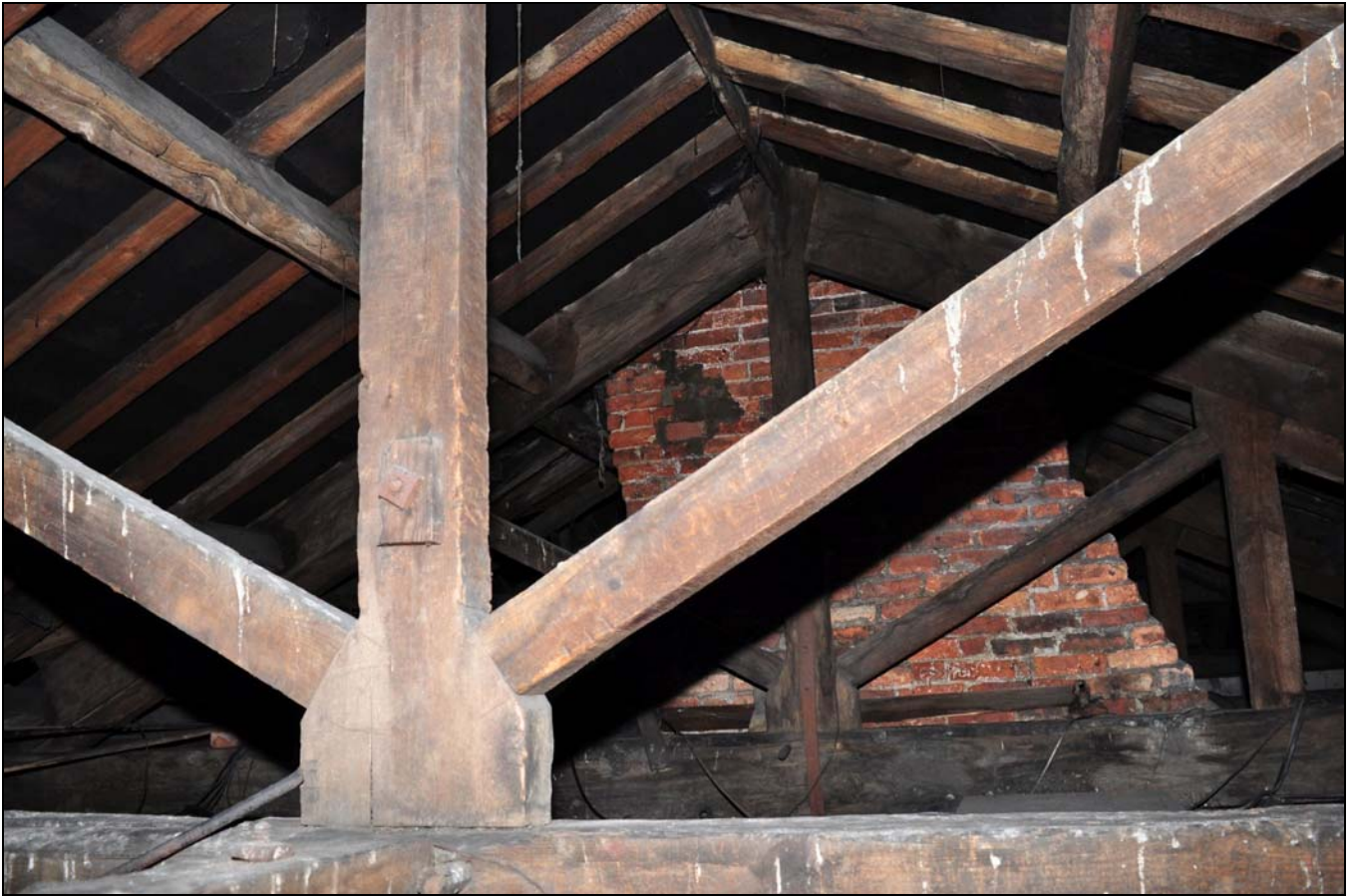
Photo 133: Roof space and part of a roof truss over front range, looking south
