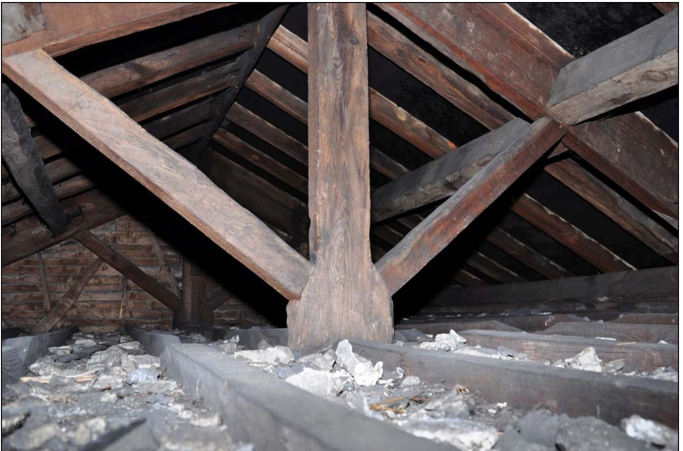
Photo 134: Roof space and part of a truss over east part of rear range, looking south
