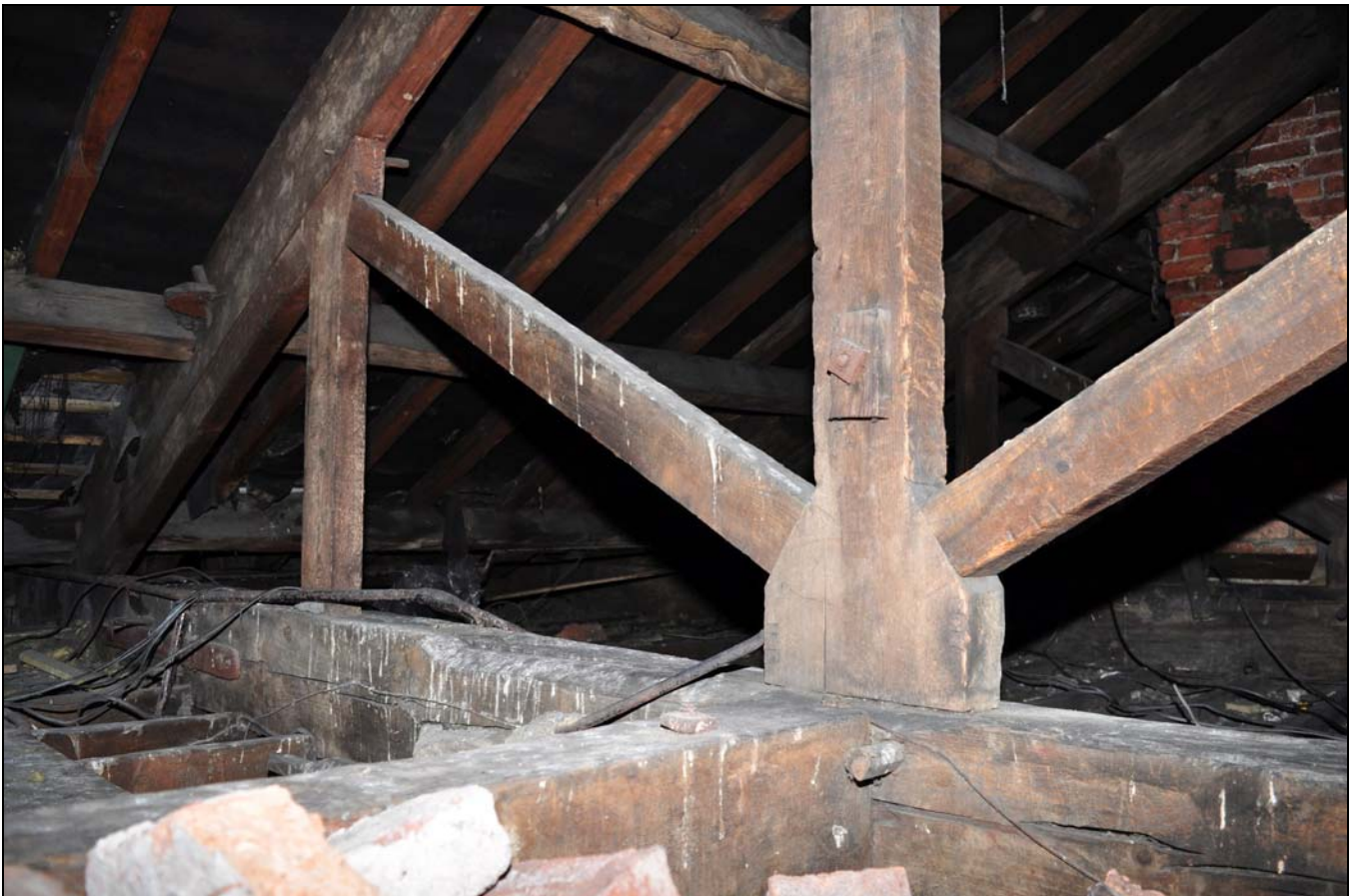
Photo 132: Roof space and part of a truss over front range, looking south-east
