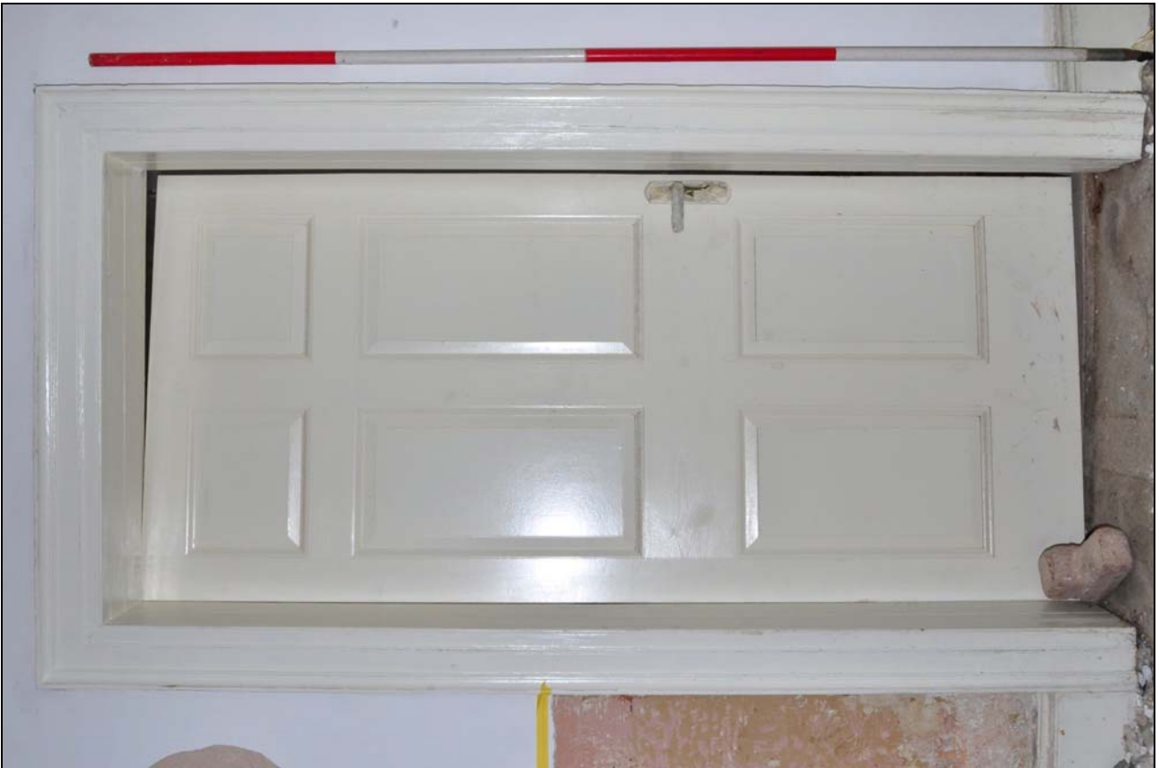
Photo 34: Ground floor: R1 (entrance hall), looking east towards modern door to R3 (historic architrave)
