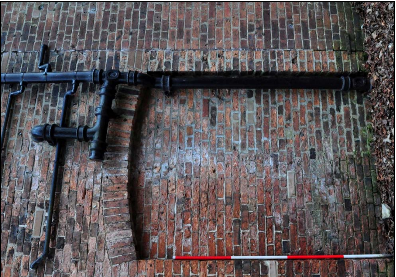
Photo 30: Blocked, arched opening in north end of rear range, with straight joint to right
