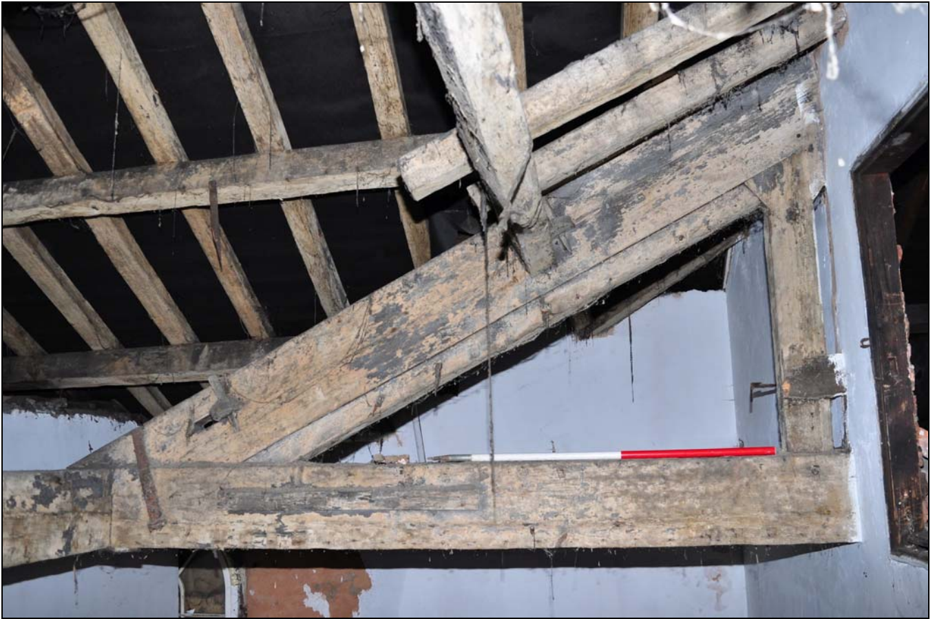
Photo 131: Second floor: R46, detail of part of exposed truss over, looking east
