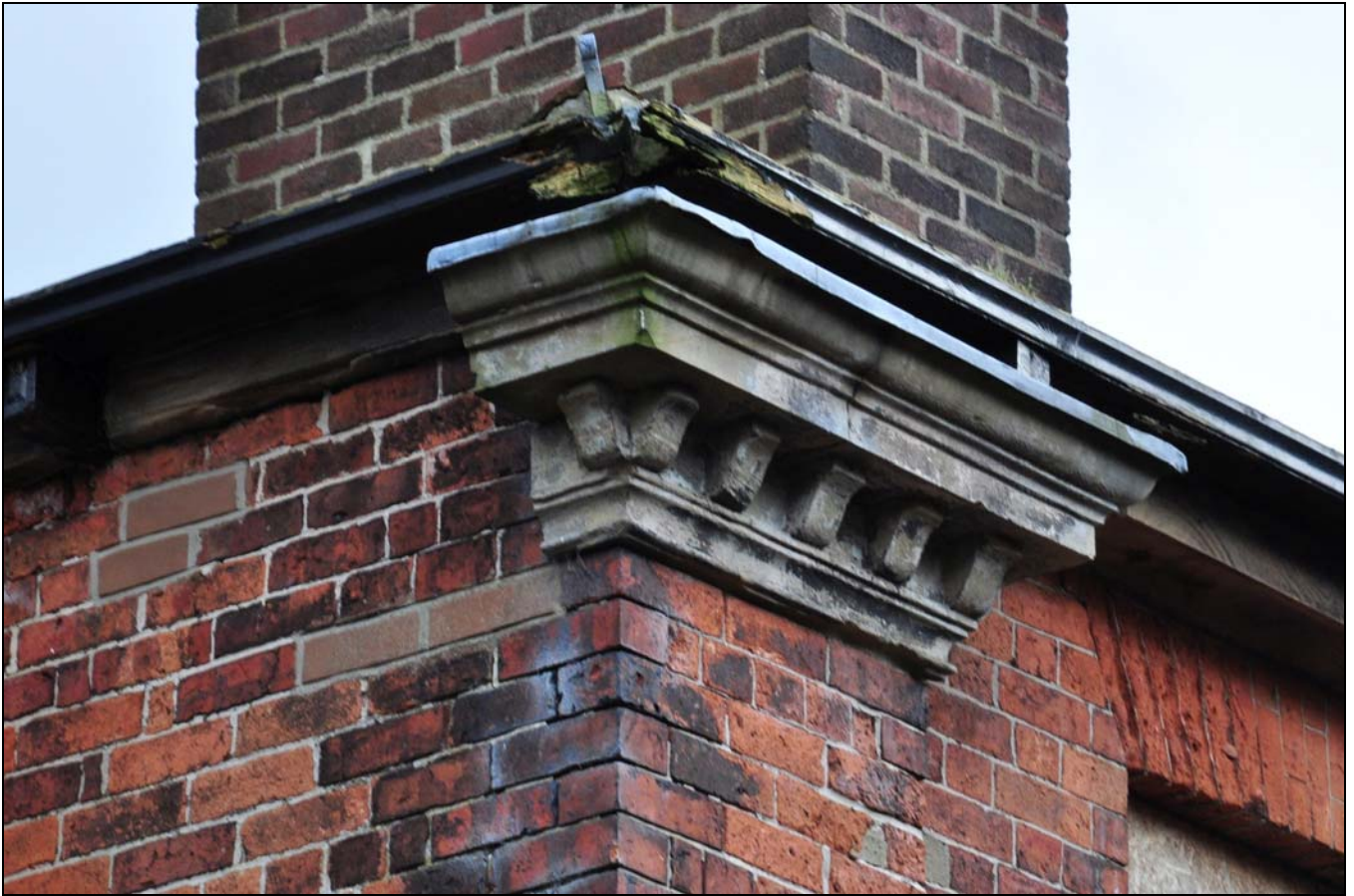
Photo 25: Detail of isolated section of eaves cornice, at north-west corner of rear range
