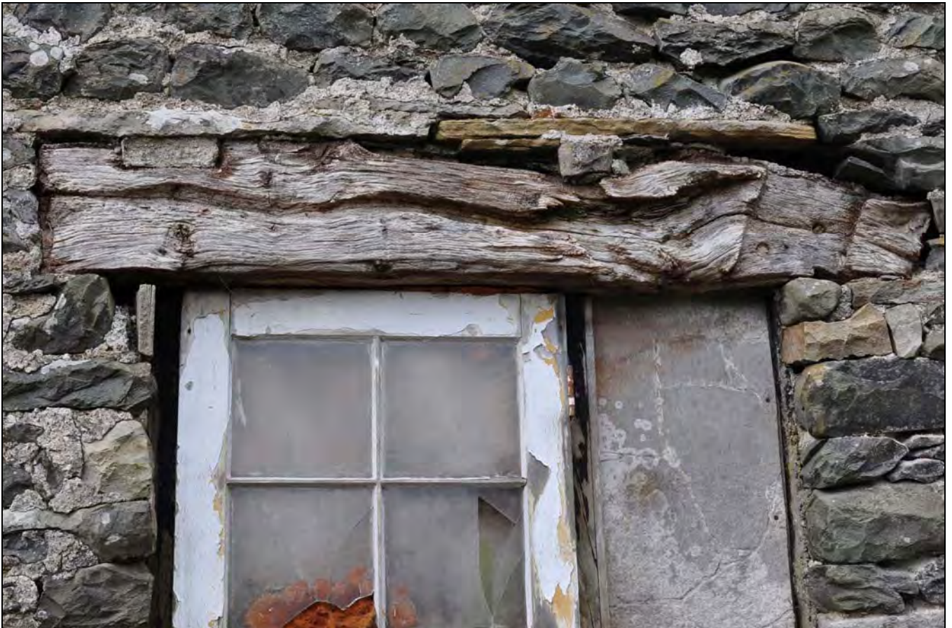
Photo 18: Detail of lintel, east side of added bay at north end of main range
