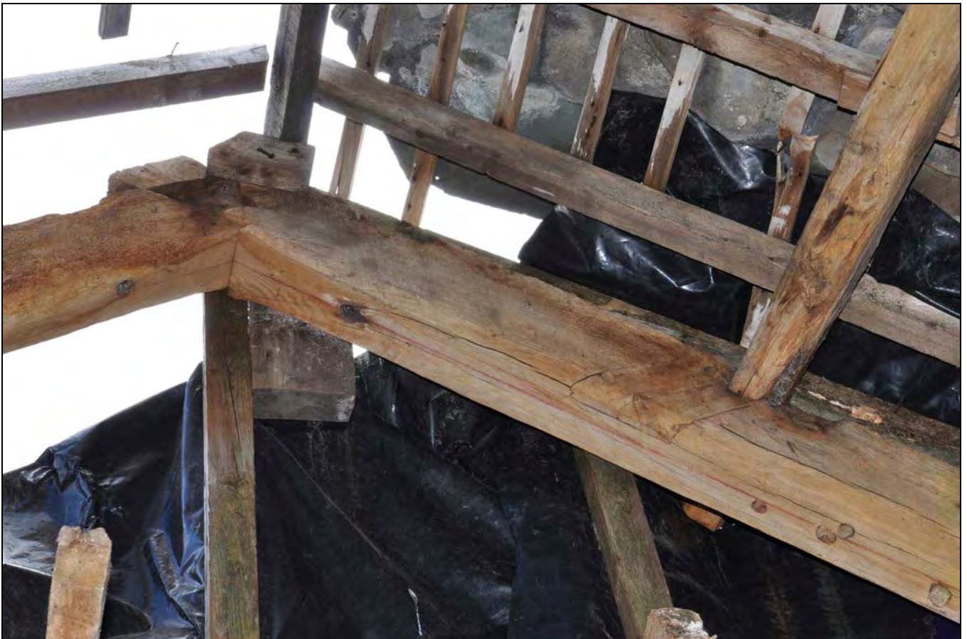
Photo 34: Detail of infilled halvings, pegs and chalk to roof truss over threshing bay, from the north
