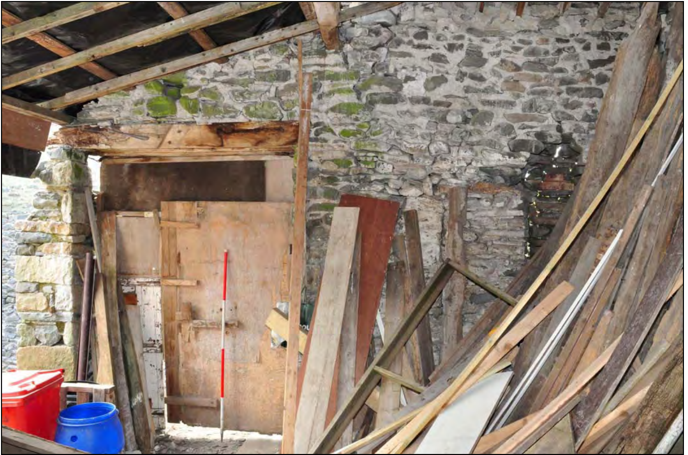
Photo 29: Threshing bay and mewstead, from the east (note blocked window at right)
