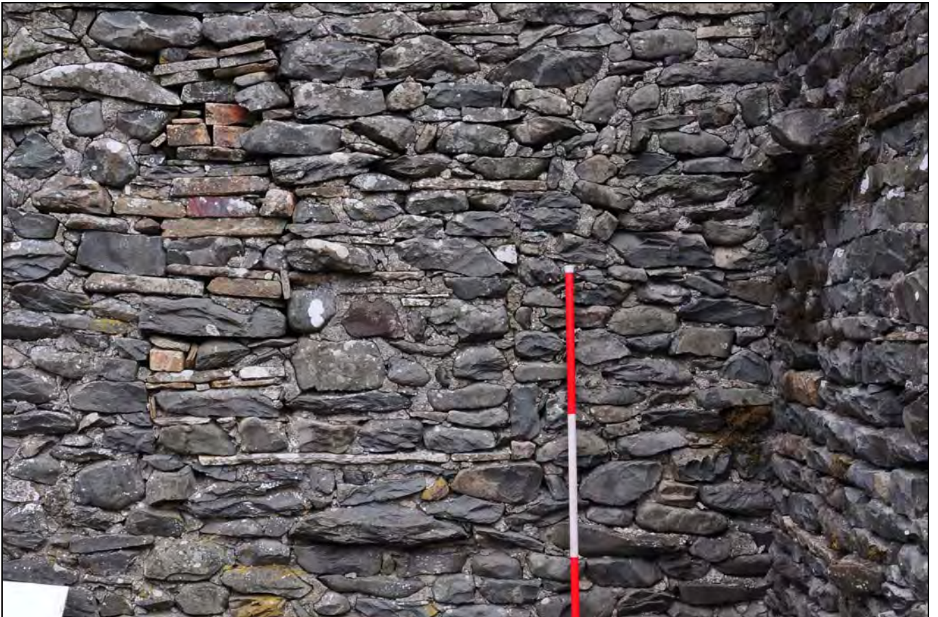
Photo 6: Blocked window to north of porch
