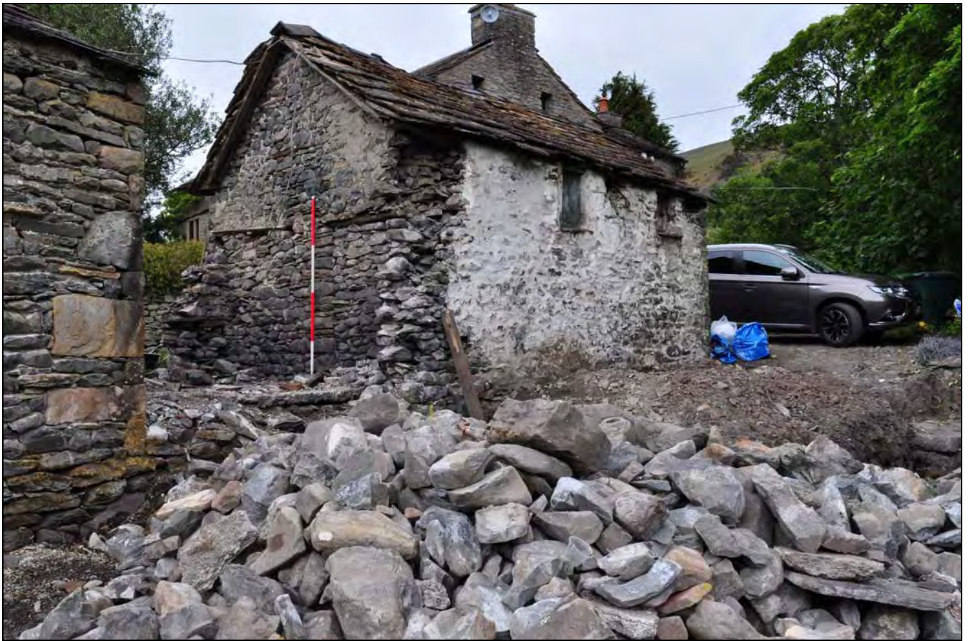
Photo 61: Garage, from the south-east, with site of collapsed lean-to in foreground
