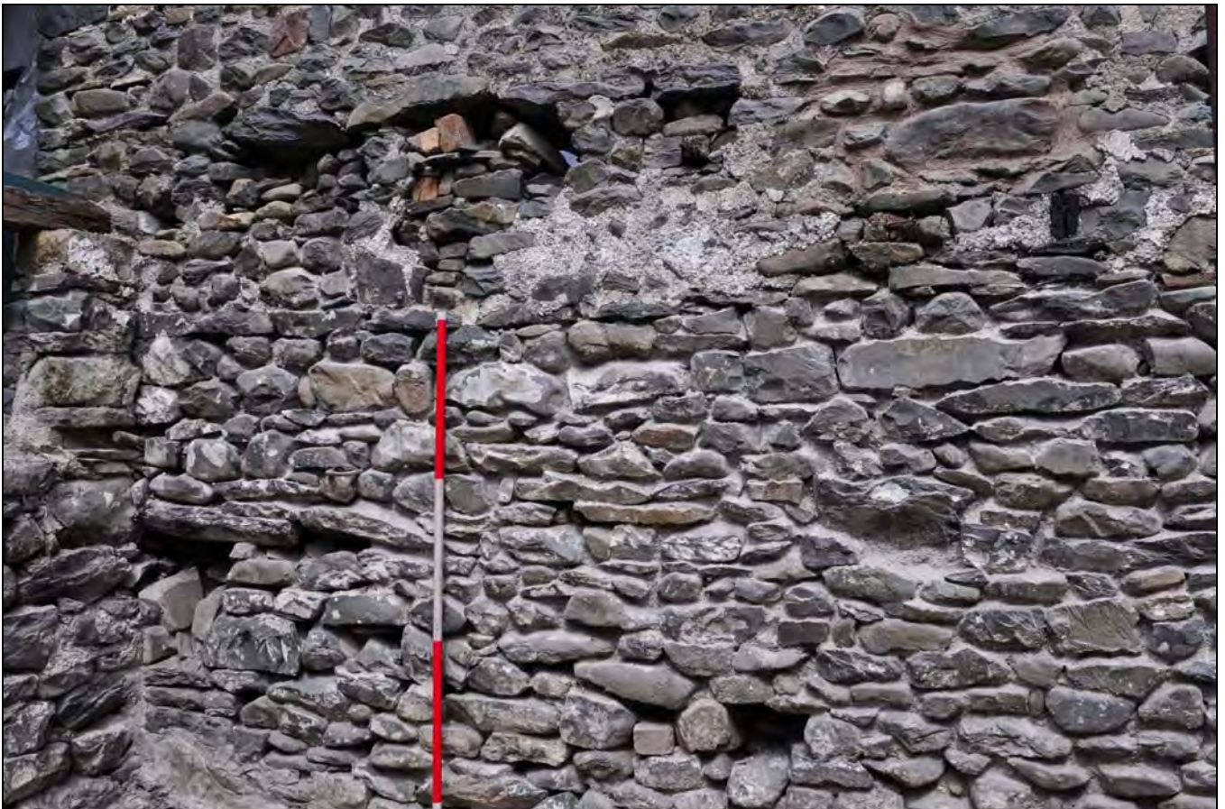
Photo 48: North-east corner of south wing, from the south-west; note two rows of loft timbers
