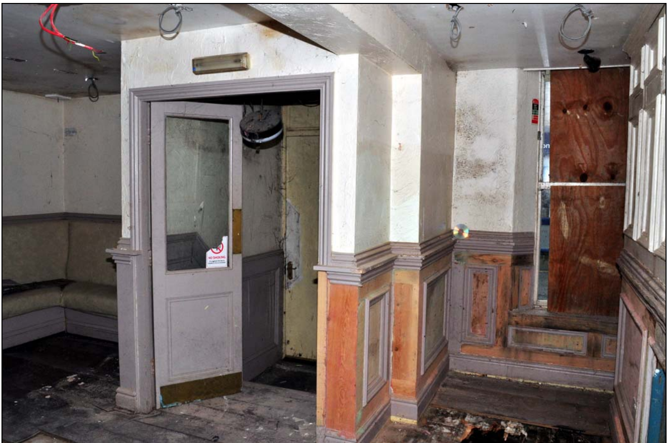
Photo 40: Basement: lobby to Dutton Street entrance, with altered floor levels, looking east
