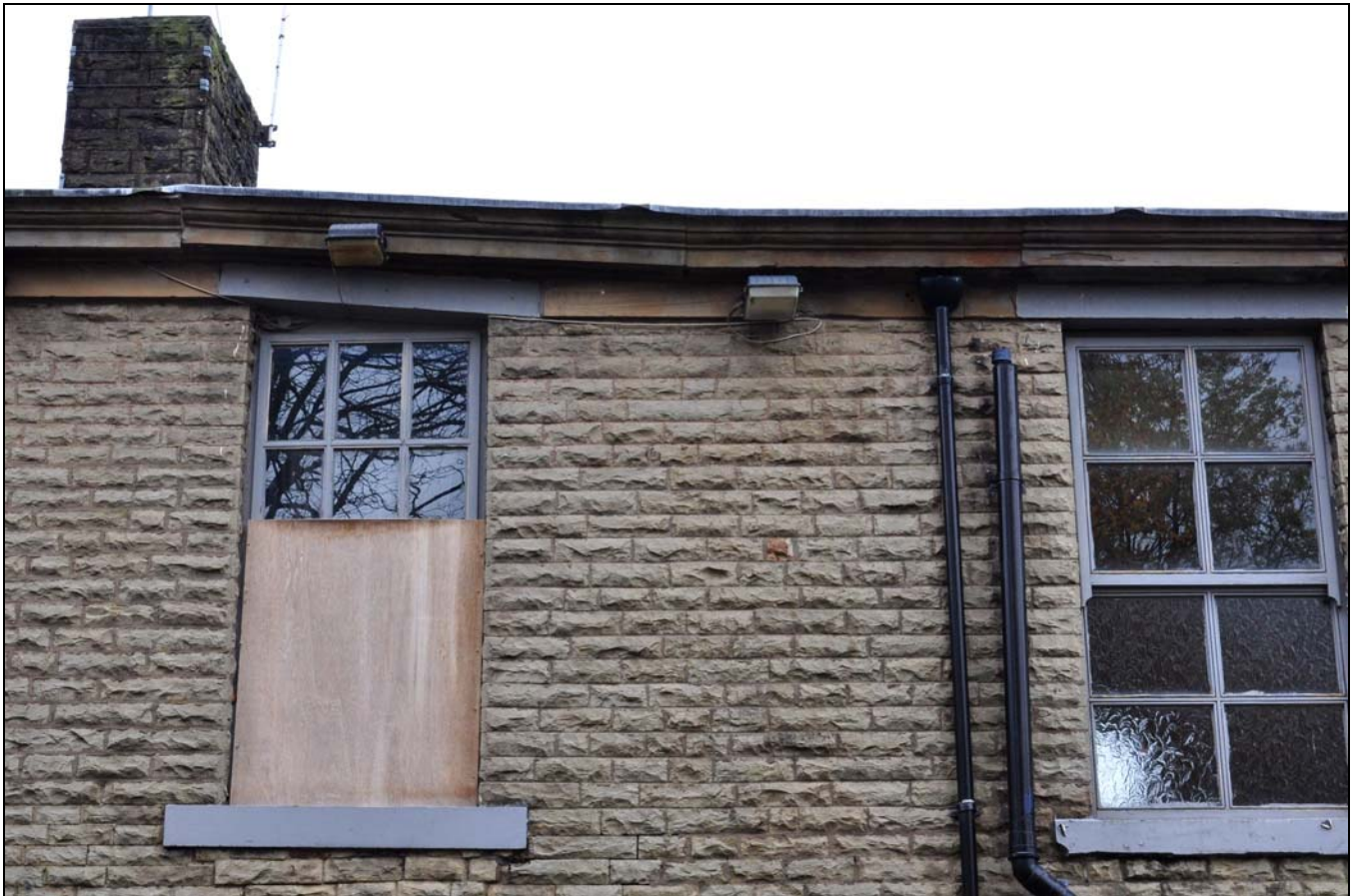
Photo 17: Inconsistent stonework at eaves, Holme Street elevation
