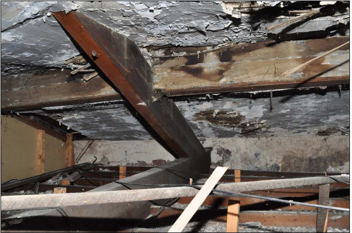
Photo 47: First floor: void over later ceilings, in former Club Room
