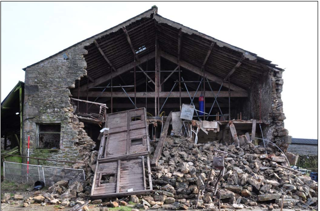
Photo 25: Barn 2: west gable (recently collapsed)
