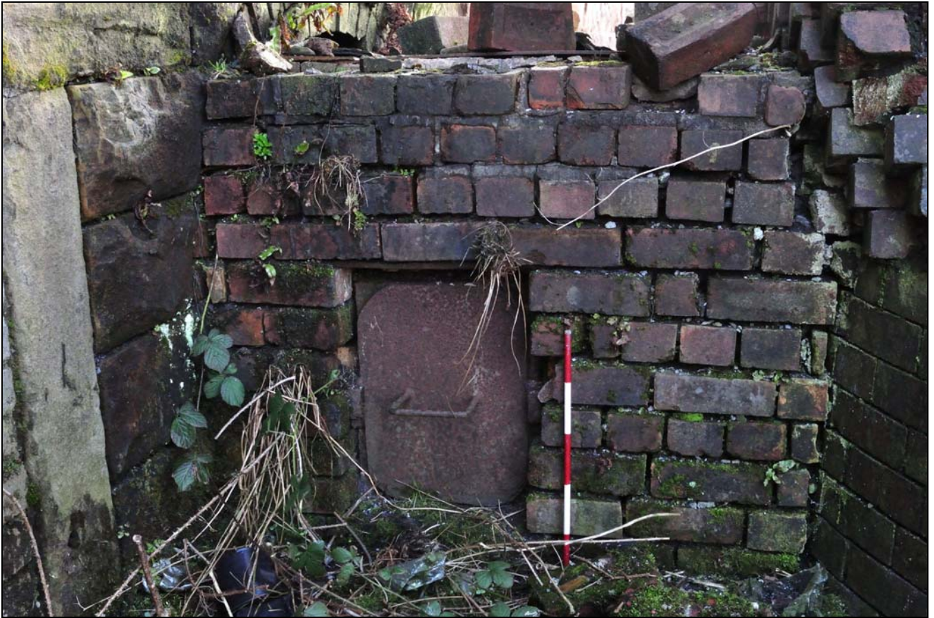
Photo 18: Shutter in north side of flue
