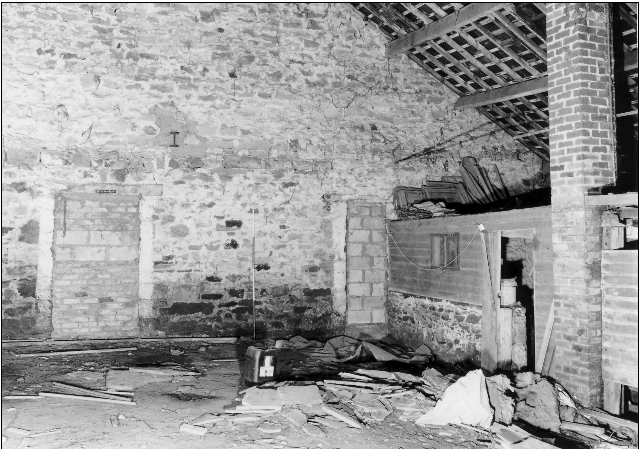
Photo 18: Interior of barn from the north-west, showing blocked doorways in original gable
