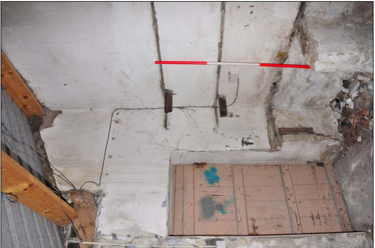
Photo 109: Building 7: lean-to at rear, east room (pantry), with door to house and traces of shelves
