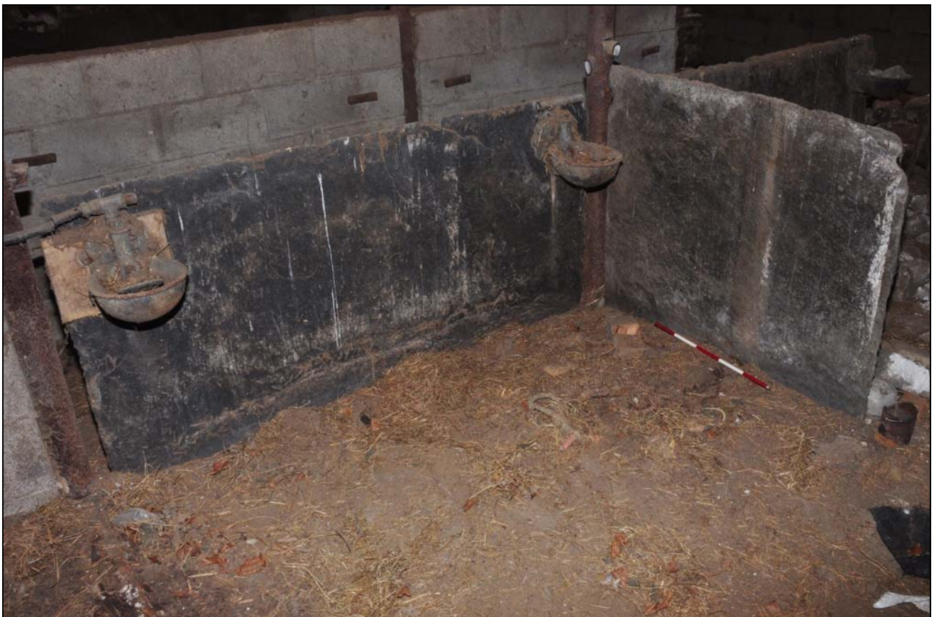
Photo 60: Building 4: remains of slate uprights in shippon, with modern steel columns, looking west
