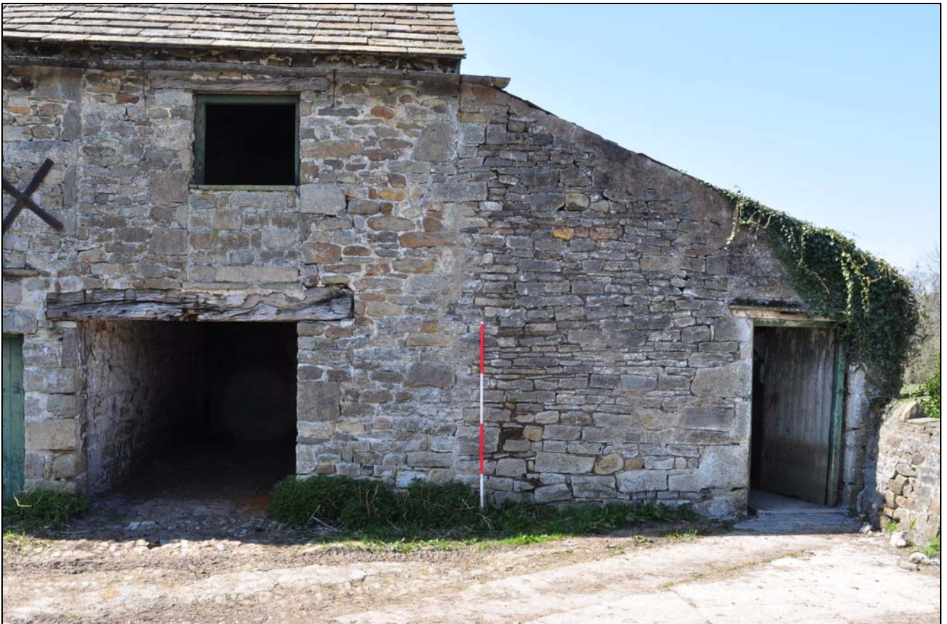
Photo 41: Front of added cart-shed and later lean-to at north end of barn, looking west
