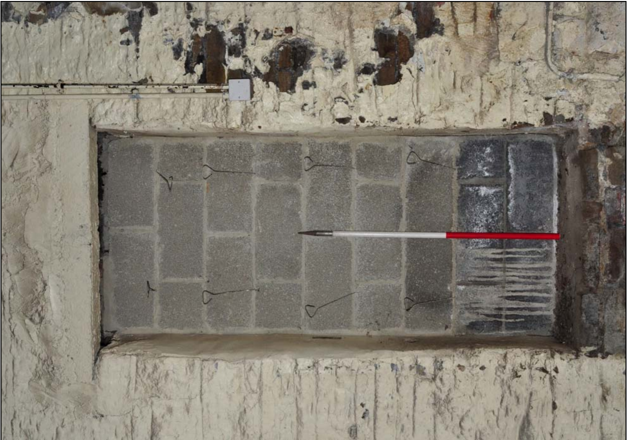
Photo 40: Blocked upper level doorway, north-east side of boiler house, from the south-west
