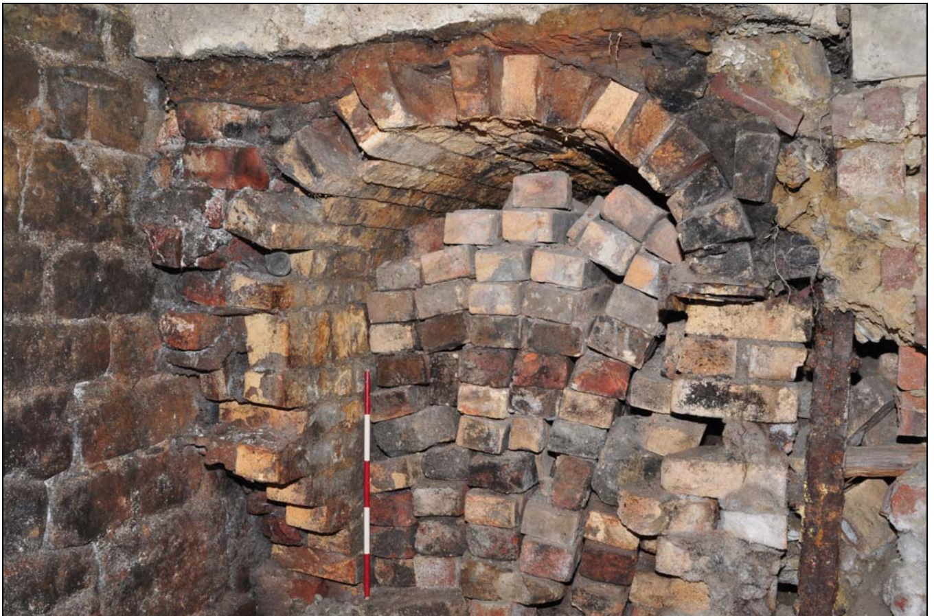
Photo 30: Remains of flue in south-east end of boiler house, from the north
