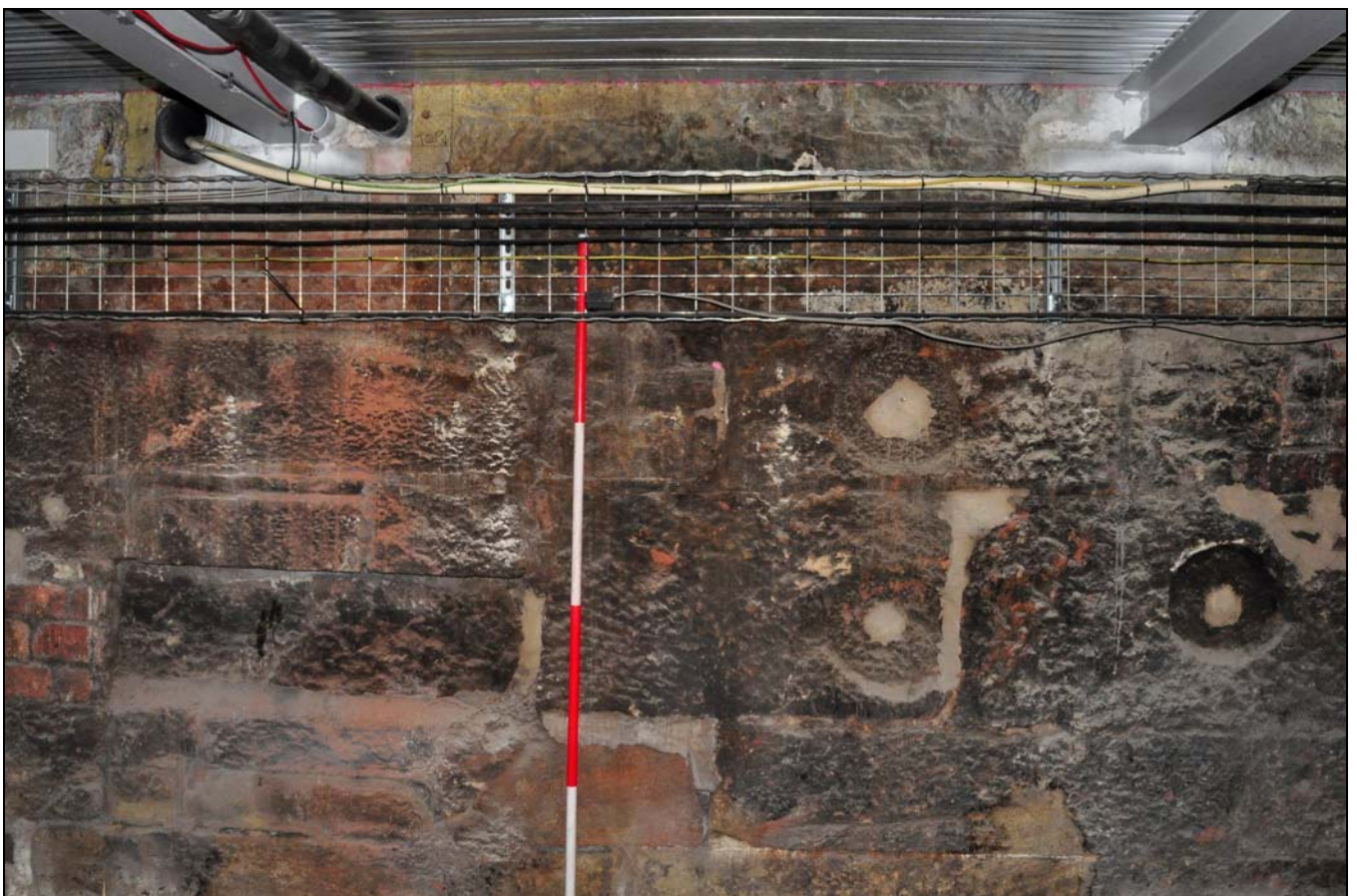
Photo 48: Large bearing box (slighted by modern upper floor), over massive blocks of stone, with bolting holes to right, north corner of engine house, from the south-west
