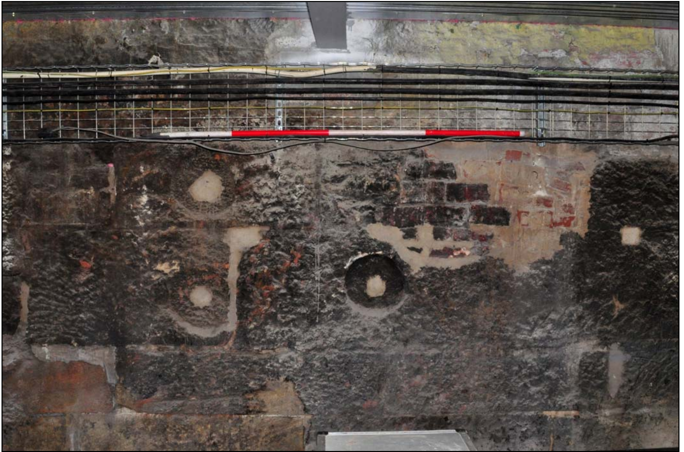
Photo 49: Bolting holes in stone blocks, north corner of engine house, from the south-west
