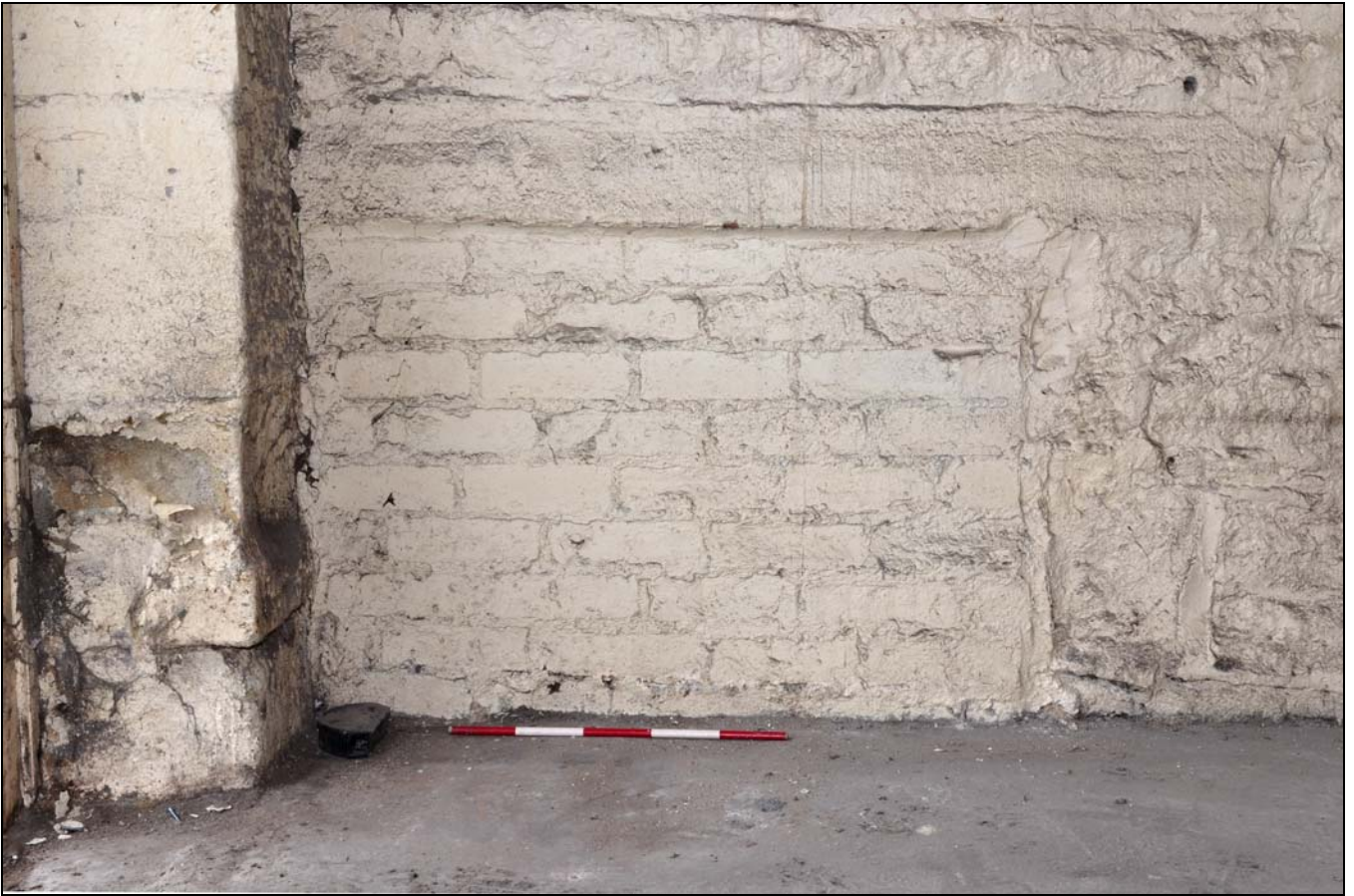
Photo 41: Blocked low opening, north-east side of boiler house, from the south-west
