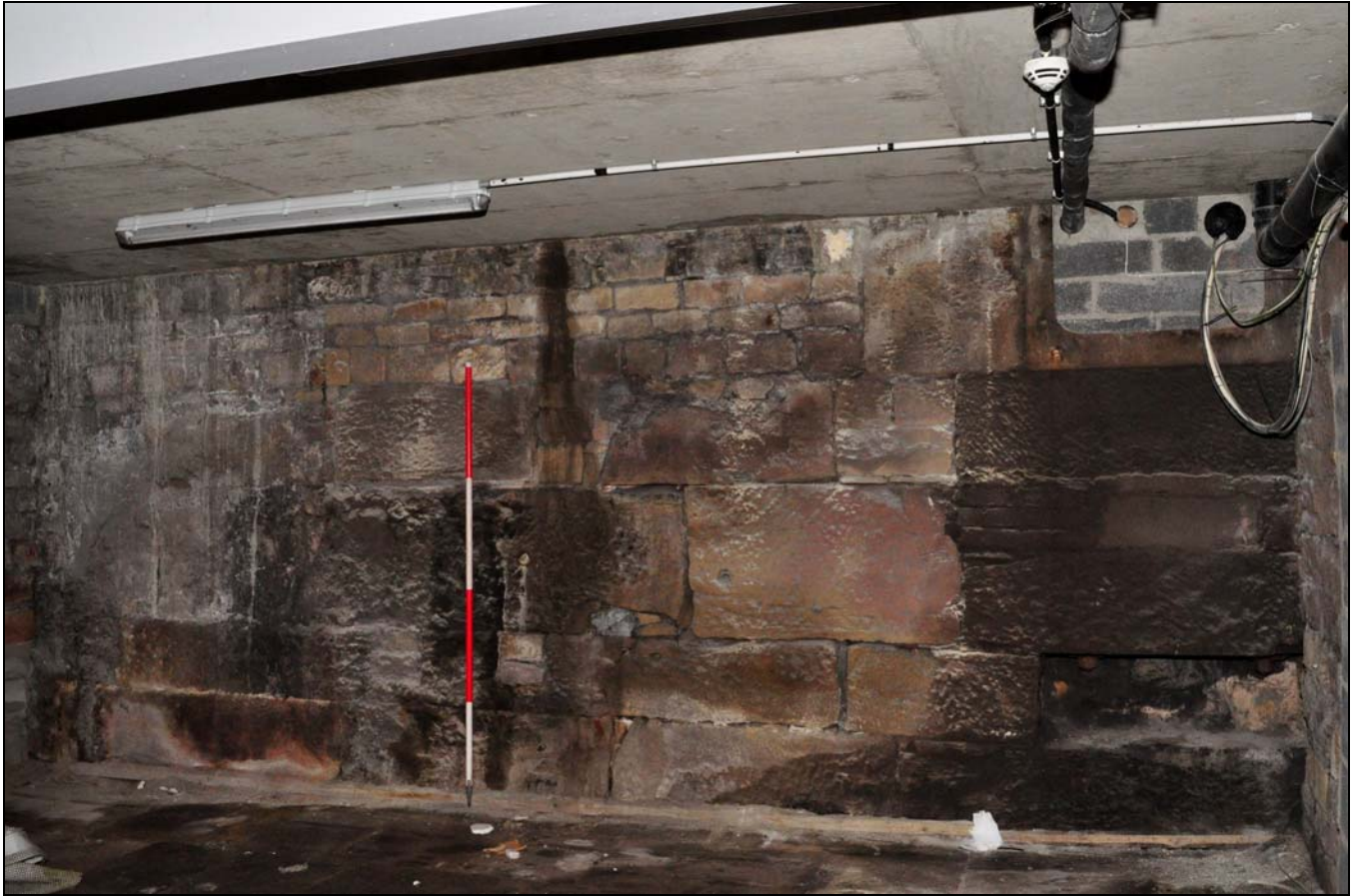
Photo 51: Massive stone blocks in wall with engine house, within main mill, from the north. Bearing box at right
