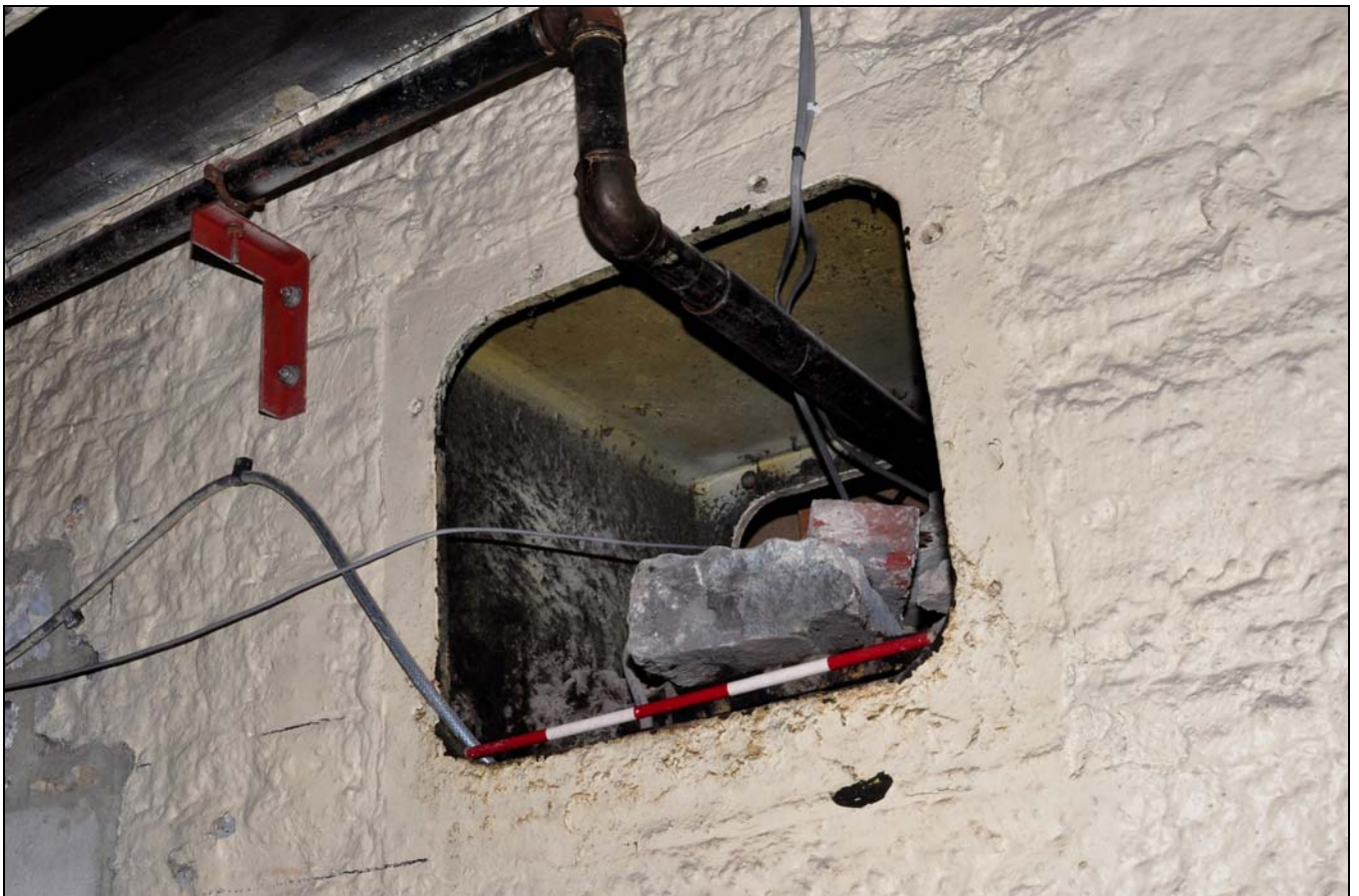
Photo 72: Bearing box for horizontal shaft into mill, in roof space over engine house, from the south
