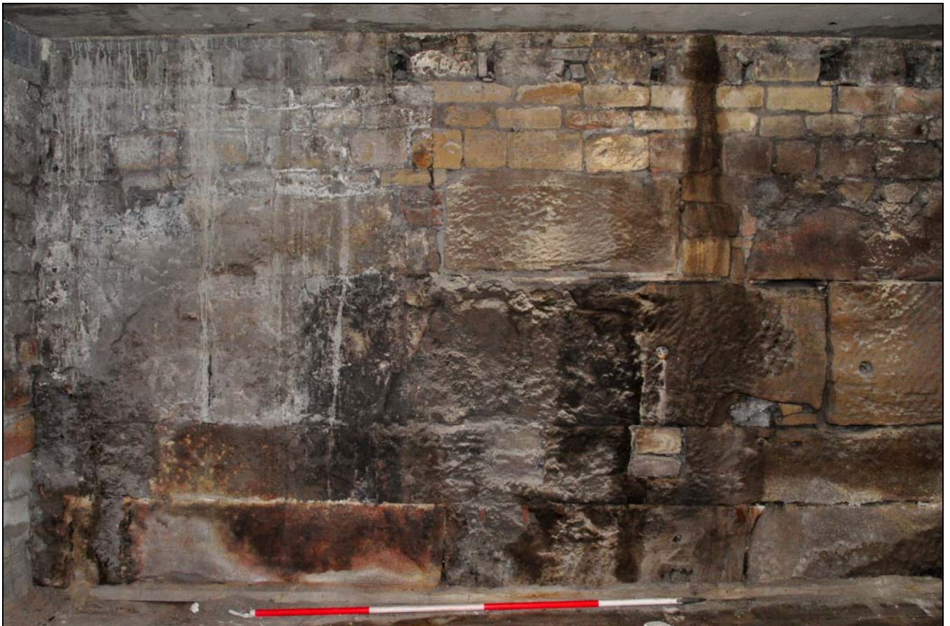
Photo 52: Massive stone blocks in wall with engine house, within main mill, from the north-east
