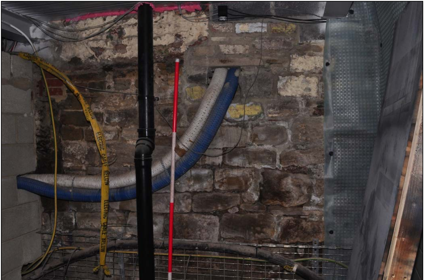
Photo 57: Ground floor of engine house, north-east side (hidden by electrical equipment), from the south-west
