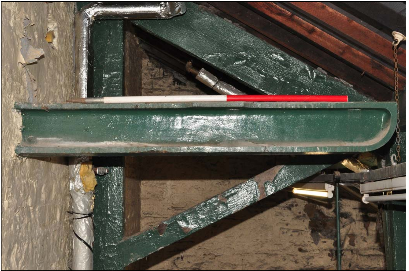
Photo 69: Cantilevered iron beam in roof space over engine house, from the north-west
