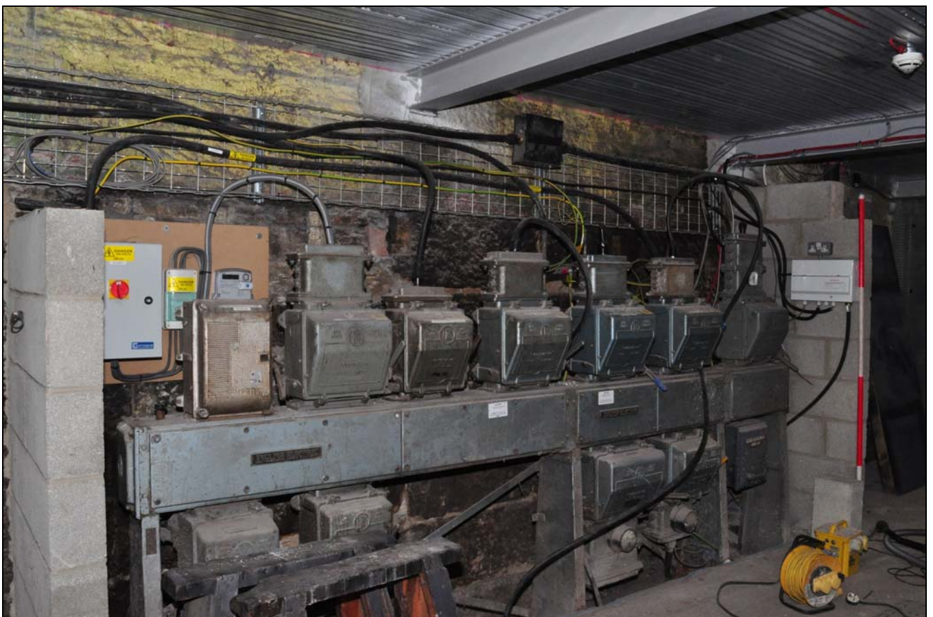
Photo 56: Ground floor of engine house, north-east side (hidden by electrical equipment), from the west
