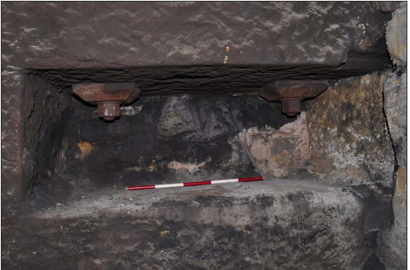
Photo 55: Vertical fastening bolts beneath large bearing box in wall with engine house, within main mill, from the north-east
