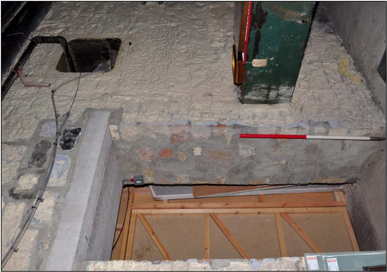
Photo 71: Inserted doorway to mill, and bearing box for horizontal shaft, in roof space over engine house, from the west
