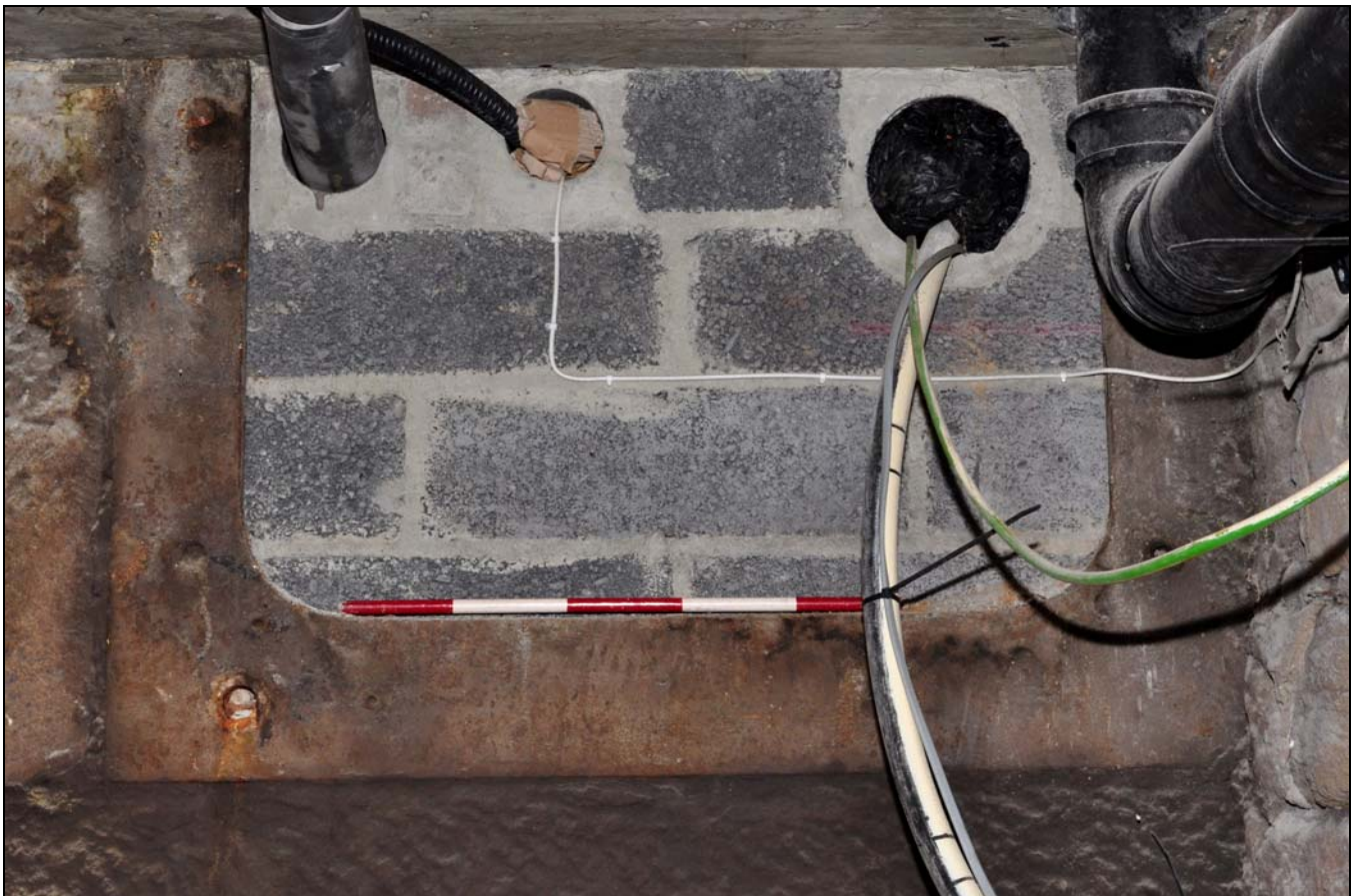
Photo 54: Large bearing box in wall with engine house, within main mill, from the north-east
