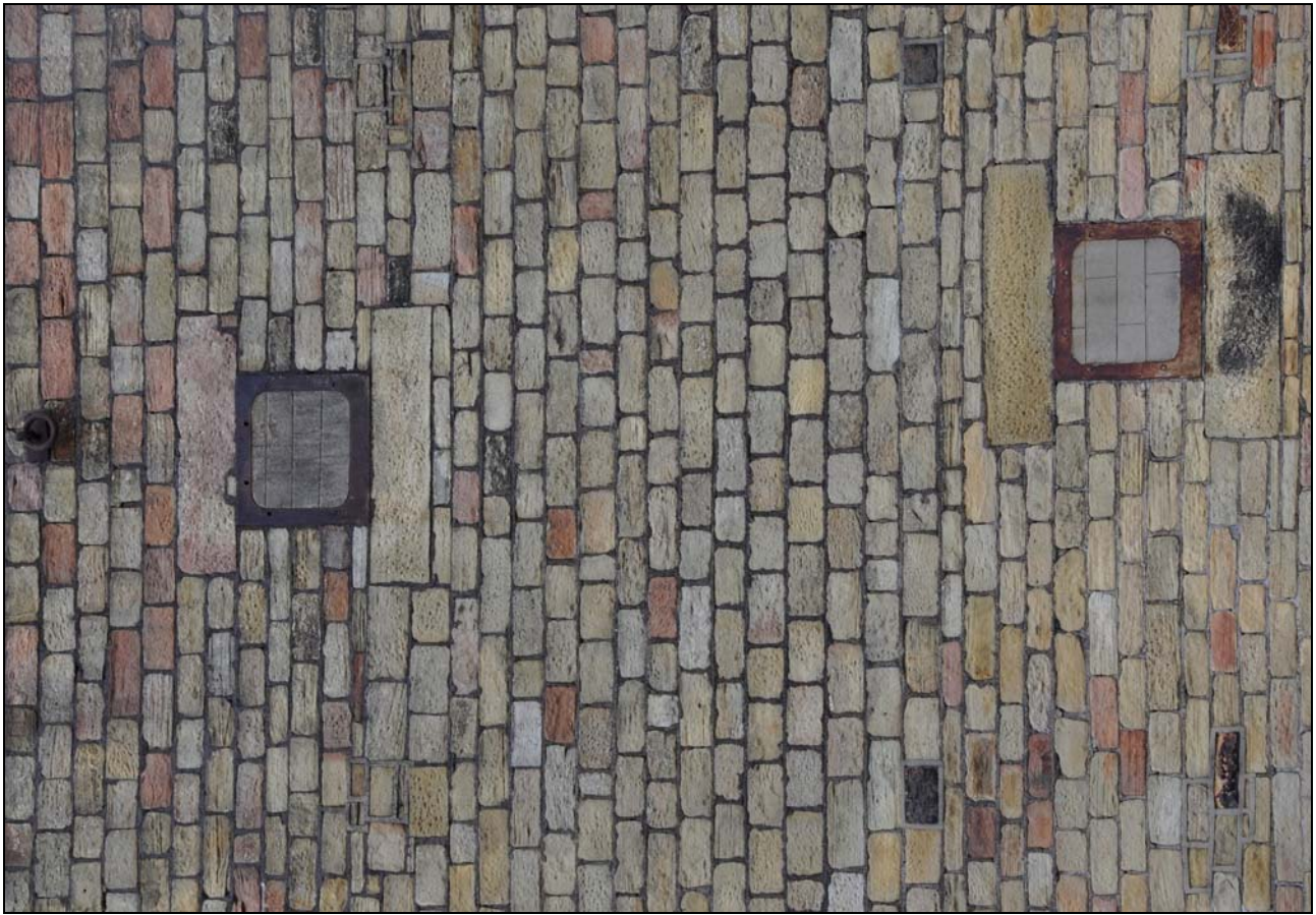
Photo 23: Bearings for shafts from rope race, in end wall of mill, from the south-west
