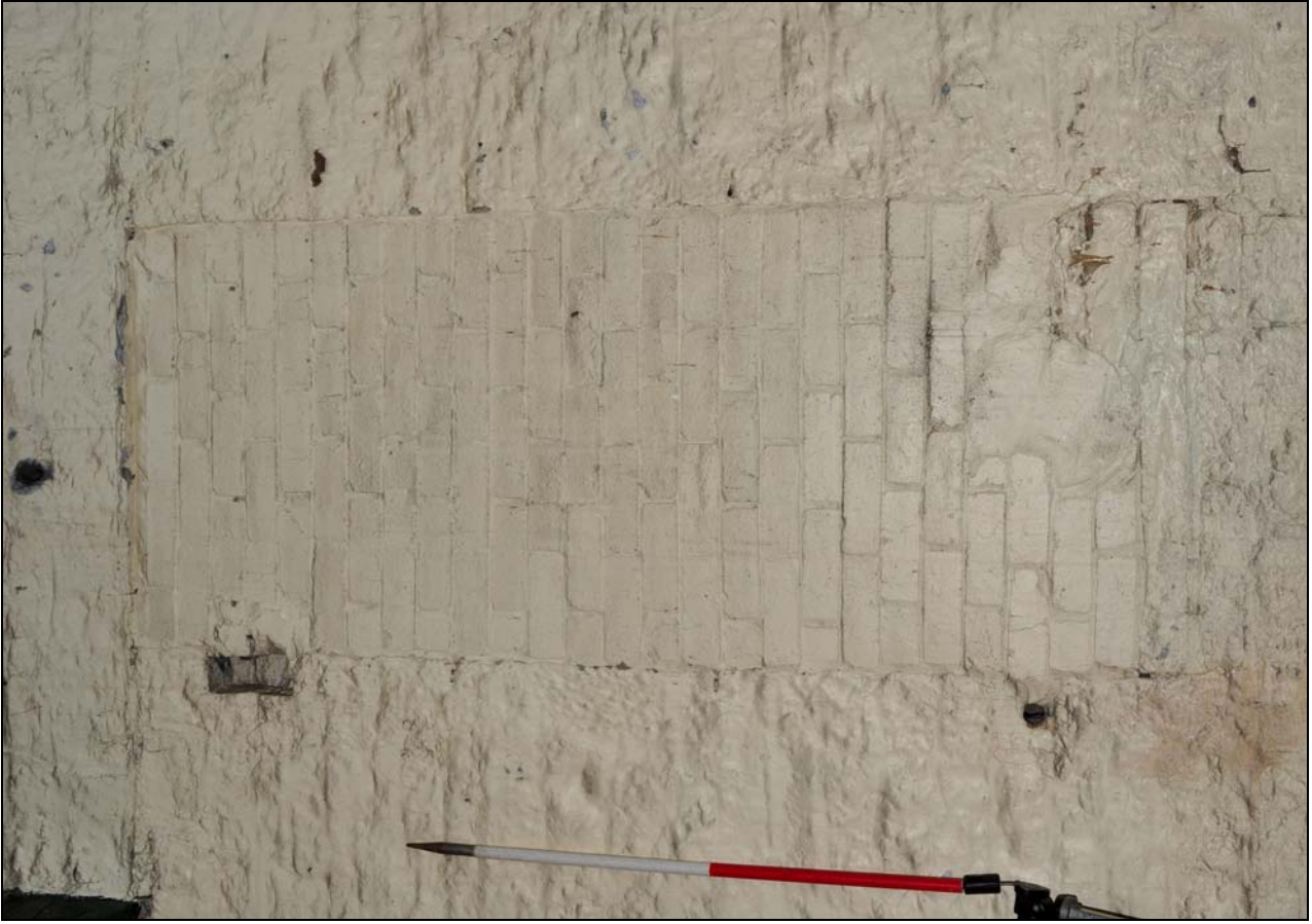
Photo 39: Blocked upper level doorway, north-east side of boiler house, from the south-west
