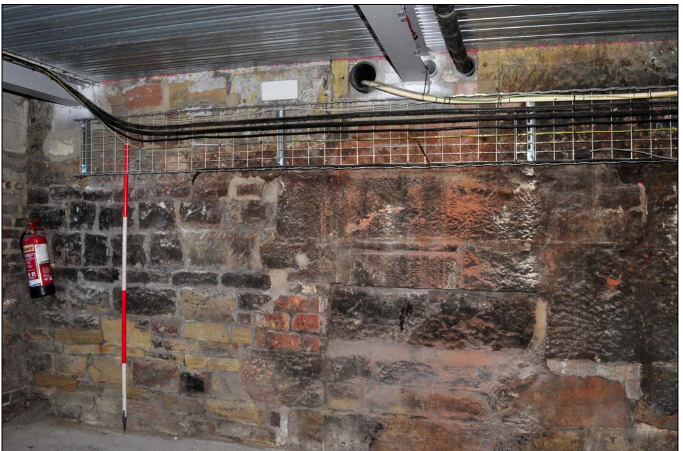
Photo 46: Large bearing box (slighted by modern upper floor), over massive blocks of stone, north corner of engine house, from the south
