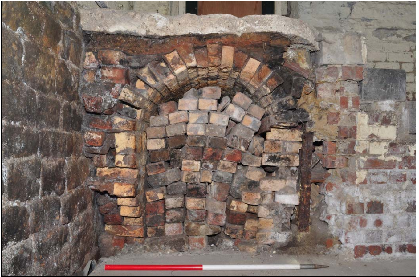
Photo 29: Remains of flue in south-east end of boiler house, from the north-east
