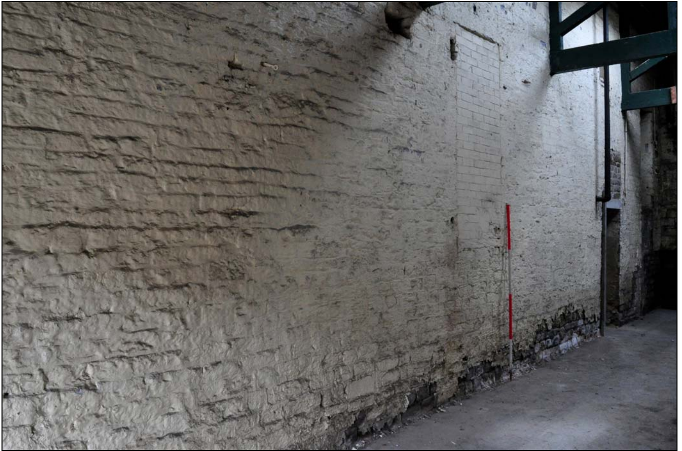
Photo 37: Interior of boiler house: north-east side, from the west
