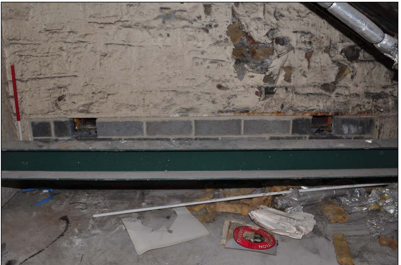
Photo 64: Window lintel in south-east side of engine house roof space, from the north-west
