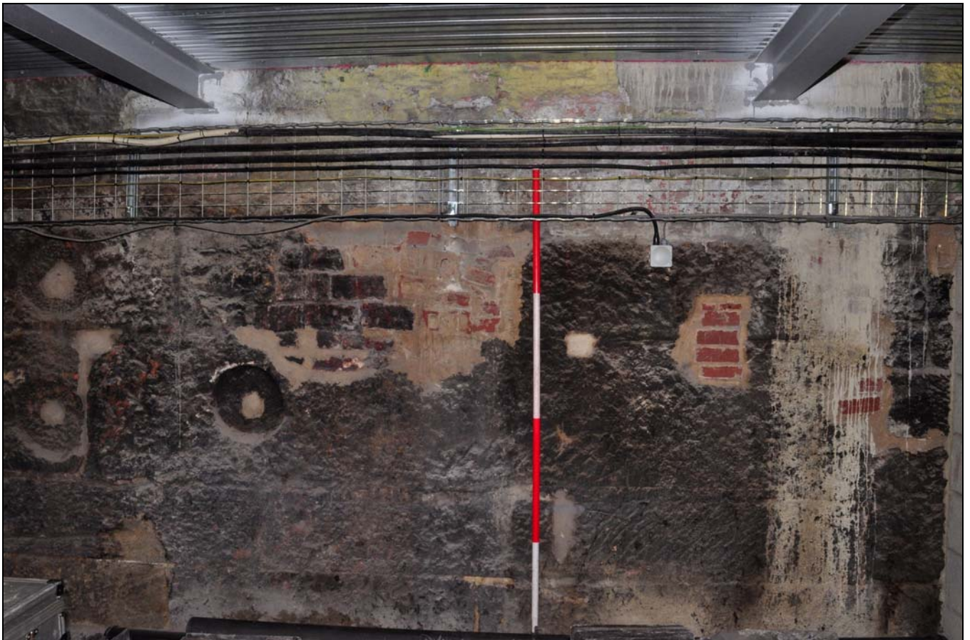
Photo 50: Bolting holes in stone blocks, north corner of engine house, from the south-west
