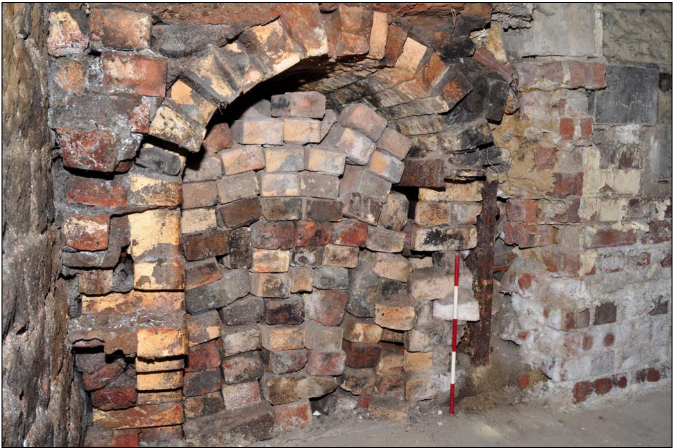
Photo 31: Remains of flue in south-east end of boiler house, from the east
