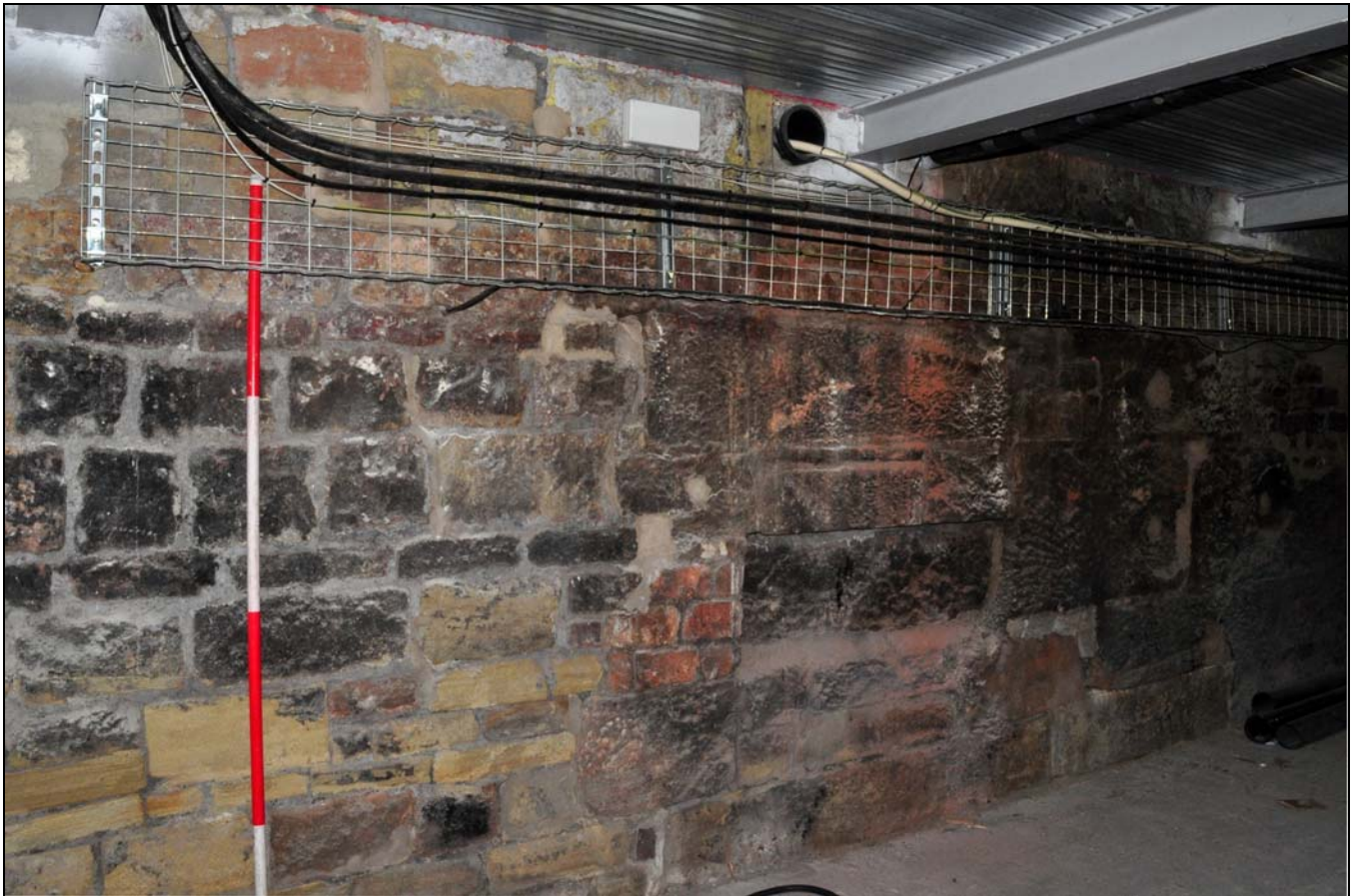
Photo 47: Large bearing box (slighted by modern upper floor), over massive blocks of stone, north corner of engine house, from the west
