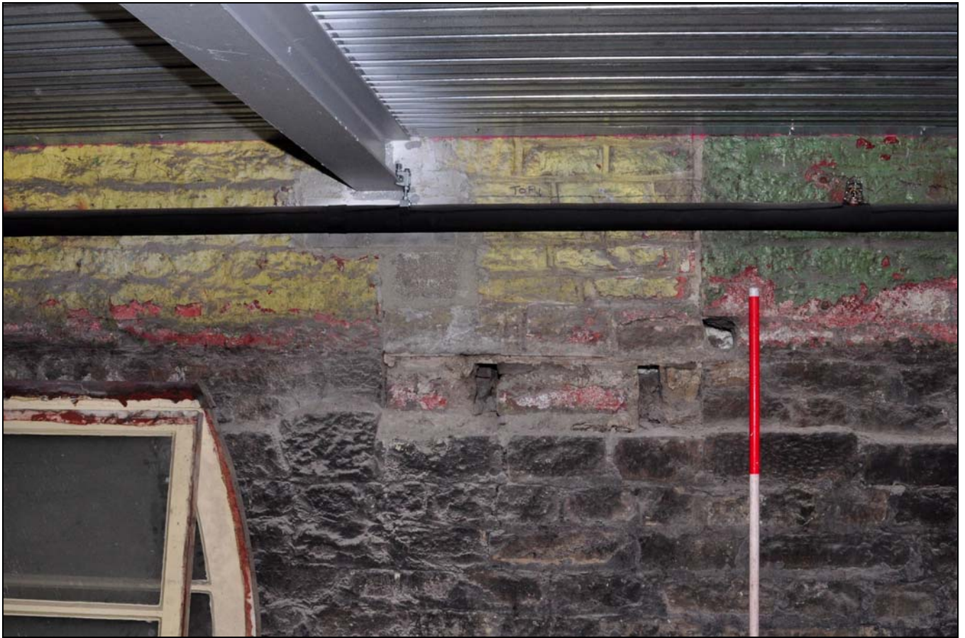
Photo 61: Base of blocked upper level doorway in south-west side of engine house, from the north-east
