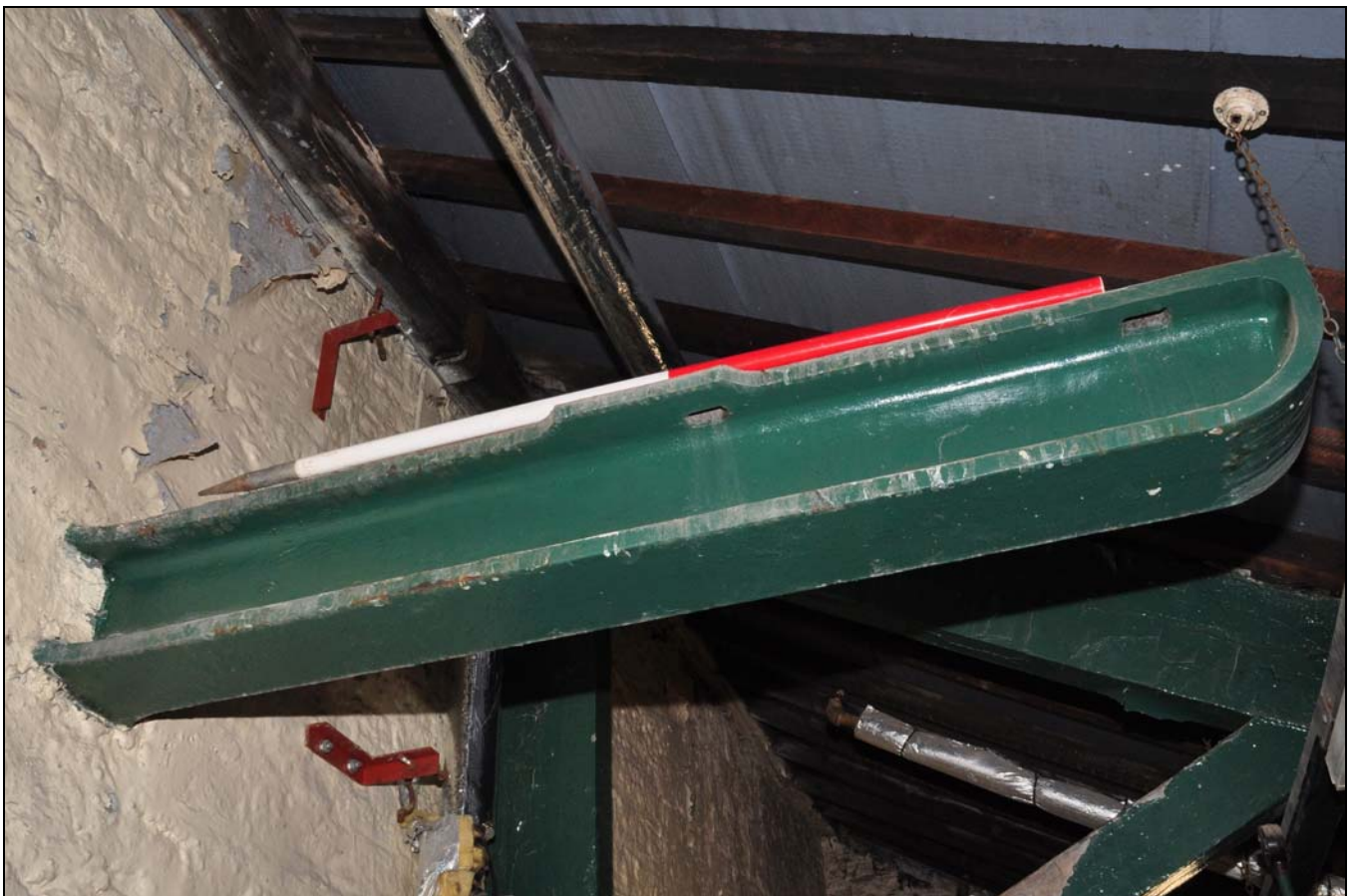
Photo 70: Cantilevered iron beam in roof space over engine house, from the west
