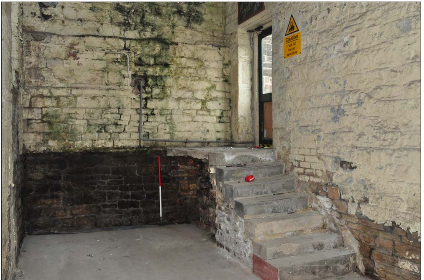
Photo 28: Remains of flue in south-east end of boiler house, with modern steps, from the north
