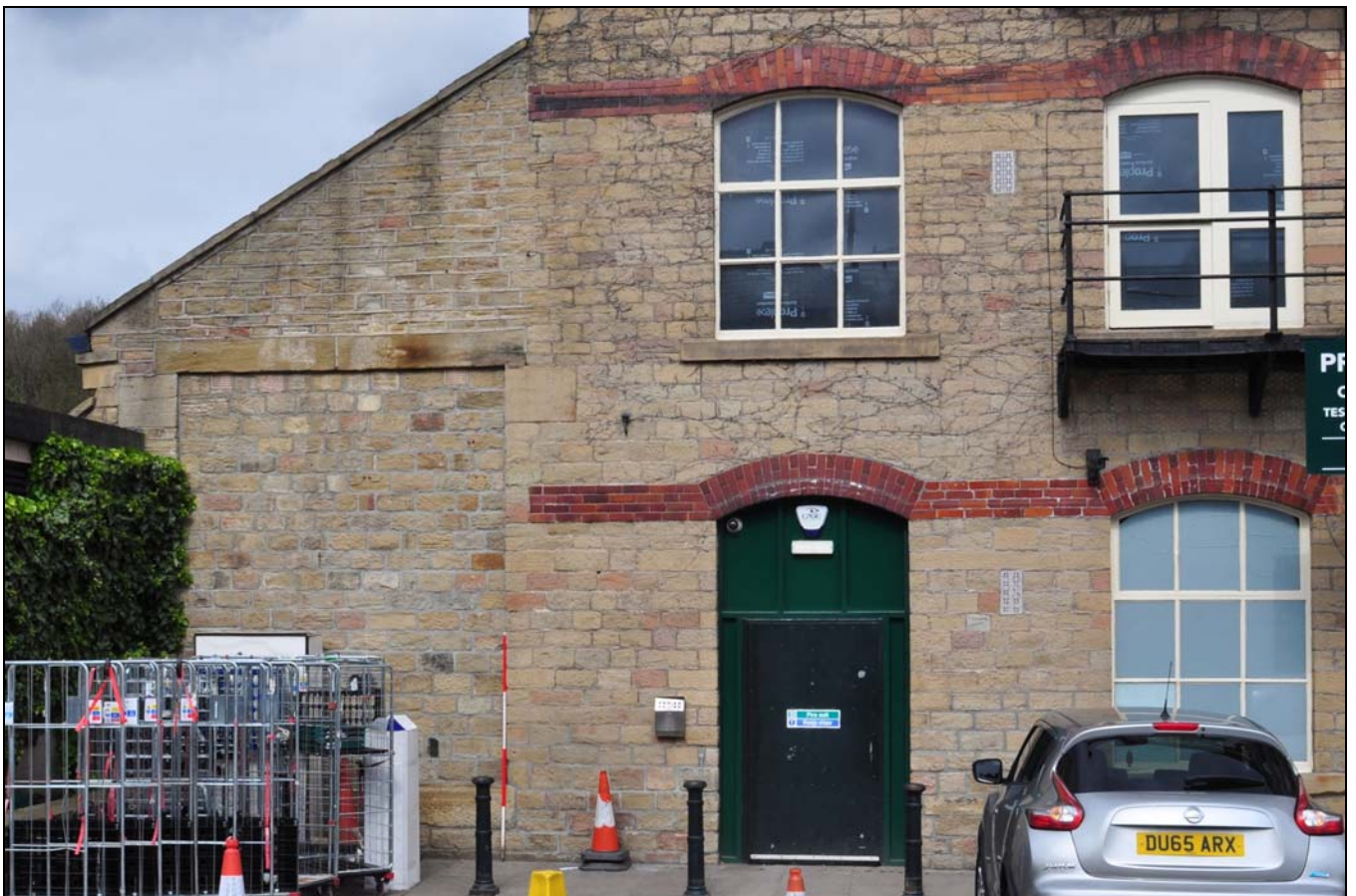
Photo 8: South-east side of engine house, with blocked window
