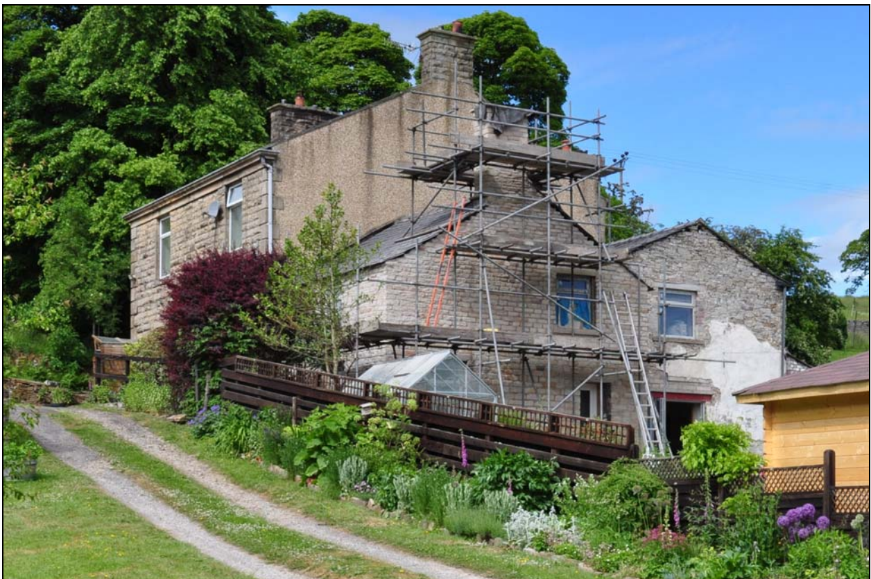
Photo 6: General view of Sweetclough Cottage (lower) and Farmhouse (upper), from the east
