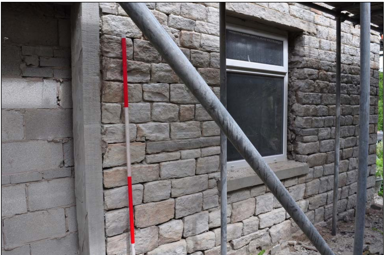
Photo 4: Ground floor window in front elevation, with earlier sill visible at higher level
