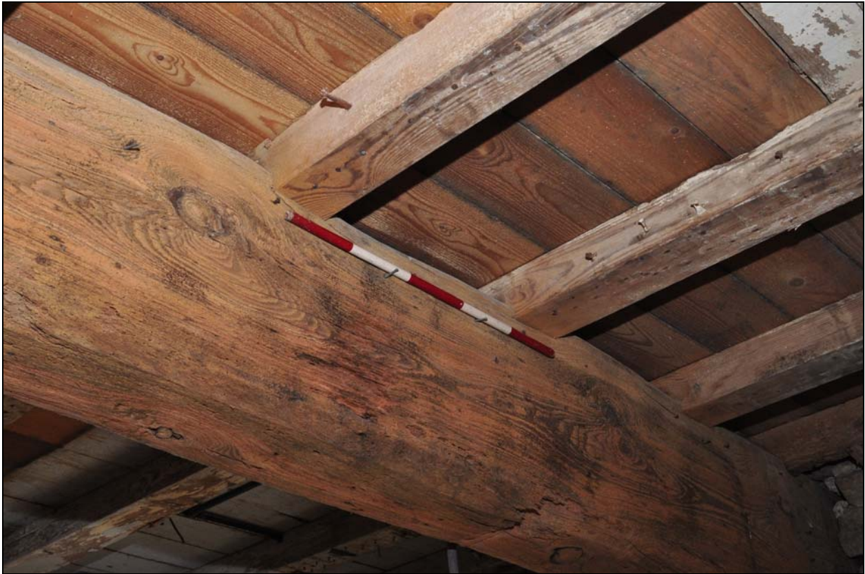
Photo 17: Ground floor room in front part of cottage: underside of first floor
