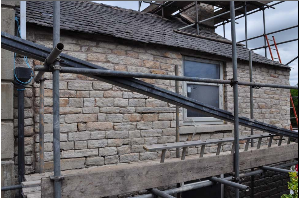
Photo 5: First floor in front elevation: straight joint at left, and earlier window sill visible
