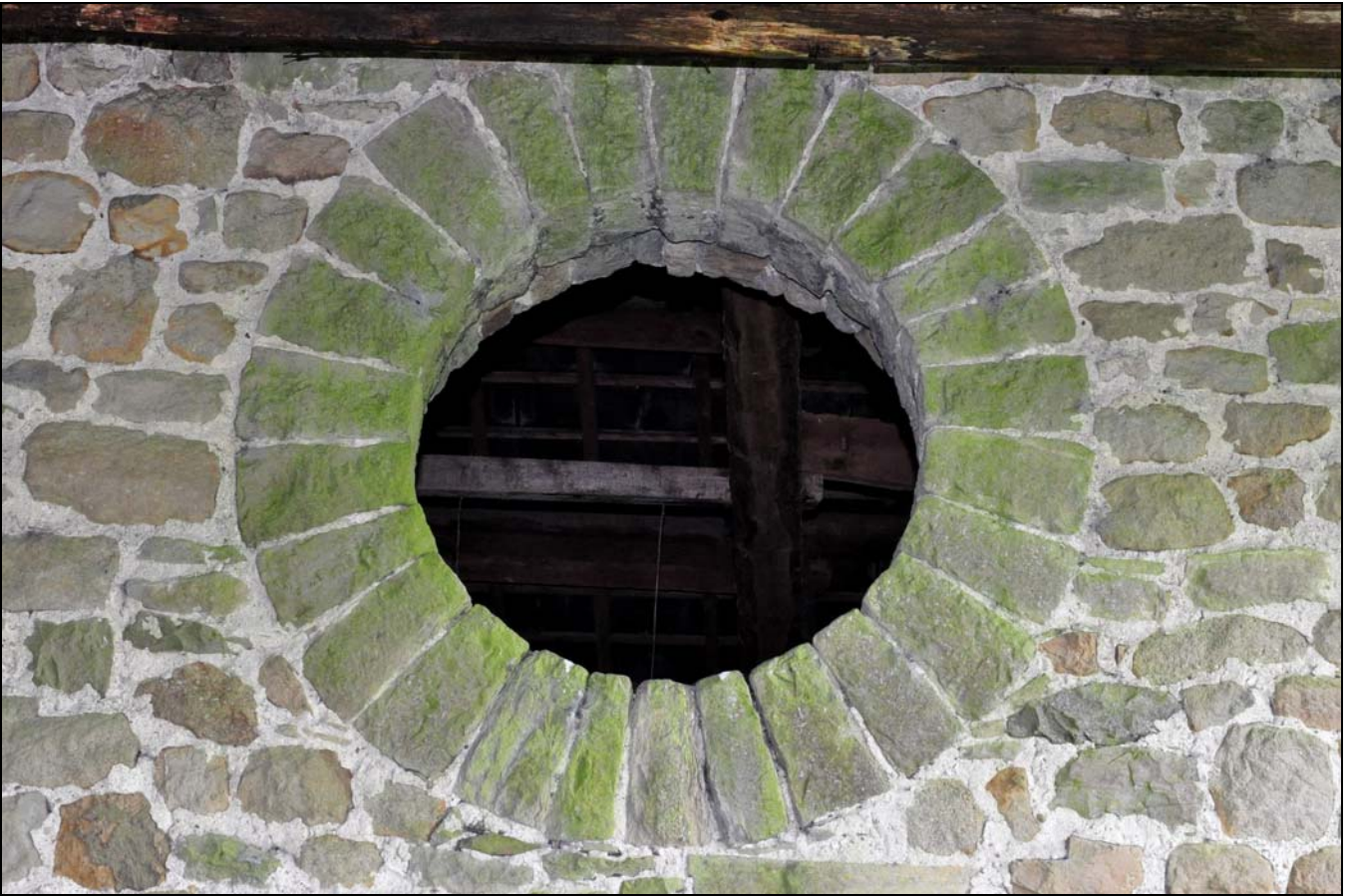
Photo 9: Detail of forking hole in front elevation (north)
