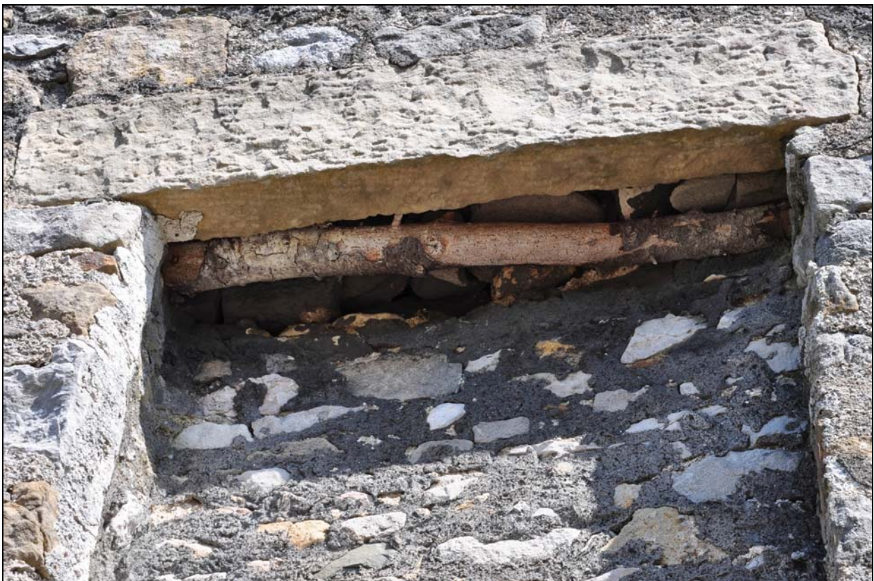
Photo 4: Detail of lintel to blind opening, upper part of south elevation, with timber to rubble core
