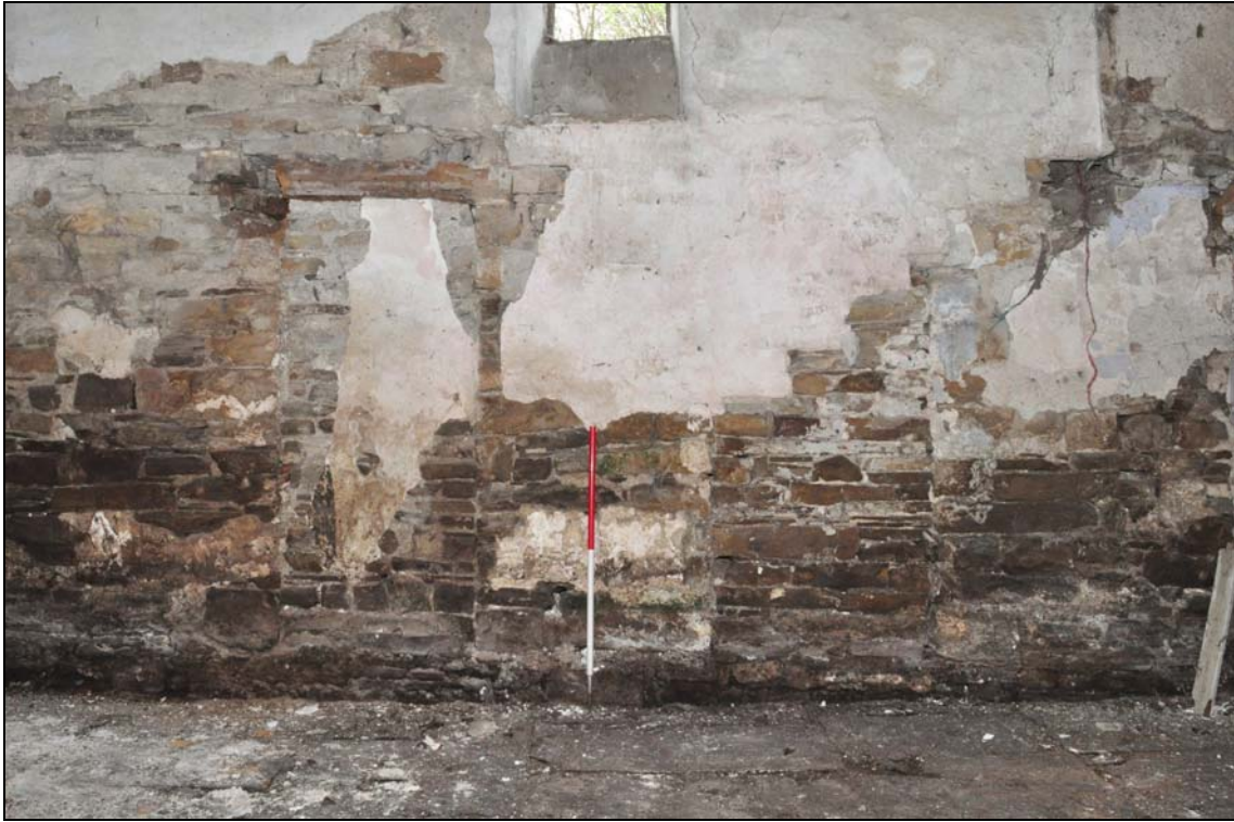
Photo 33: Farmhouse interior: housebody, looking south, towards blocked doorways to former stairs outshut
