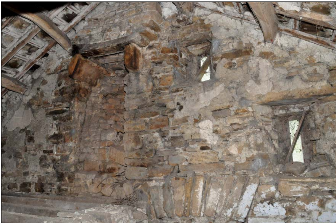
Photo 70: East part, interior: east gable at first floor level, showing site of smoke-hood
