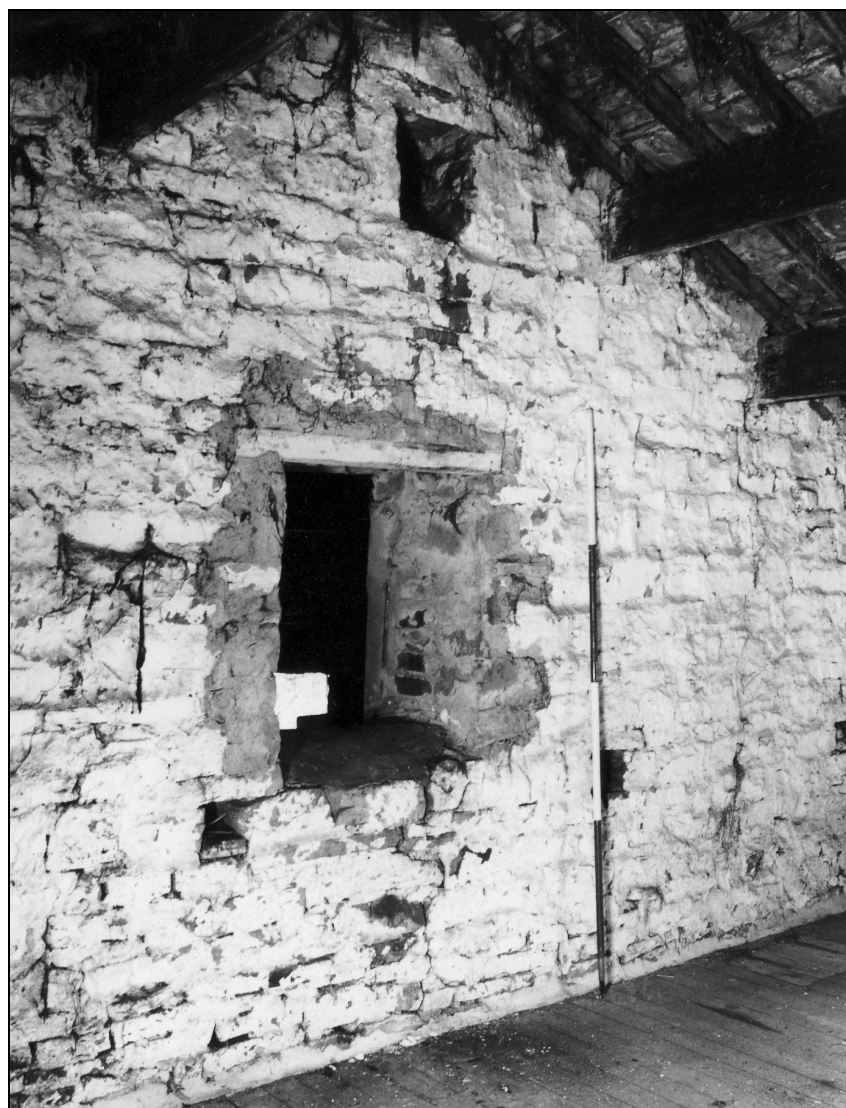
Photo 33: Inserted first floor opening, and earlier owl hole, between lofts in stable and barn, from the west
