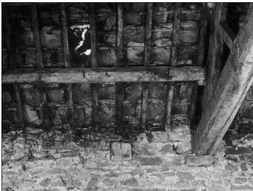
Photo 42: Redundant corbel in north side of mewstead
