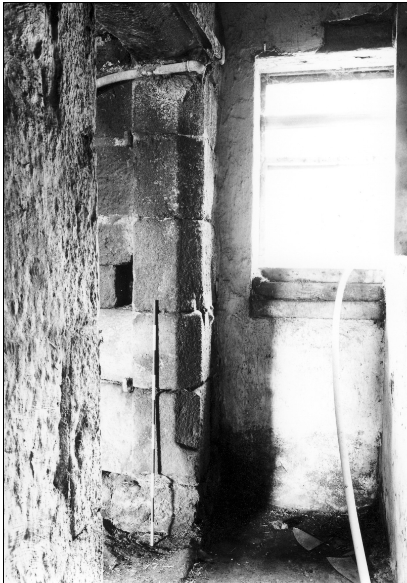
Photo 13: Detail of chamfer and stop to doorway at north end of east gable
