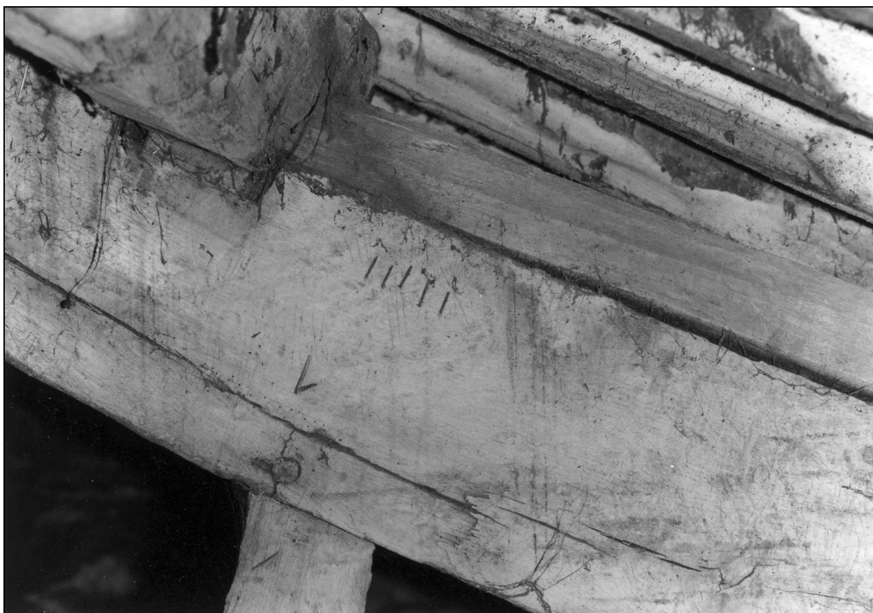
Photo 46: Upper face of west truss in barn: assembly marks to outer strut at north end
