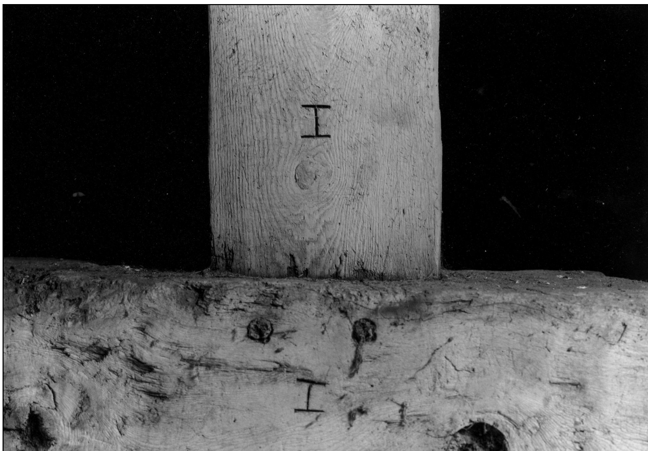
Photo 43: Upper face of west truss in barn: assembly marks to foot of king post
