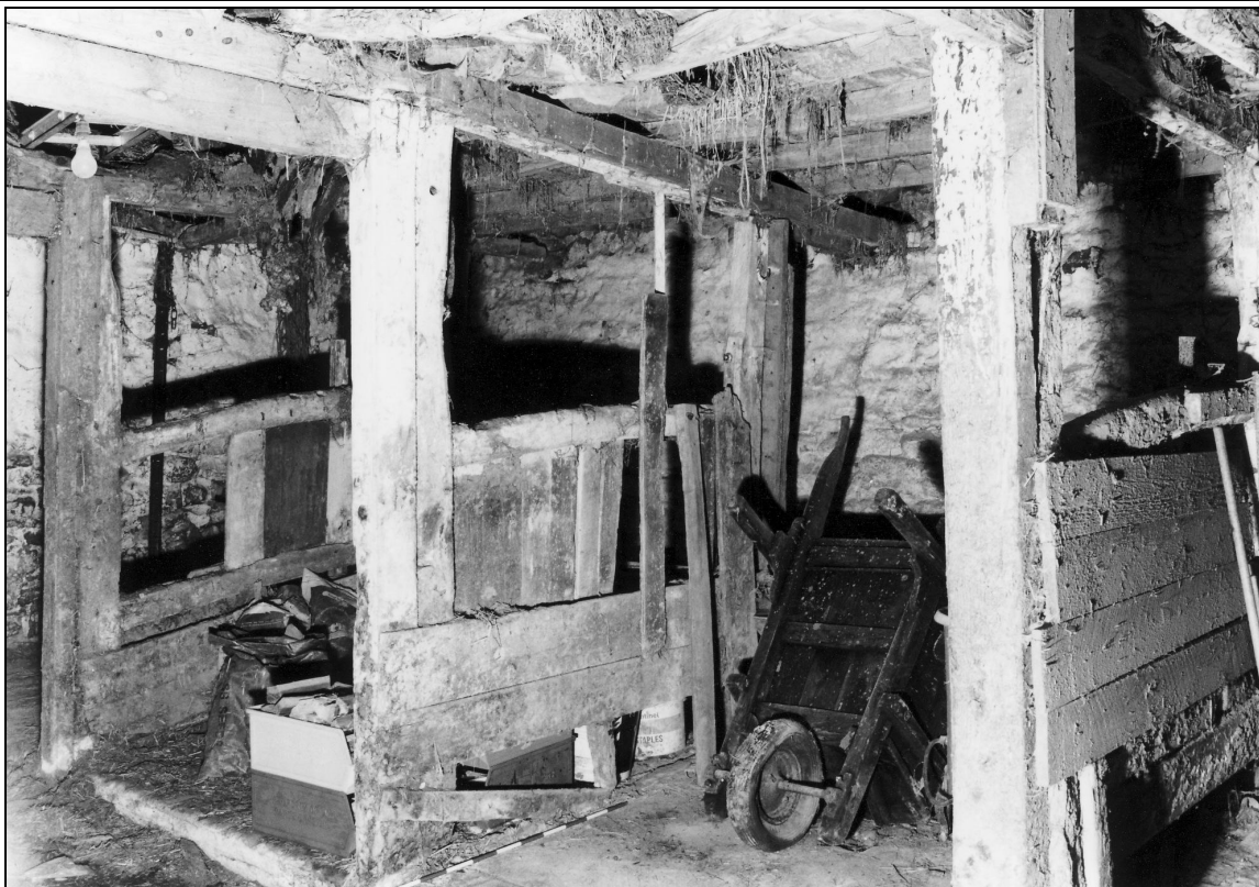
Photo 20: Altered stable divisions (boskins) along north side of stable, from the south-east
