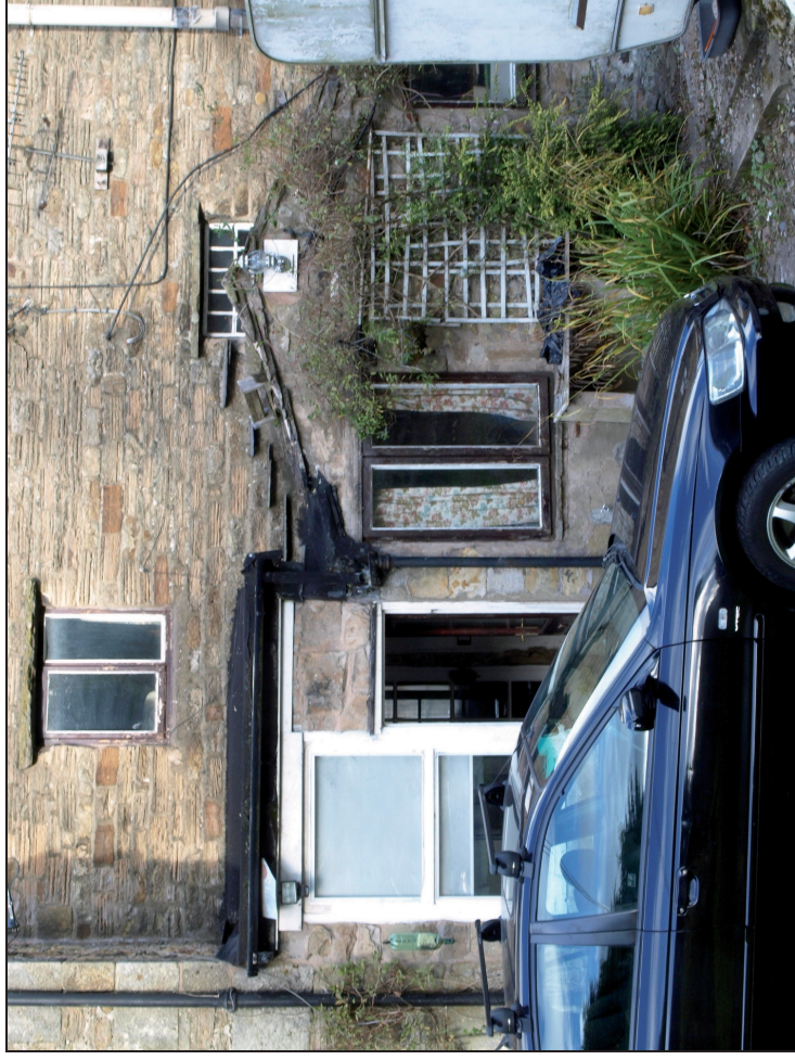
Photo 10: Back kitchen at foot of rear elevation: 19th century part under stone slate roof to right, 1980s addition under flat roof at left
