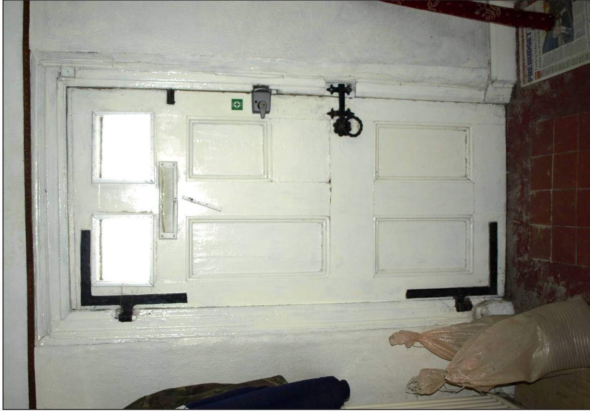
Photo 3: Rear of front door: note L-hinges
