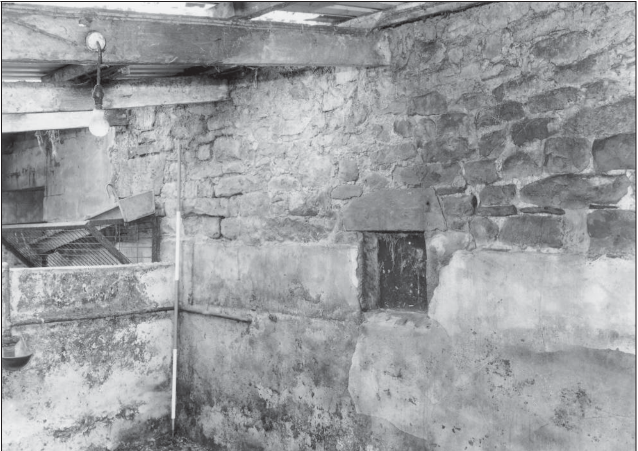
Photo 7: Muck hole and blocked breathers in east gable of barn
