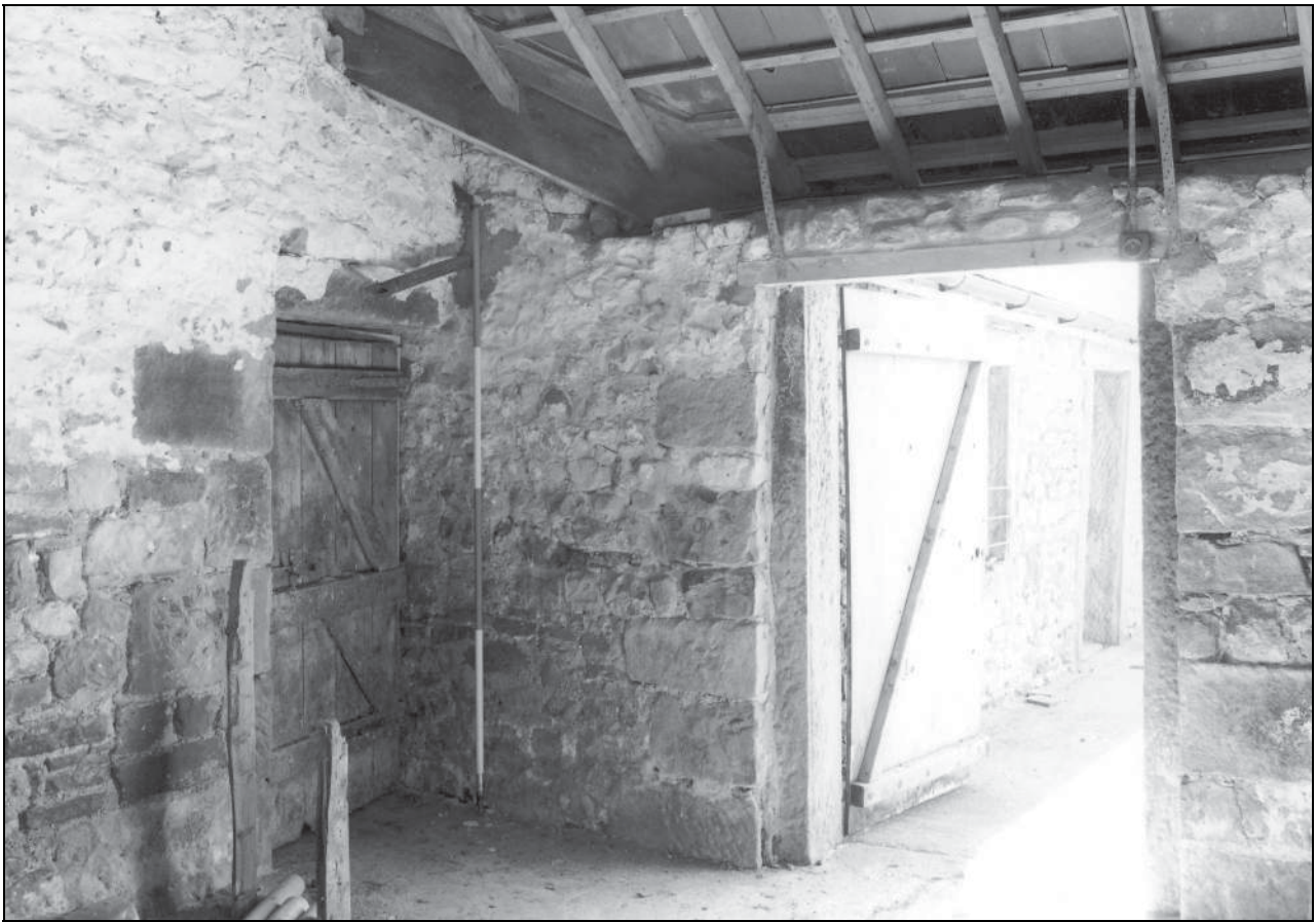
Photo 27: Interior of second loose box to east of farmhouse, from the north-west
