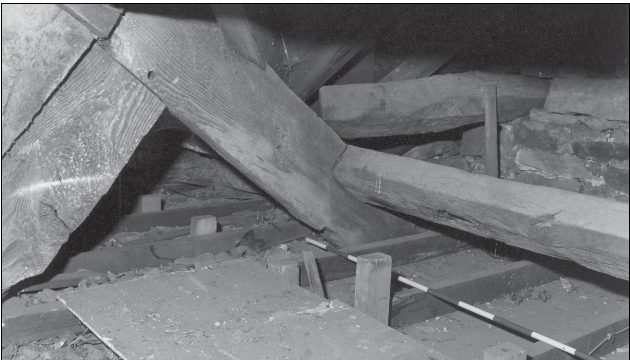
Photo 26: The 17th century house: north roof truss in south-west wing, from the south-west, showing chamfered oak purlin
