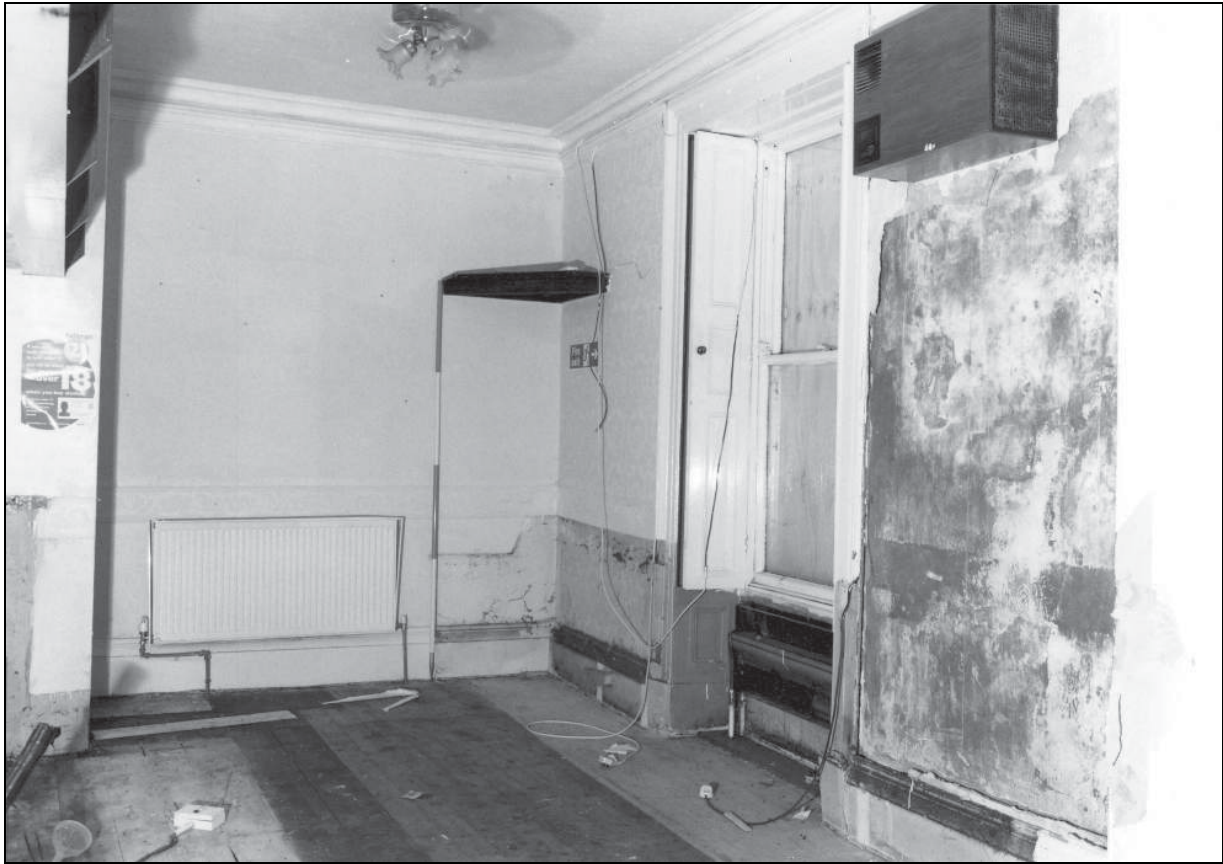
Photo 62: The 19th century house: north-west ground floor day room, from the south-east
