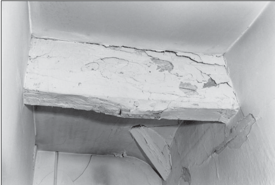
Photo 19: The 17th century house: sawn-off tenon in tie beam soffit, south-west wing
