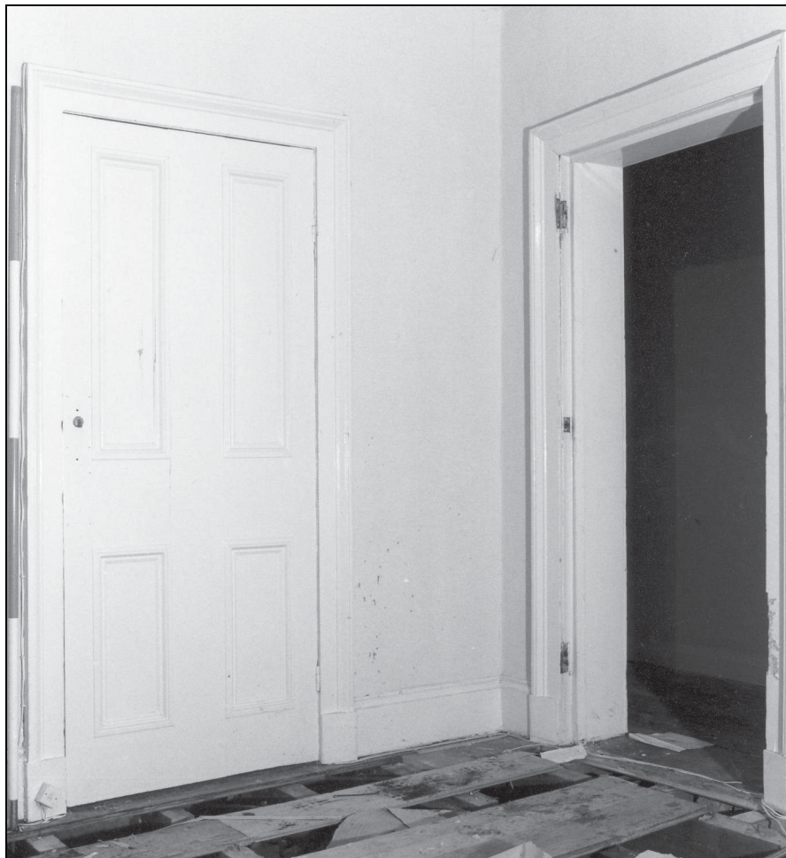
Photo 79: The 19th century house: original four panel door to closet, in bedroom on north side of house
