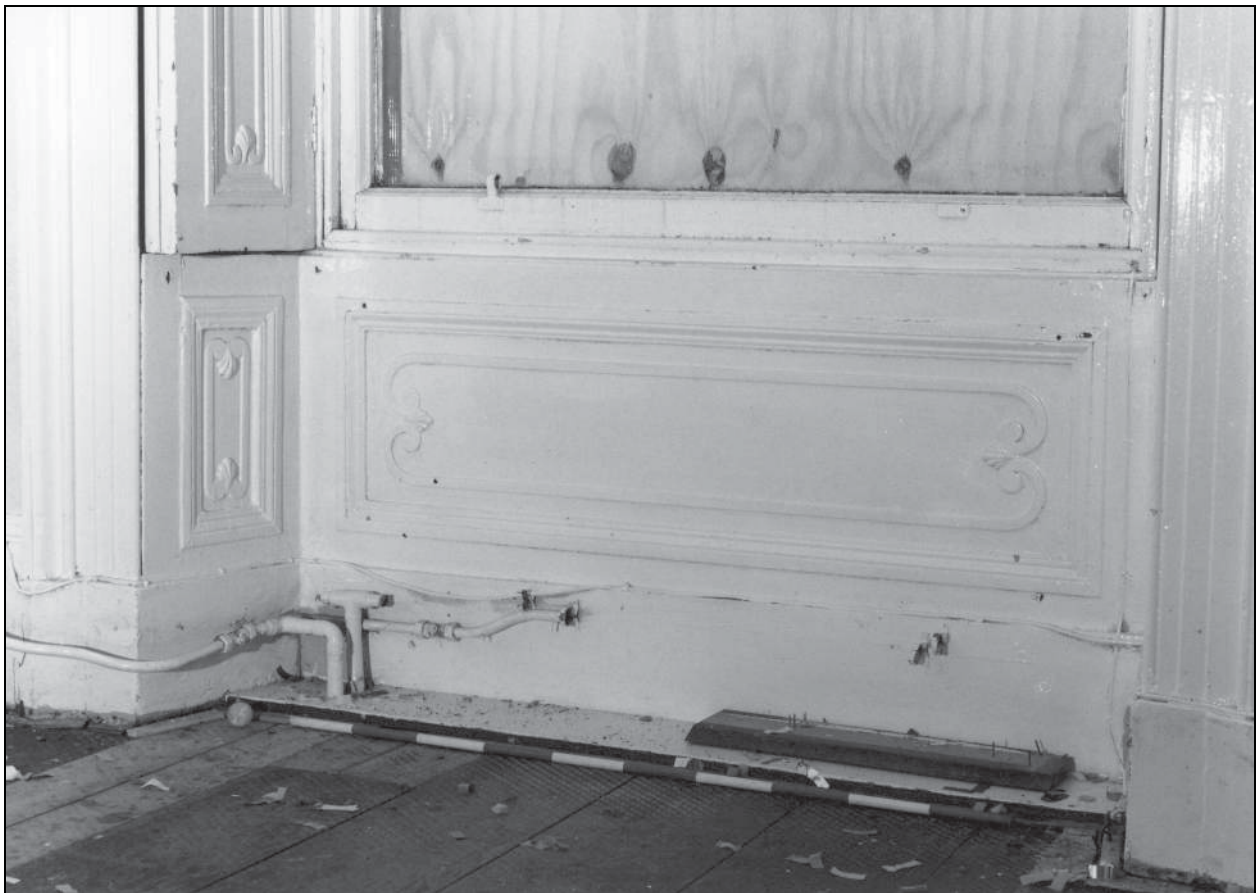
Photo 60: The 19th century house: detail of panelling below window, north side of north-east ground floor room
