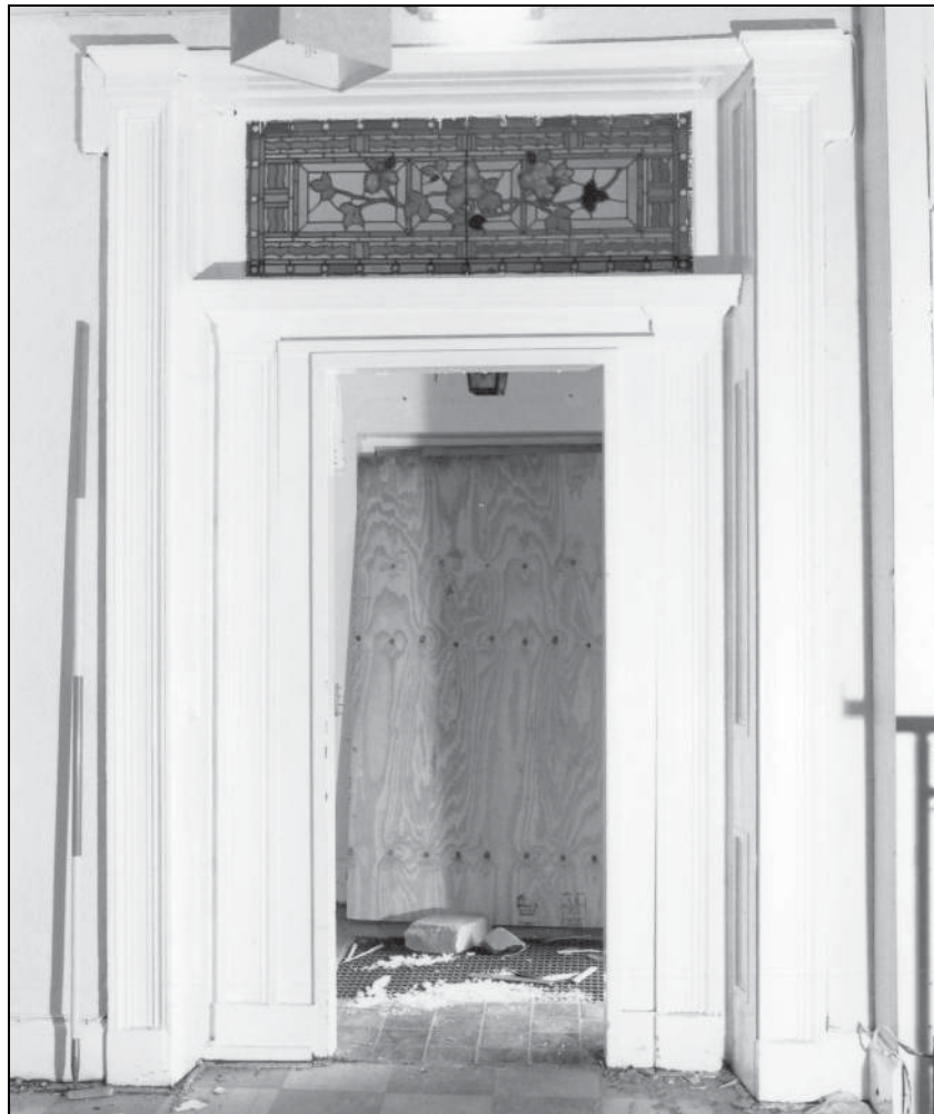
Photo 45: The 19th century house: internal view of east doorway to entrance hall
