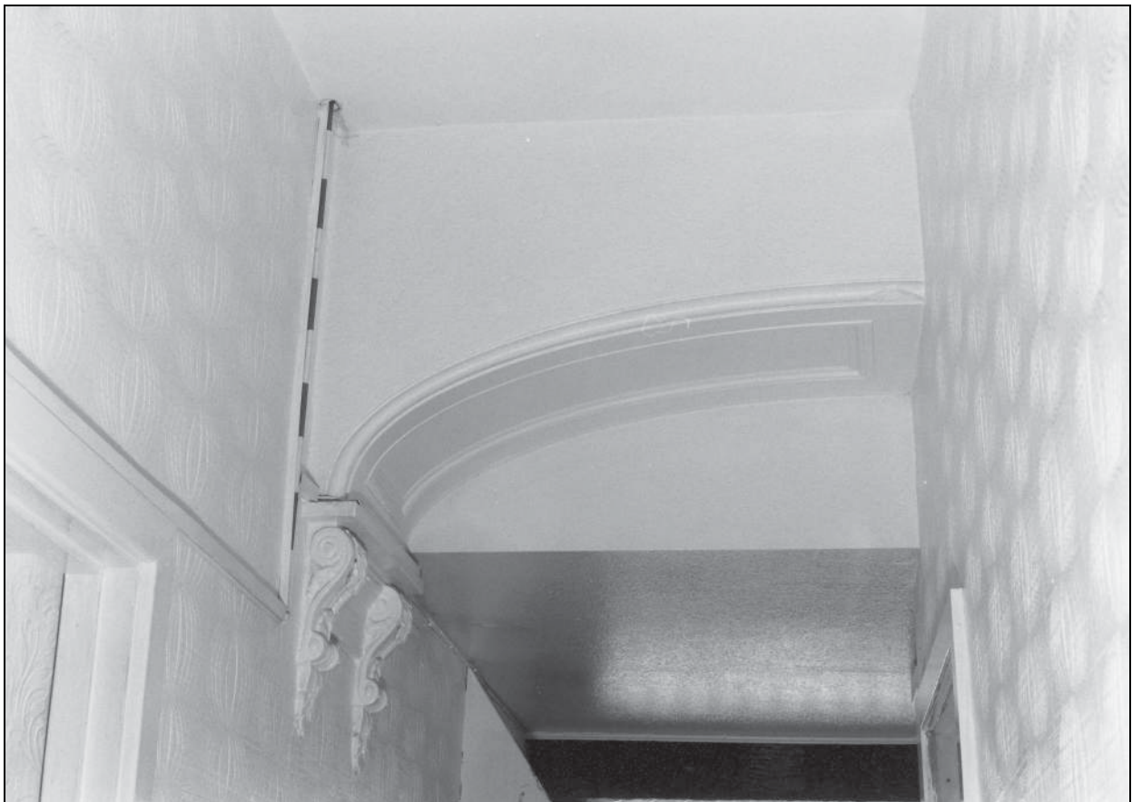
Photo 48: The 19th century house: arch originally between entrance hall and staircase, from the west
