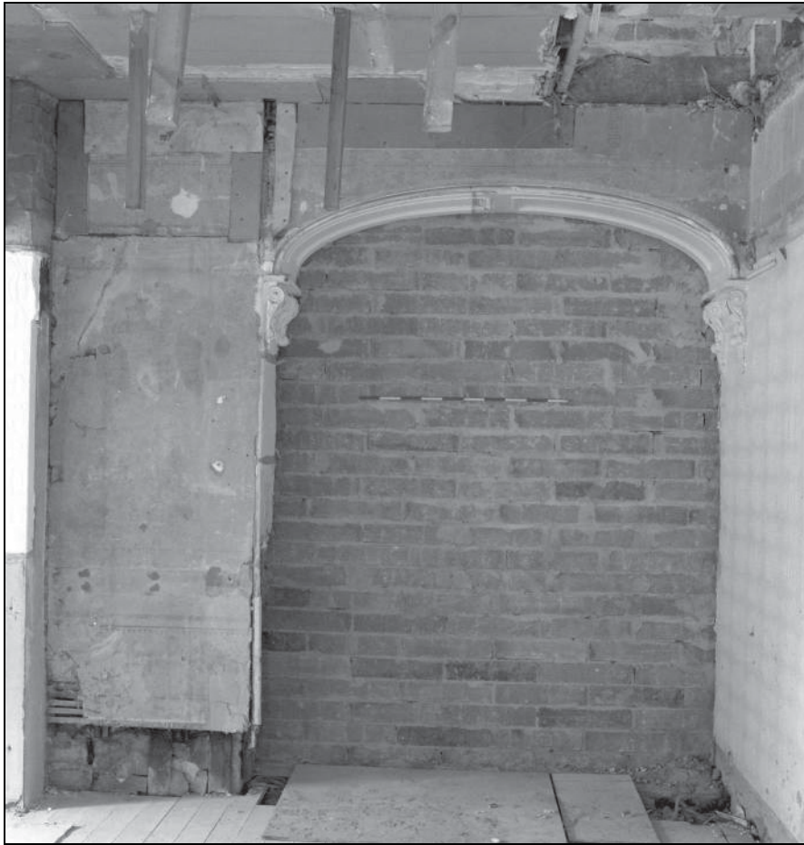
Photo 46: The 19th century house: arch originally between entrance hall and staircase, from the east
