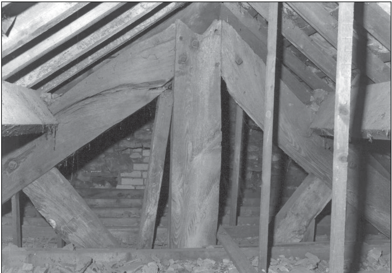
Photo 20: The 17th century house: south roof truss in south-west wing, from the north
