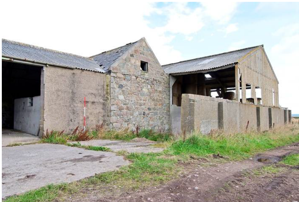
Phase 1 agricultural building (centre), infilled barn wall (left) and straw and hay storage (right)
