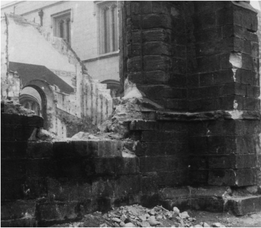
III 31 Demolition of the church (foreground) with the 1768 extension (top left) (Aberdeen City Libraries).
