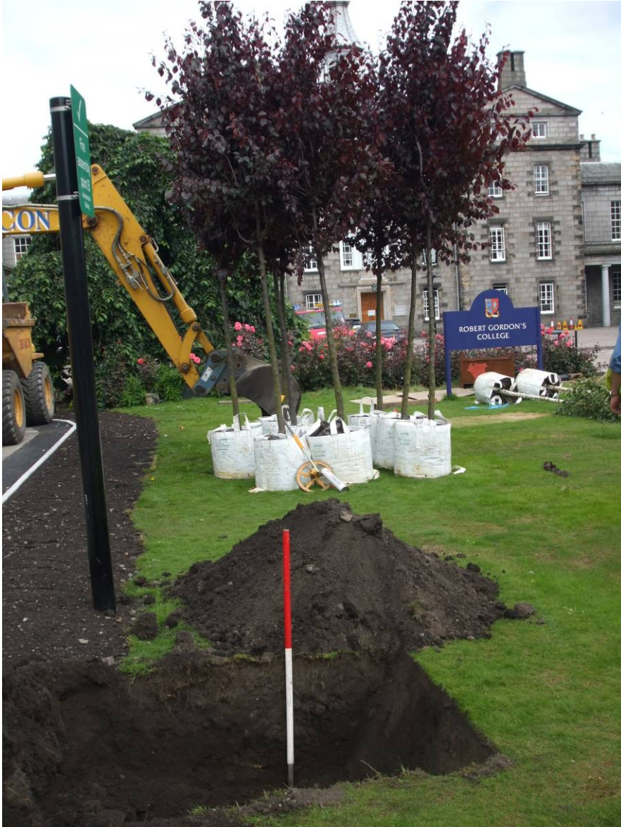
Pits for tree planting, with trees and Robert Gordon's College in the background, facing north
