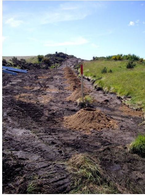
Plate 14: General view showing excavated fence post holes by auguring within area of fenceline clearance, facing north-west
