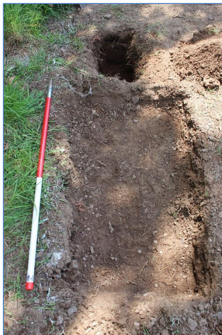
Figure 2: Post-excitation of trench for trough base and hole for new water toby
