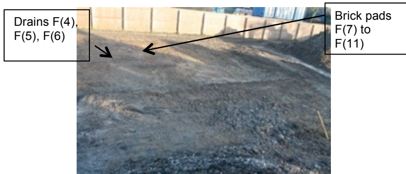
Figure 30: South facing view of drain F(4), F(5), F(6) and brick pad F(8) locations
