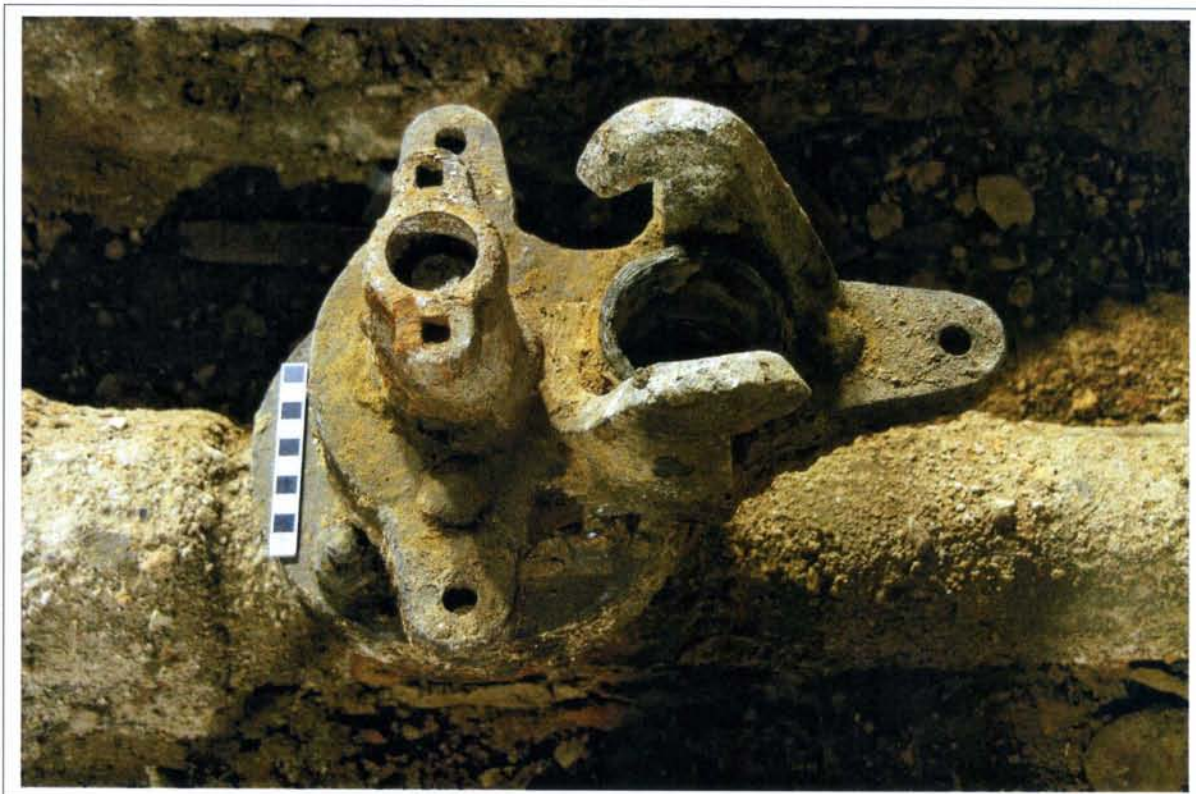
Plate 17: View of hydrant fitting, Scale 1x0.1m
