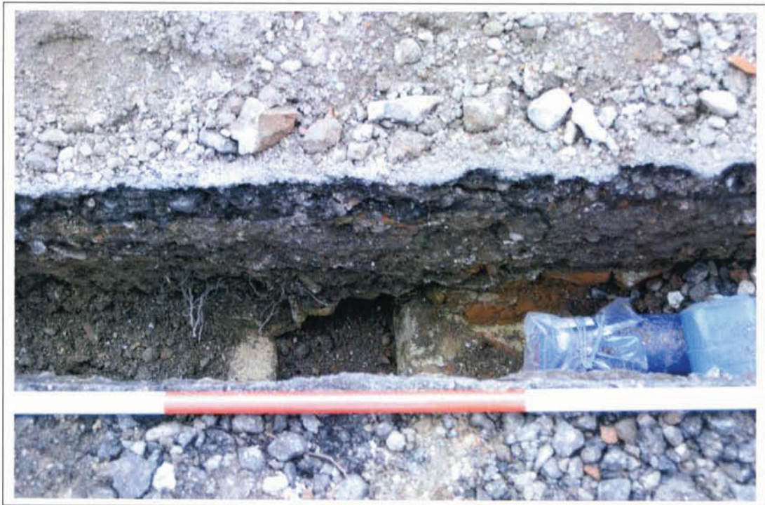
Plate 12: View of damaged brick culvert
