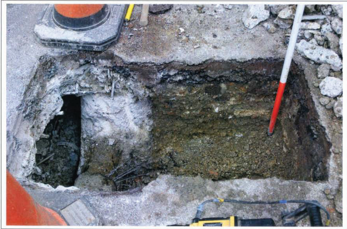
Plate 10: View of heating duct butted against by possible in situ deposits
