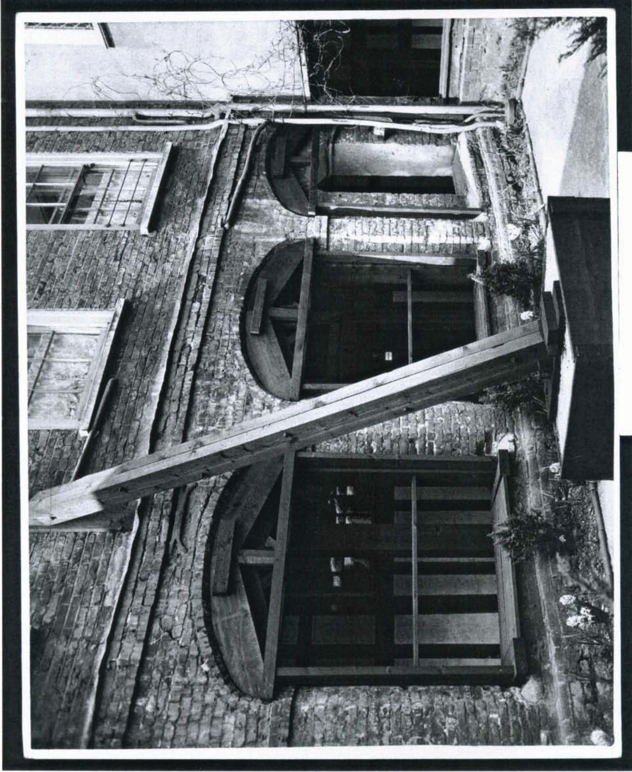
Figure 12. Photograph of east facing wall within courtyard area of Canons cloister, c. 1950, prior to consolidation work.
