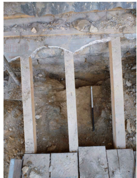
Plate 19 Junction between the east curtain wall and east wall of the east range
