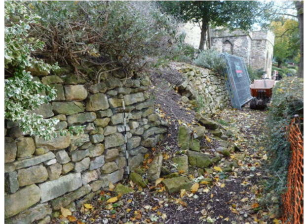
Plate 1 Location of intervention showing failed revetment wall looking east (scale 1.0m)
