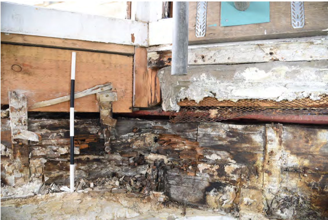
Plate E72 Detail of exposed timberwork of lantern base at junction between NE and E elevations showing decay, looking NE, scale 50cm (BRH054)
