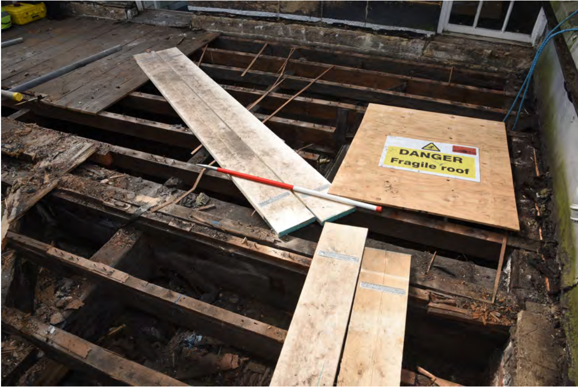
Plate E93 Roof construction following board lift, SW side, looking SE, scale 1.0m (BRH130)
