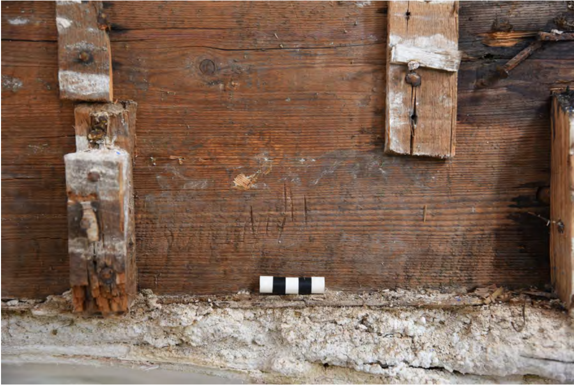
Plate E79 Detail – Possible chisel marks and red chalk setting-out line, looking SW, scale (BRH062)
