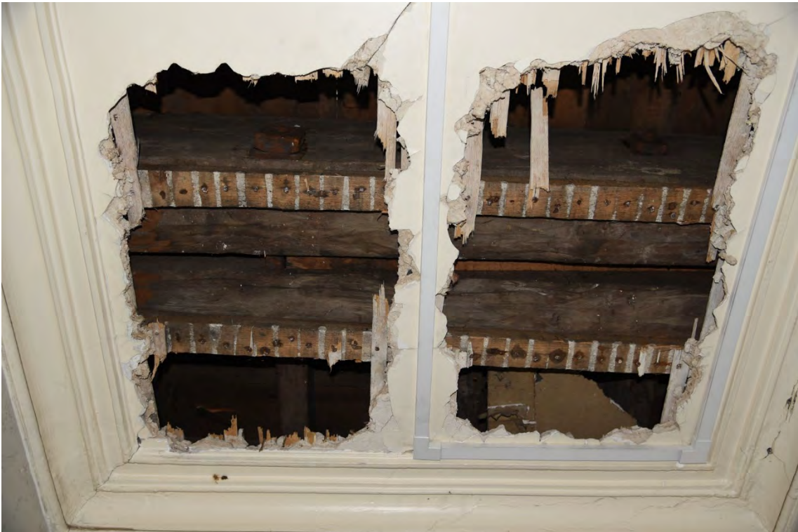
Plate E40 Internal view into vestibule roof space from north corridor at second floor level showing ironwork bolt pinning the tie-beams, looking E (BRH218)
