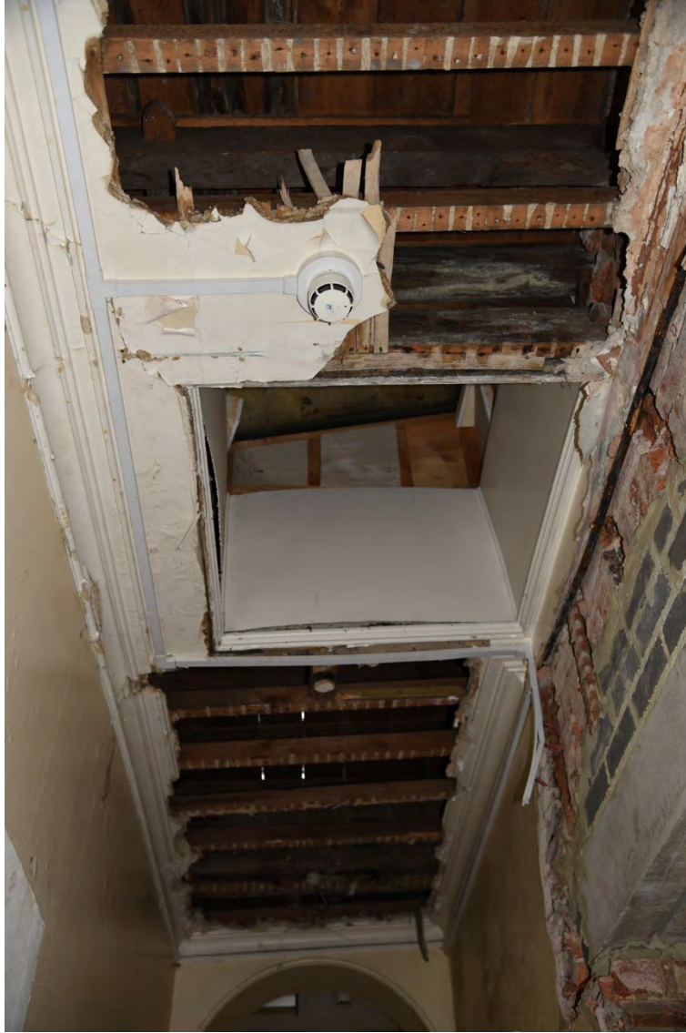
Plate E46 Internal view of vestibule roof E skylight from east corridor at second floor level, looking N (BRH224)
