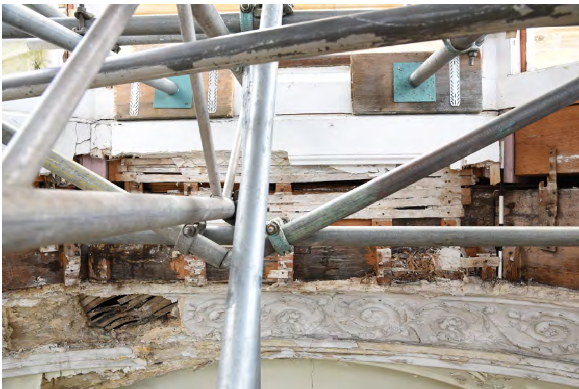
Plate E66 Interior view, exposed timbers of lantern base, looking S, scale 50cm (BRH039)
