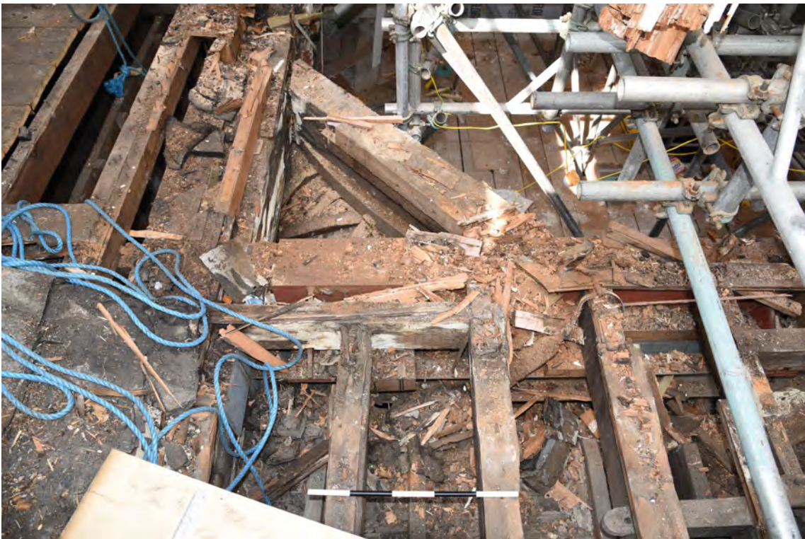
Plate E108 View showing roof construction SE pendentive, looking W, scale 50cm (BRH145)
