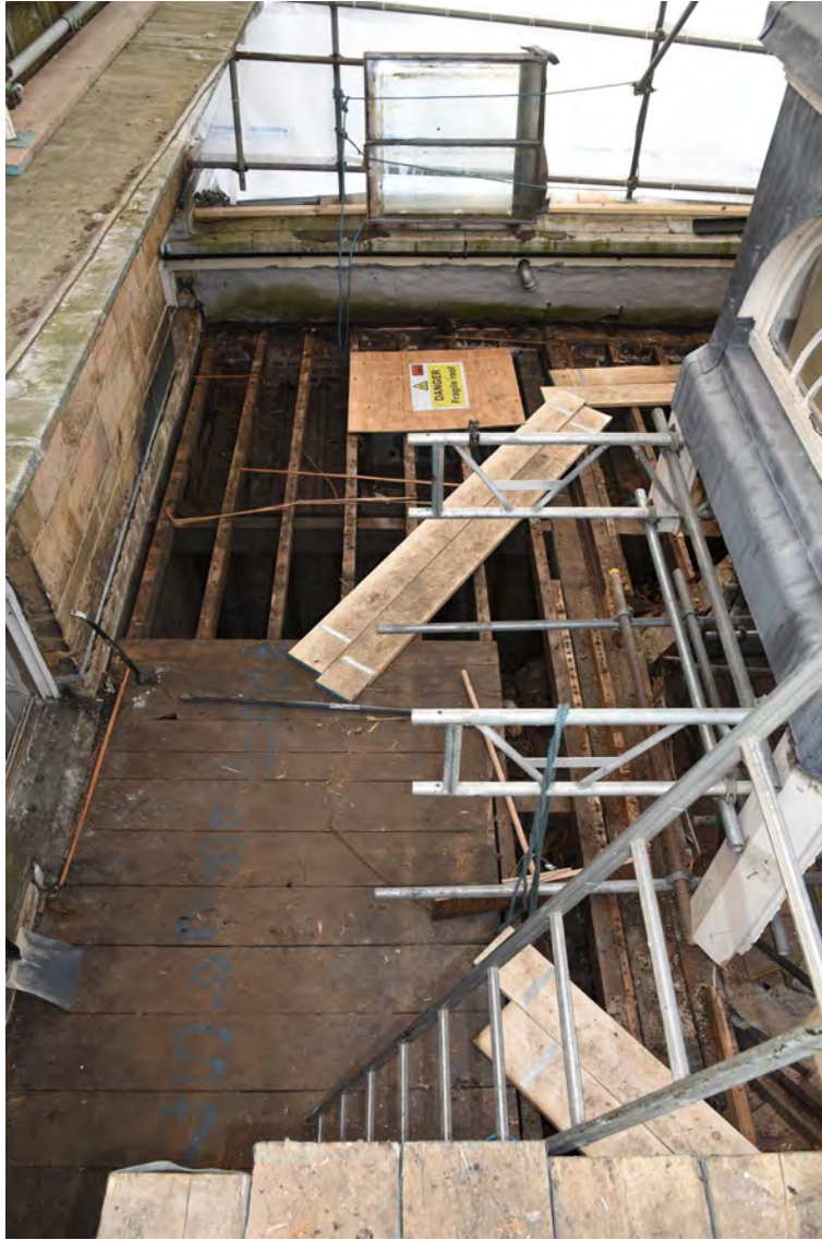
Plate E209 General view of flat roof following opening-up works, looking W (BRH165)
