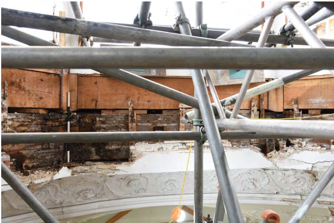
Plate E62 Interior view, exposed timbers of lantern base, looking N, scale 50cm (BRH035)
