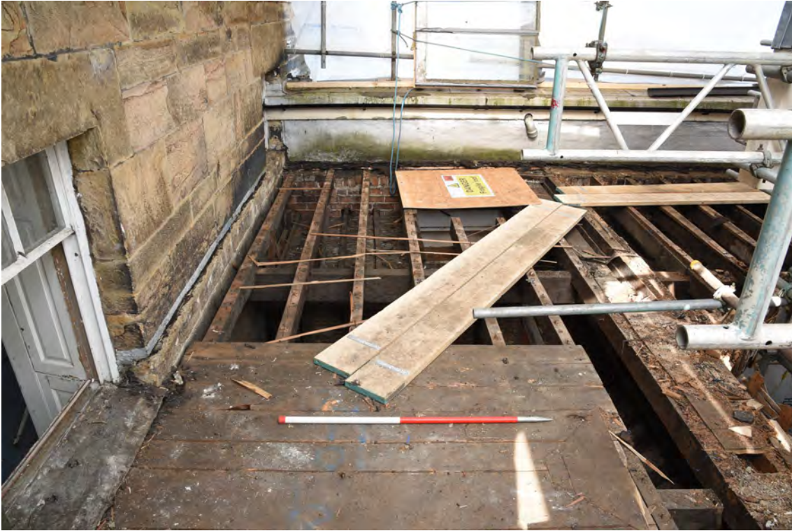
Plate E207 Roof construction following board lift, S side, looking W, scale 1.0m (BRH117)
