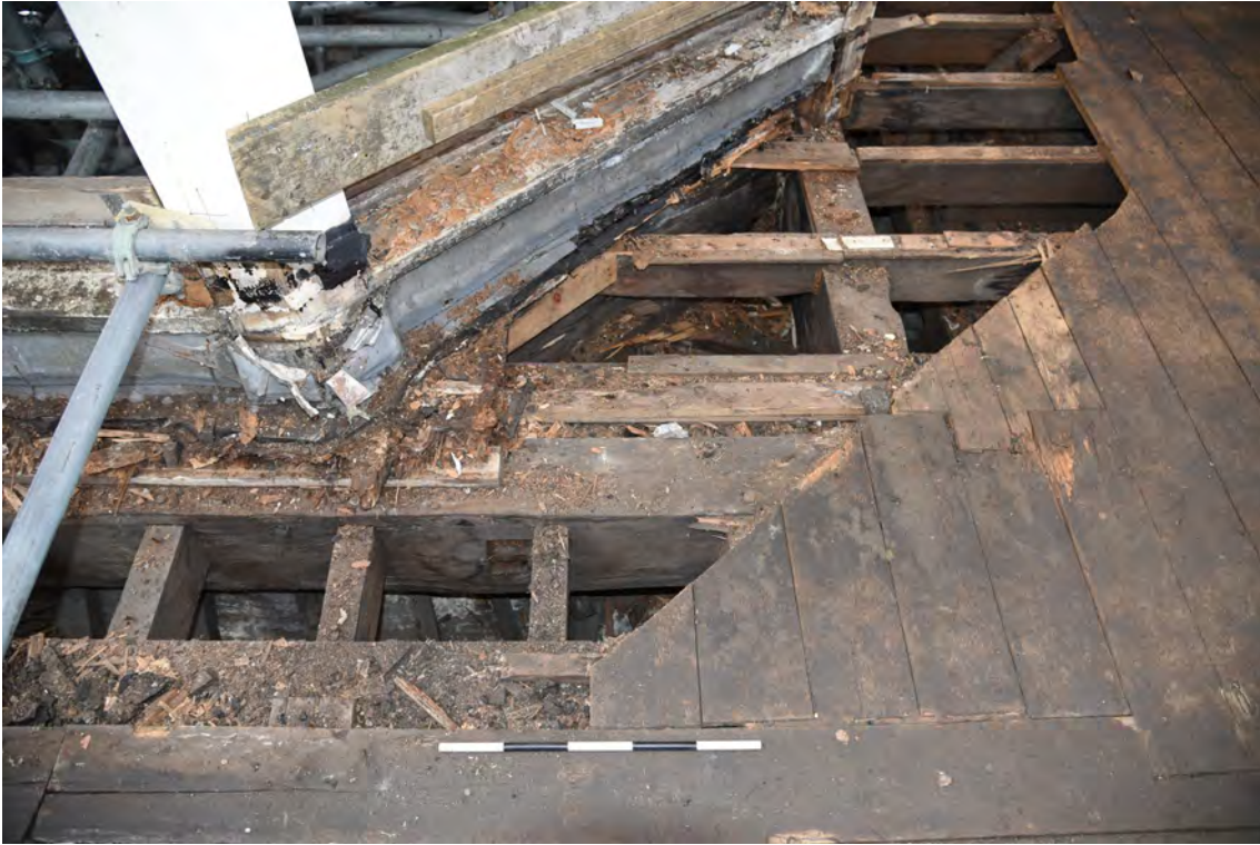
Plate E185 Lantern base, tie beam and roof joists, NW side, looking S, scale 50cm (BRH095)
