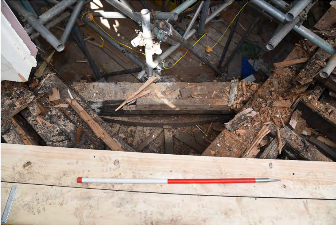
Plate E97 SE elev. lantern base and vestibule roof construction, looking NW, scale 1.0m (BRH134)
