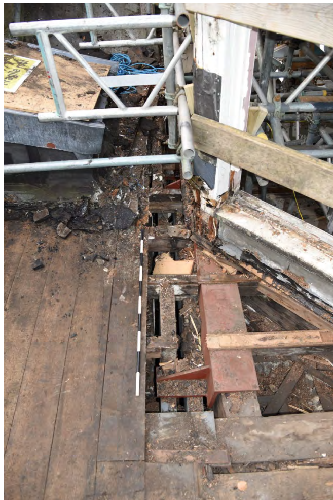
Plate E172 View into roof space following board lift showing modern steel repairs, looking S, scale 1.0m (BRH081)
