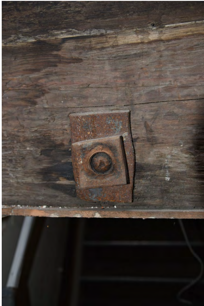
Plate E115 Detail of iron bolt fastening in S tie-beam, looking S (BRH161)
