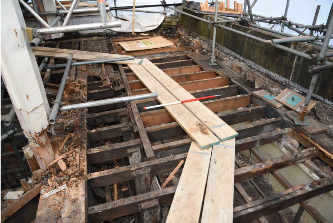
Plate E89 Roof construction following board lift, N side, looking W, scale 1.0m (BRH126)
