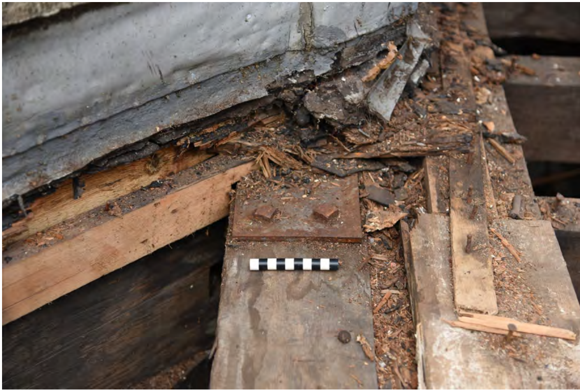
Plate E181 Detail of steel plate repair, looking W, scale 10cm (BRH090)
