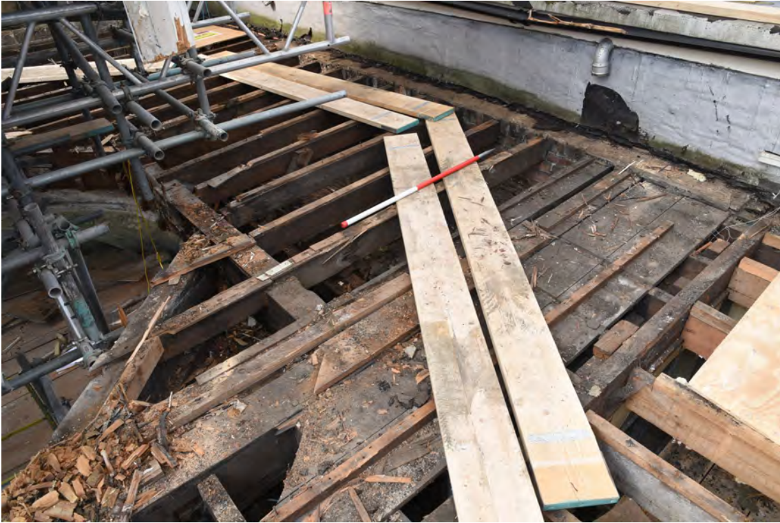
Plate E91 Roof construction following board lift, W side, looking SW, scale 1.0m (BRH128)
