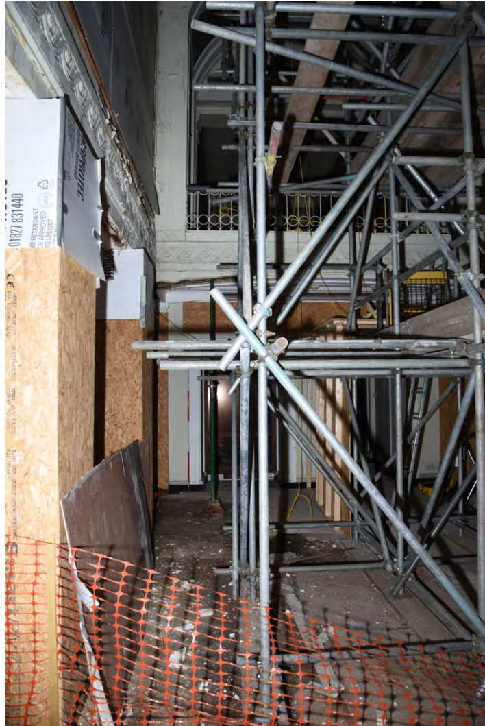
Plate E23 General view, ground floor of vestibule during works, looking S (BRH201)
