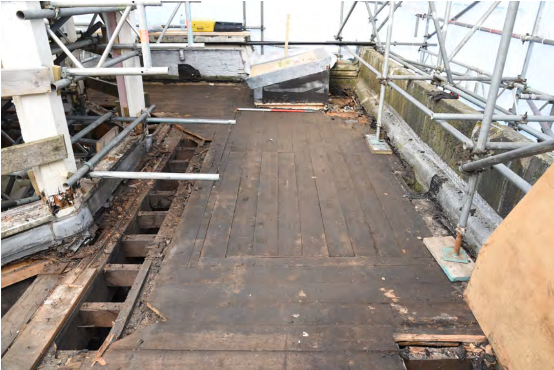
Plate E170 Flat-roof boards after removal of felt/bitumen, N side, looking W, scale 1.0m (BRH079)
