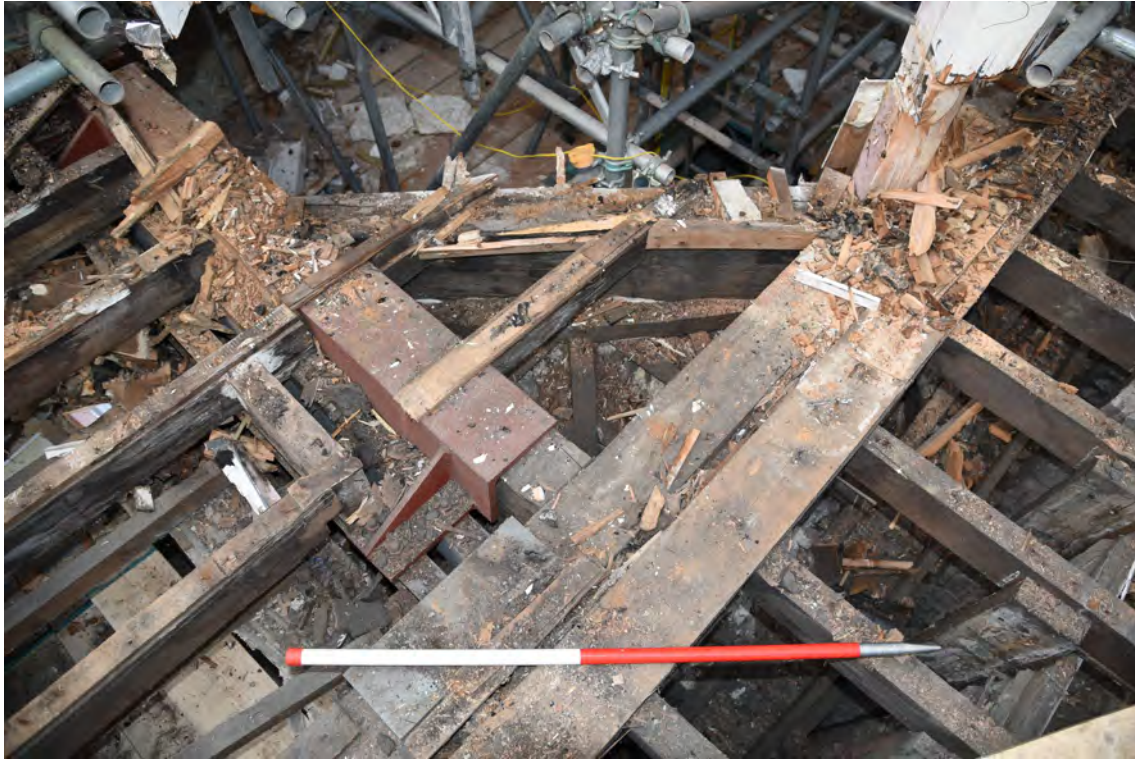
Plate E95 NE elev. lantern base and vestibule roof construction, looking SW, scale 1.0m (BRH132)
