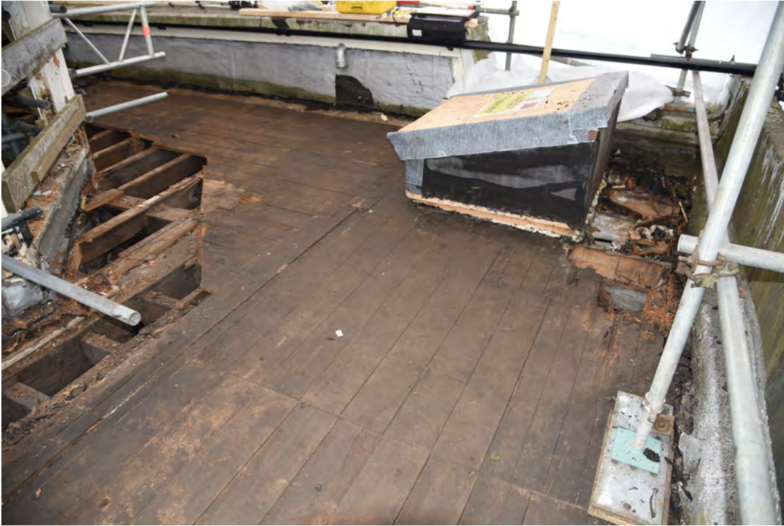
Plate E199 Flat-roof boards after removal of felt/bitumen, NW side, looking SW (BRH109)
