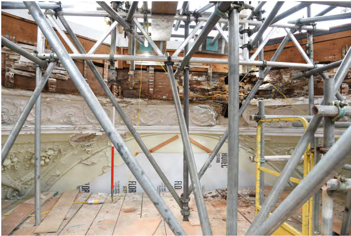
Plate E11 Interior view of decorative plasterwork frieze, looking W, scale 1.0m (BRH033)
