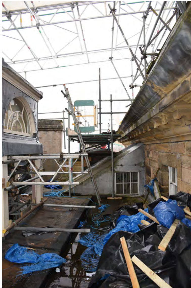
Plate E164 General view vestibule roof S of lantern, looking E (BRH020)
