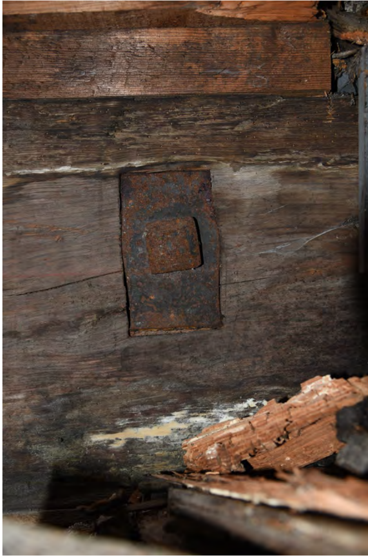
Plate E116 Detail of iron bolt fastening in S tie-beam, looking S (BRH162)
