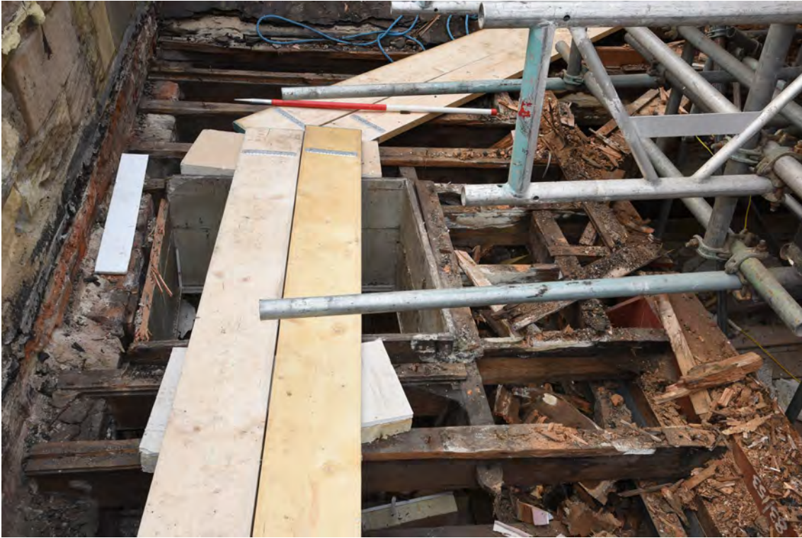
Plate E87 Roof construction following board lift, E side, looking S, scale 1.0m (BRH124)
