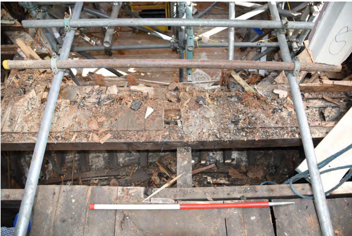
Plate E98 S elevation lantern base and vestibule roof construction, looking N, scale 1.0m (BRH135)
