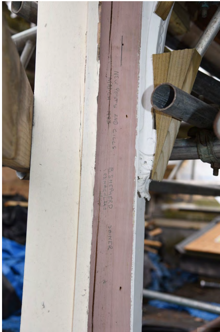
Plate E118 S elevation window frame upright timber with joiner's pencil inscription reads - 'NEW POSTS AND CILLS MARCH 1983 B SHEPHERD 93 HAIGH LANE HAIGH JOINER', looking SW (BRH074)
