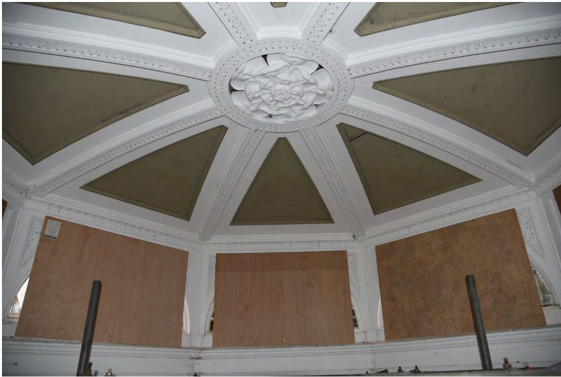
Plate E129 View into the lantern ceiling space looking S, looking S (BRH077)
