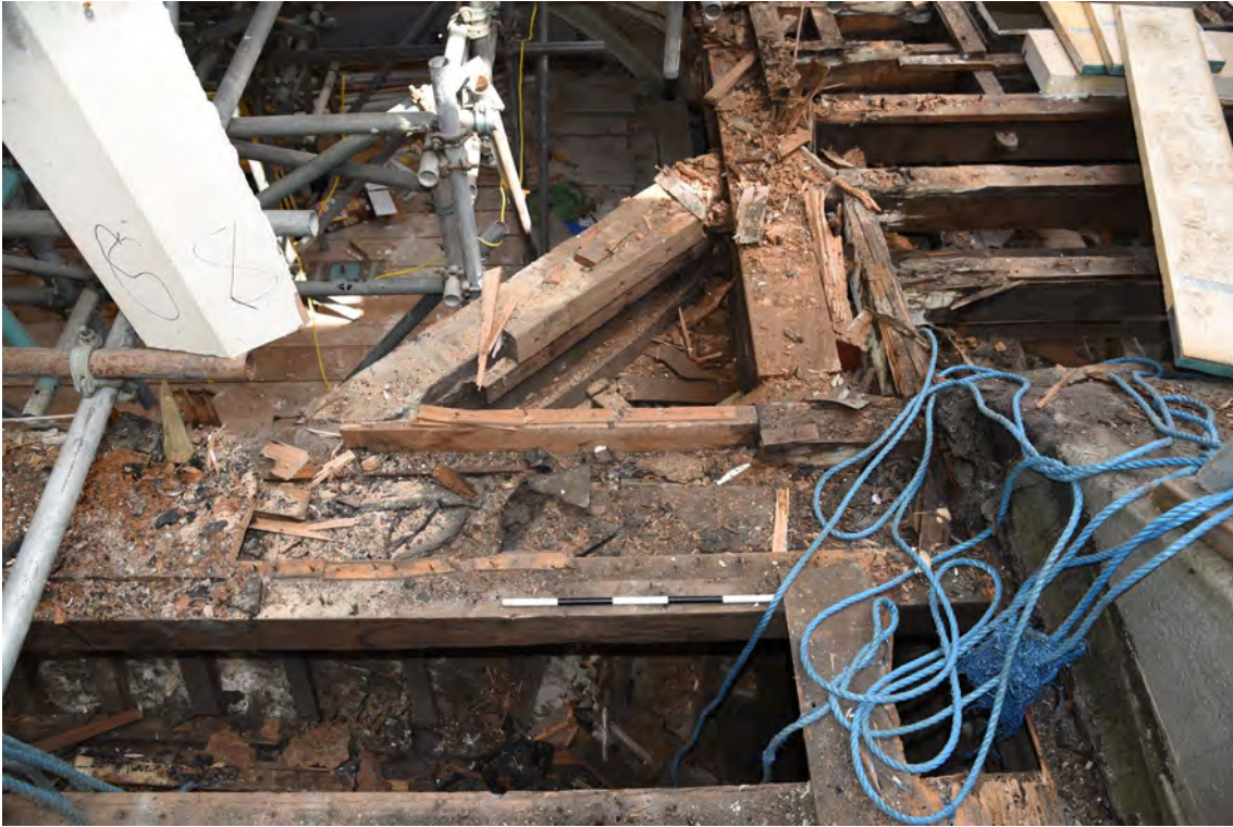
Plate E109 View showing roof construction SE pendentive, looking N, scale 50cm (BRH146)
