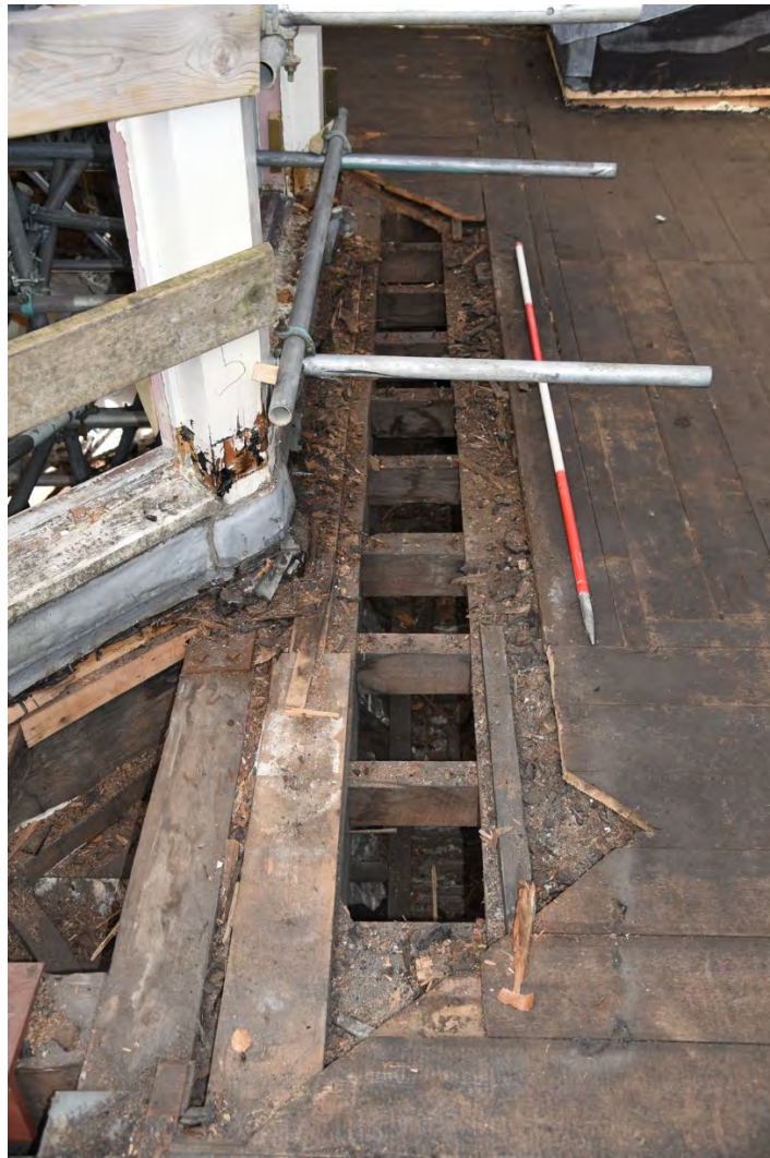
Plate E173 View of roof joists and tie beam following board lift, looking W, scale 1.0m (BRH082)
