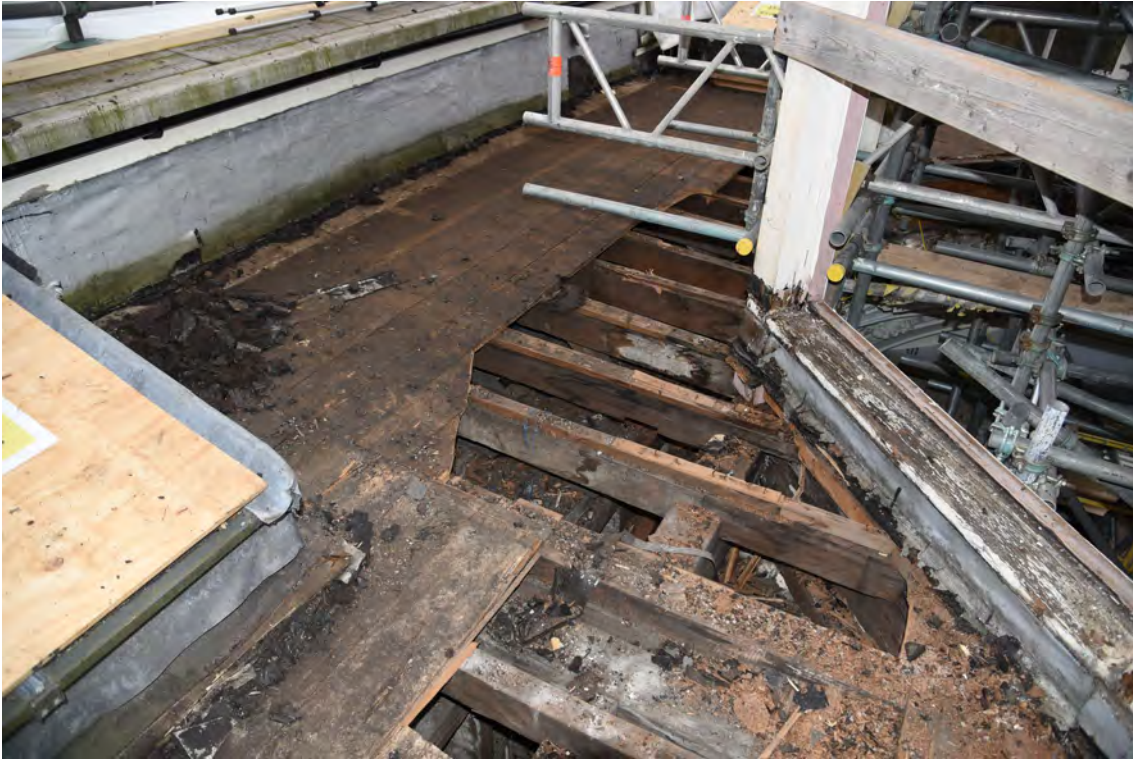
Plate E201 Flat-roof boards after removal of felt/bitumen, SW side, looking NW (BRH111)
