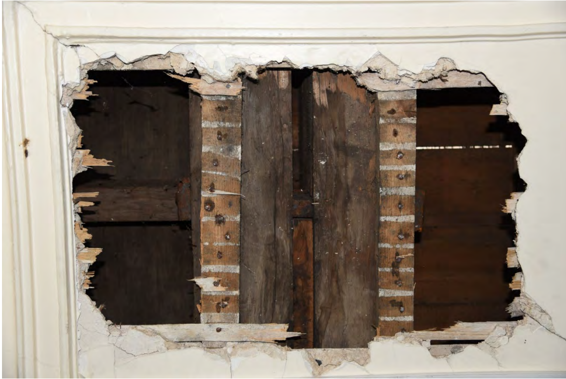
Plate E41 Internal view into vestibule roof space from north corridor at second floor level showing ironwork bolt pinning the tie-beams, looking S (BRH219)
