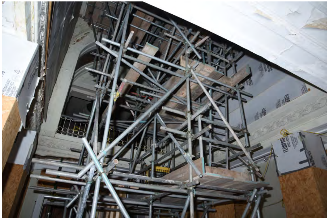
Plate E24 View of scaffold tower accessing lantern interior, looking S (BRH202)
