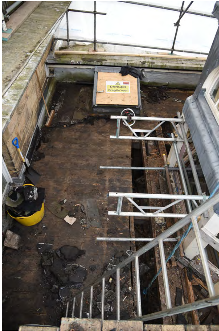
Plate E206 Flat-roof boards after removal of felt/bitumen, S side, looking W (BRH116)
