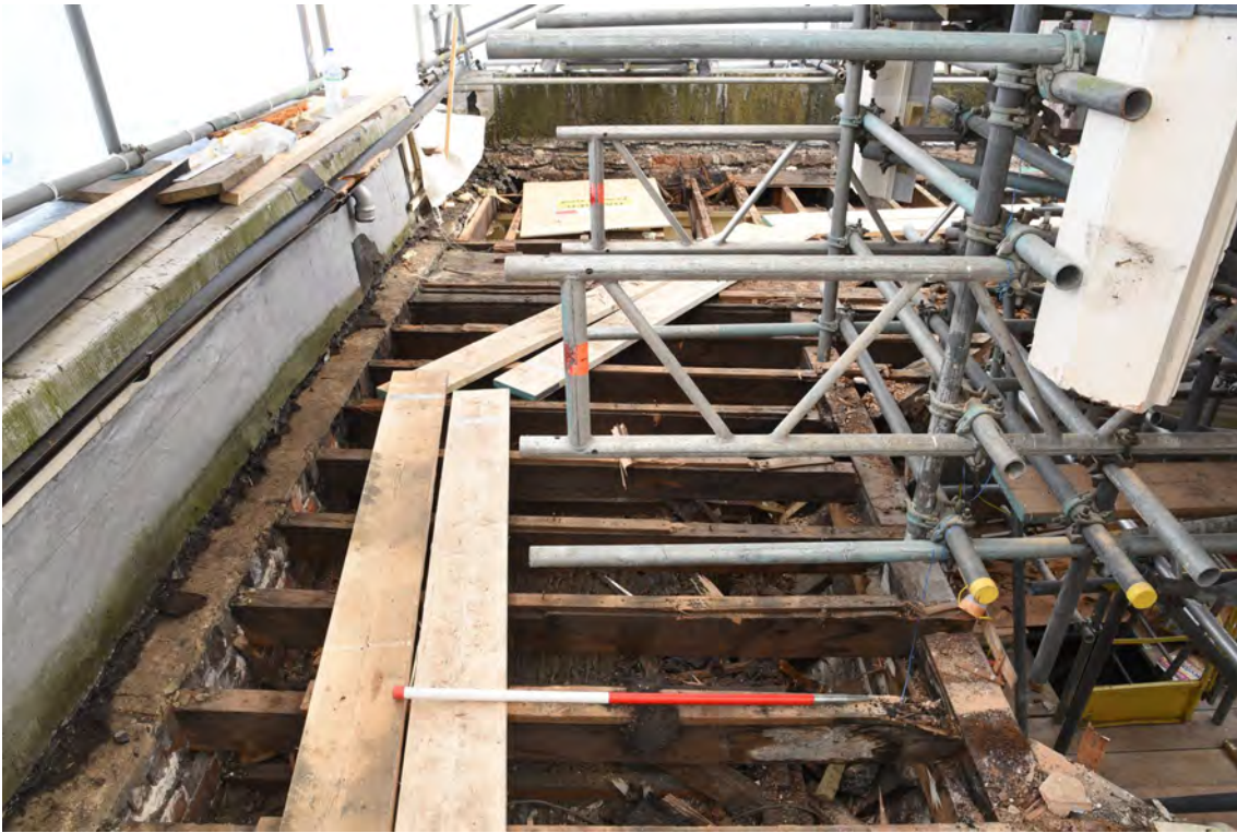
Plate E83 Roof construction following board lift, W side, looking N, scale 1.0m (BRH120)
