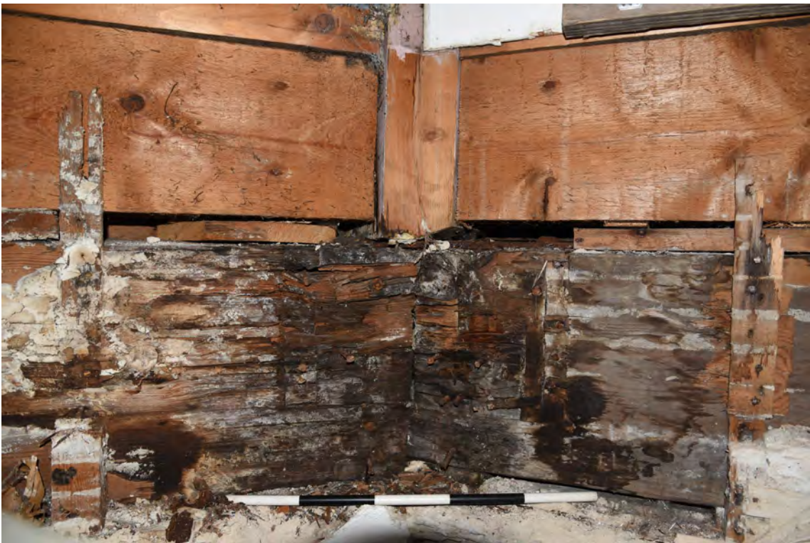
Plate E70 Detail of exposed timberwork of lantern base at junction between N and NW elevations showing decay, looking NW, scale 50cm (BRH052)
