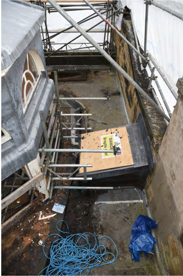
Plate E163 Vestibule flat roof and E skylight before works, looking N (BRH019)
