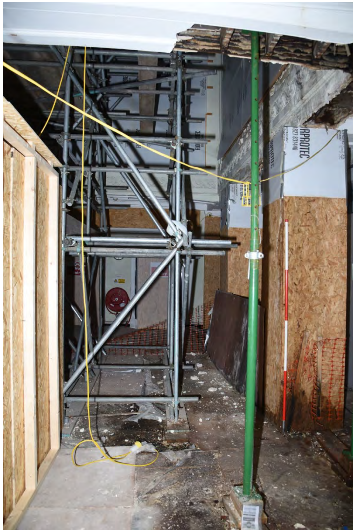
Plate E22 General view, ground floor of vestibule during works, looking N, scale 1.0m (BRH200)
