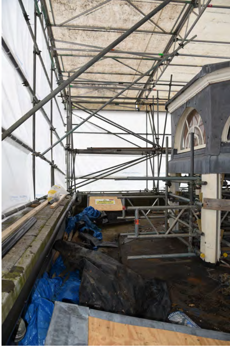
Plate E165 General view vestibule roof W of lantern, looking N (BRH021)
