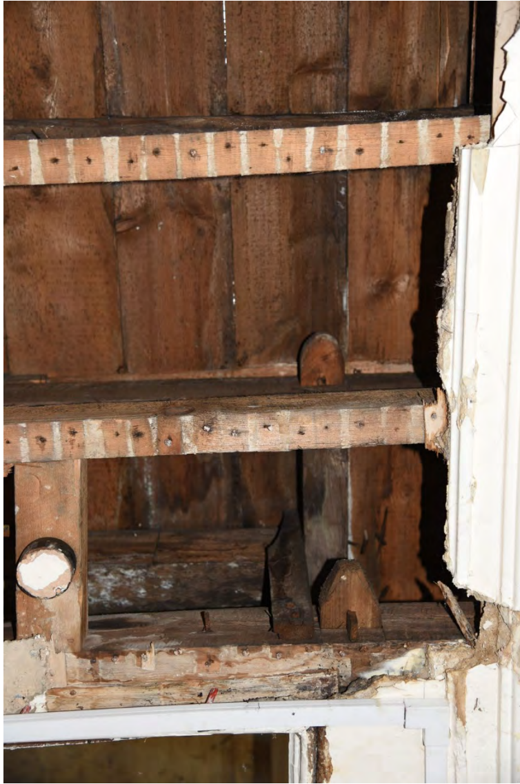
Plate E45 Internal view into vestibule roof space from east corridor at second floor level, detail of E skylight construction, looking S (BRH223)
