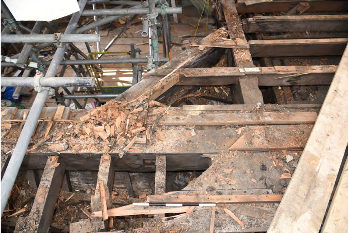
Plate E105 View showing roof construction NW pendentive, looking S, scale 50cm (BRH142)
