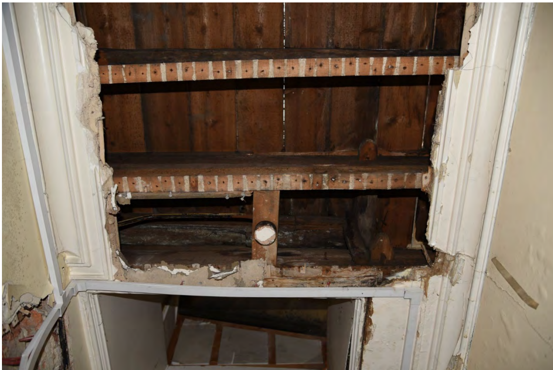
Plate E44 Internal view into vestibule roof space from east corridor at second floor level showing E skylight construction, looking S (BRH222)
