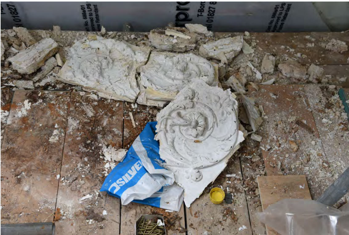
Plate E20 View of deteriorated decorative plasterwork from frieze (BRH064)
