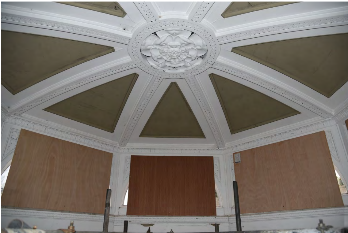
Plate E128 View into the lantern ceiling space looking E, looking E (BRH076)
