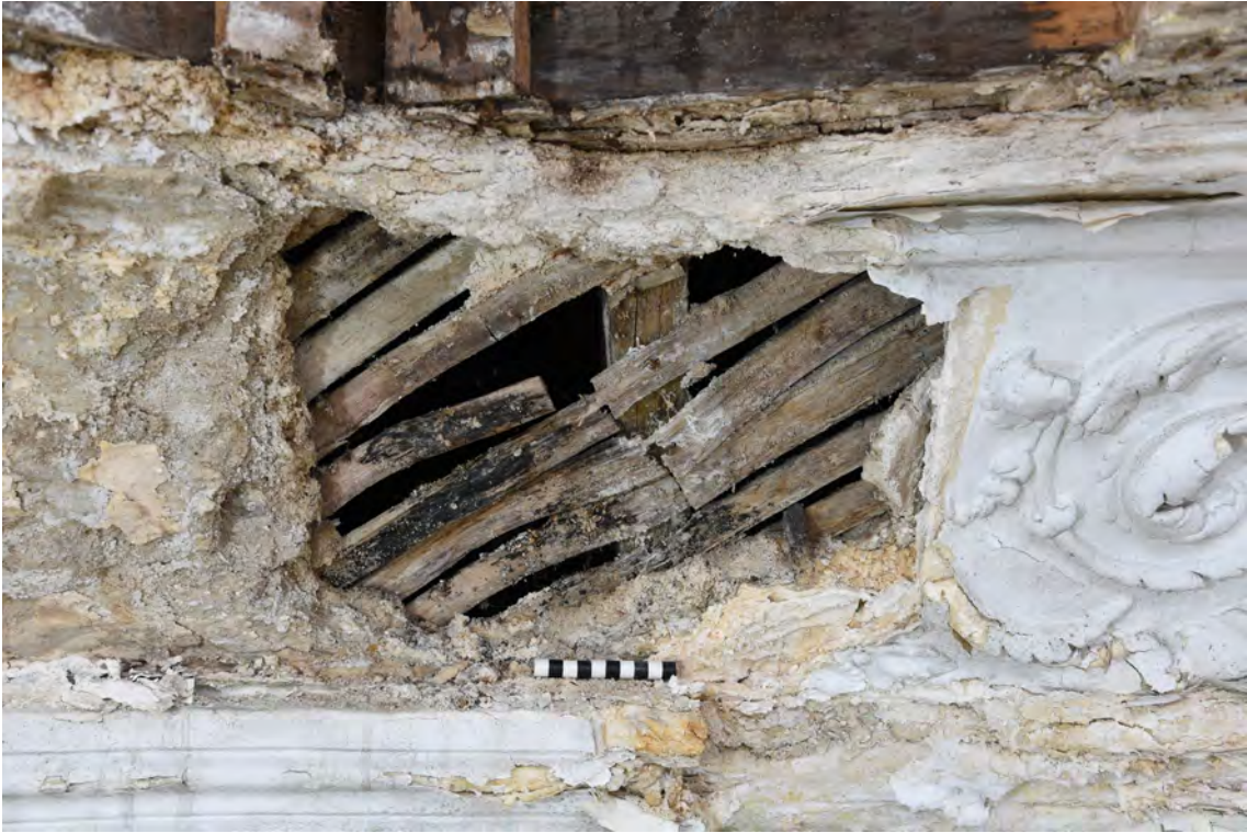
Plate E77 Detail – Plaster removal reveals lathwork beneath, looking S, scale 10cm (BRH059)
