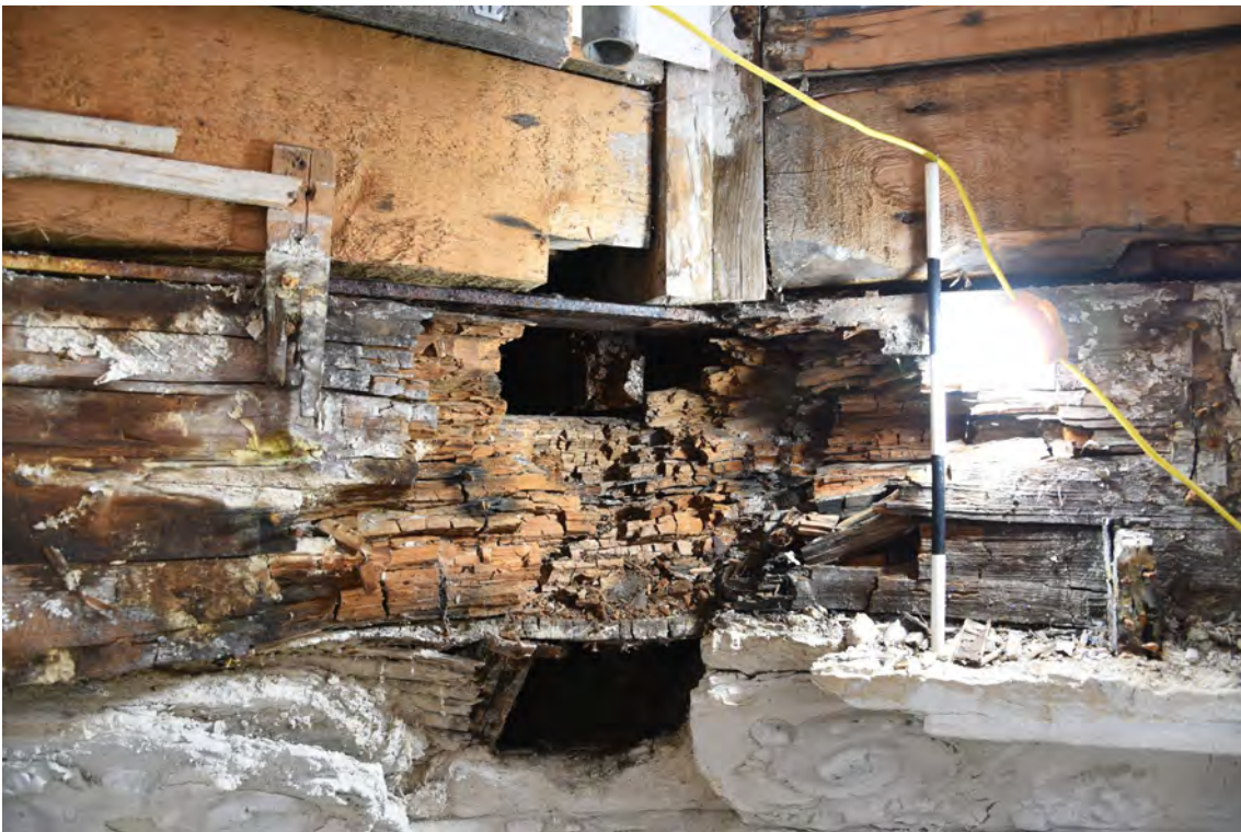
Plate E80 Detail – Exposed timberwork of lantern base at junction between W and NW elevations showing wood decay and later steel plate reinforcement, looking W, scale 50cm (BRH063)
