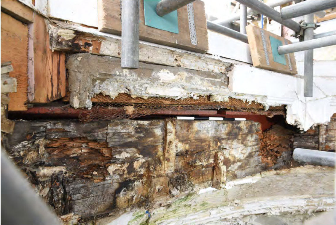
Plate E73 Detail of lantern base E elevation showing later steel reinforcement and extent of wood decay, looking SE, scale 50cm (BRH055)
