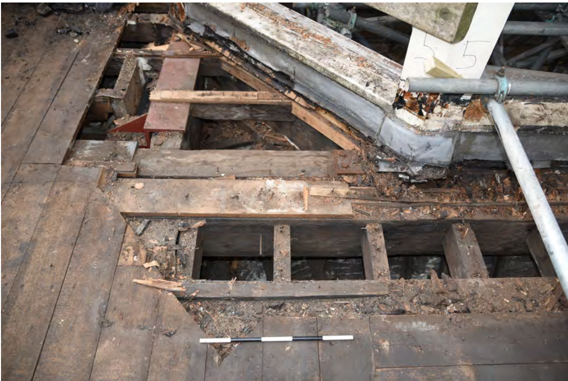
Plate E184 Lantern base, tie beam and roof joists, NE side, looking S, scale 50cm (BRH094)
