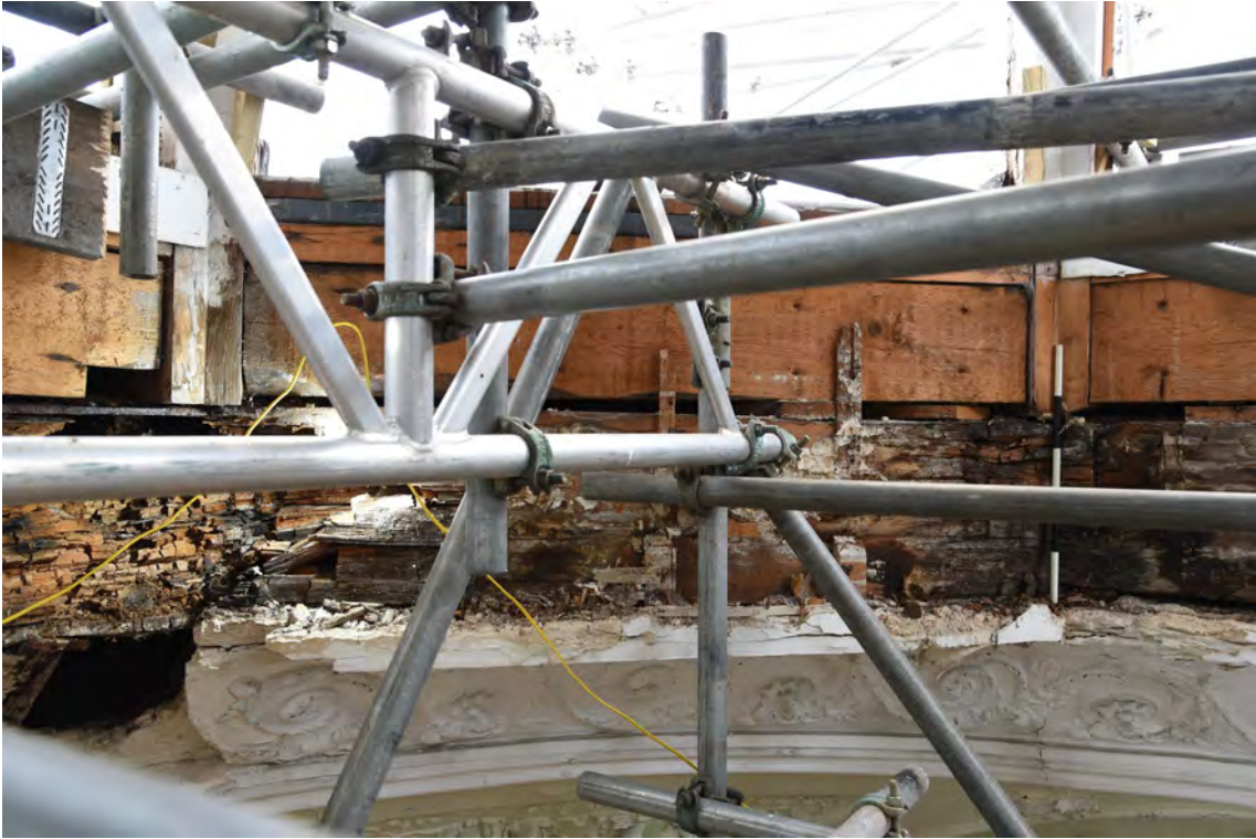
Plate E69 Interior view, exposed timbers of lantern base, looking NW, scale 50cm (BRH042)
