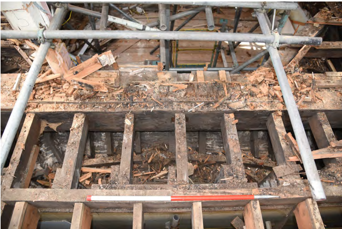
Plate E94 N elevation lantern base and vestibule roof construction, looking S, scale 1.0m (BRH131)
