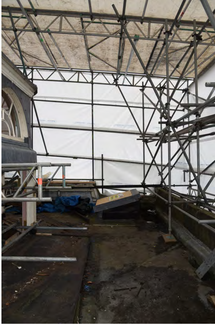
Plate E168 General view vestibule roof and NW skylight, N of lantern, looking W (BRH024)
