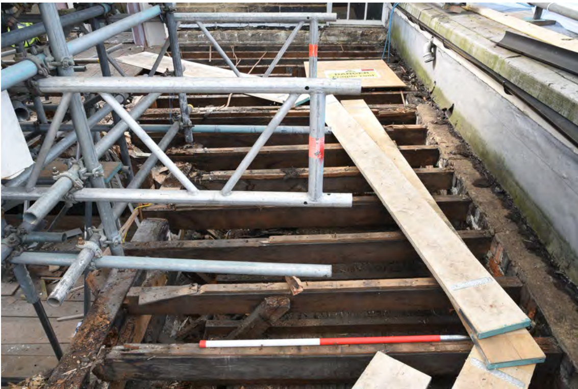
Plate E92 Roof construction following board lift, W side, looking S, scale 1.0m (BRH129)
