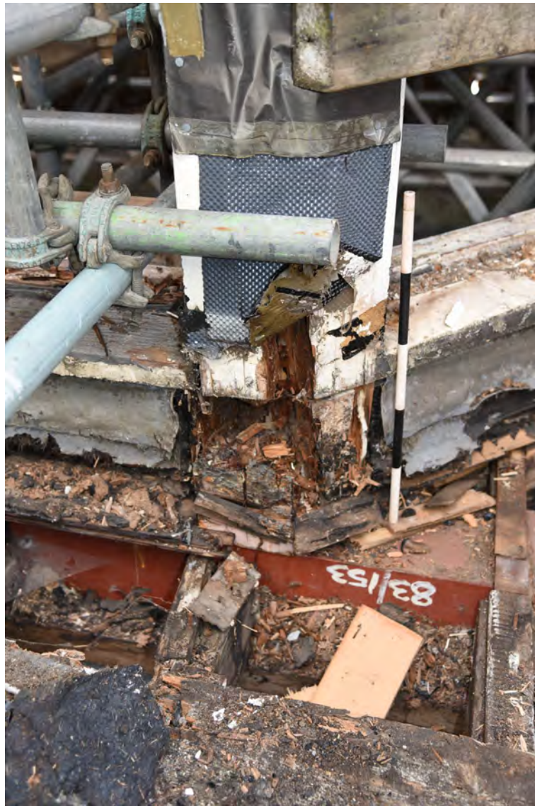
Plate E180 External window frame upright timber showing decay, looking W, scale 50cm (BRH089)
