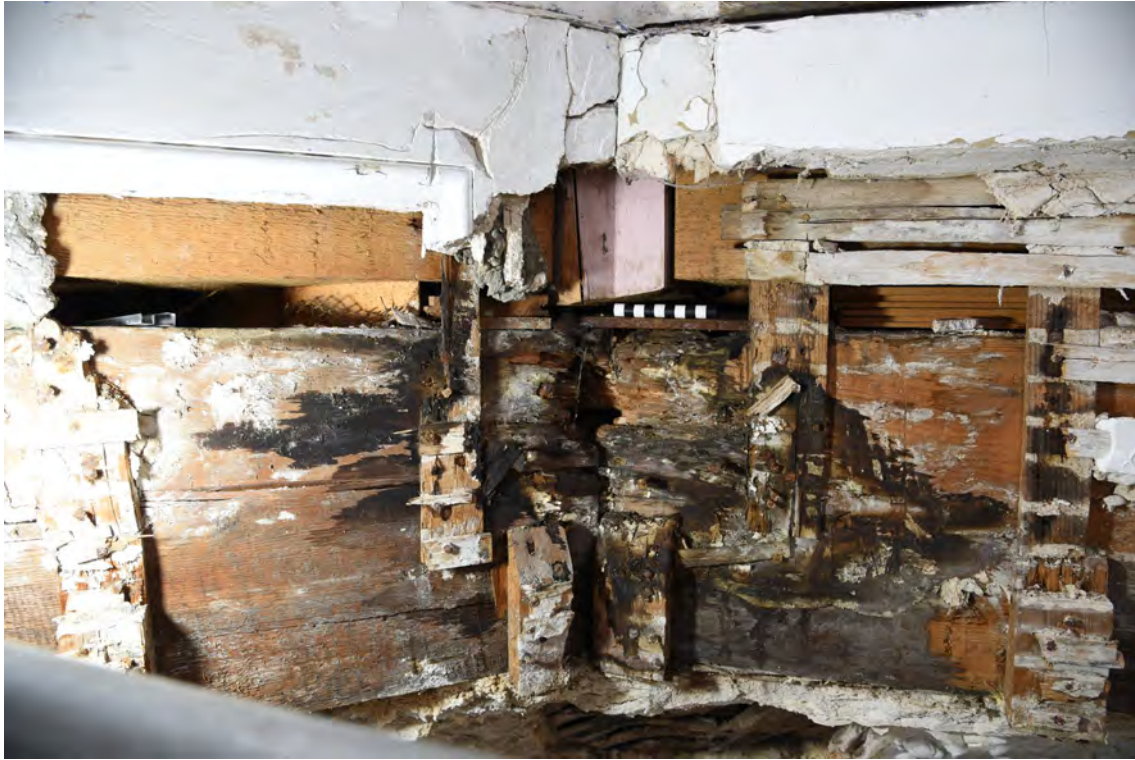
Plate E75 Detail of exposed timberwork of lantern base at junction between SE and S elevations showing decay, looking S, scale 10cm (BRH057)
