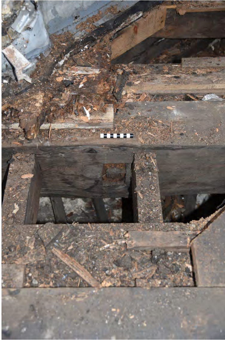
Plate E113 Detail – Ironwork bolt fastening through double tie beams to the northwest of the lantern, looking S, scale 10cm (BRH093)
