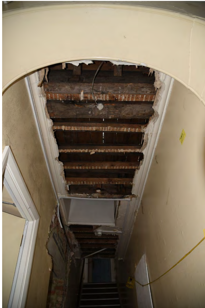
Plate E42 Internal view into vestibule roof space from east corridor at second floor level showing joists, tie-beam and E skylight, looking S (BRH220)
