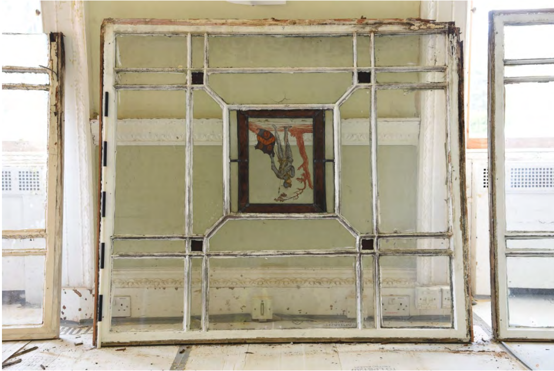
Plate E143 Window panel removed from the lantern's SE elevation, interior view, looking - (BRH181)
