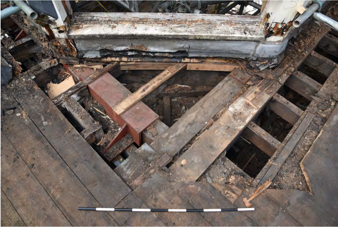
Plate E171 View into roof space following board lift showing modern steel repairs, looking SW, scale 1.0m (BRH080)
