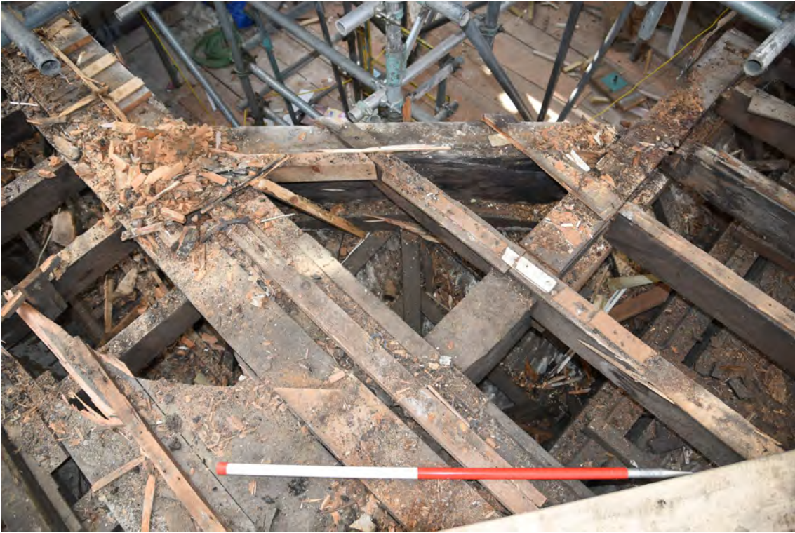
Plate E101 NW elevation lantern base and vestibule roof construction, looking SE, scale 1.0m (BRH138)
