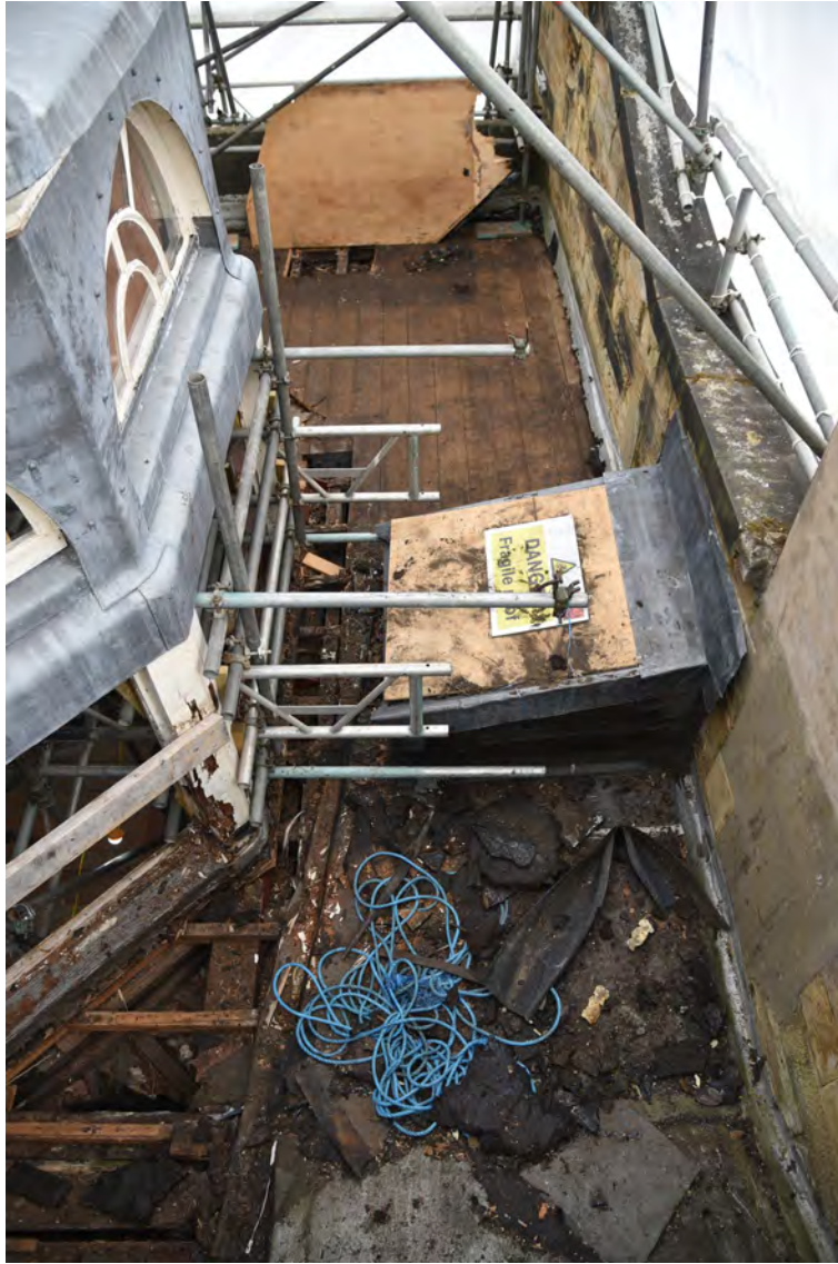
Plate E205 Flat-roof boards after removal of felt/bitumen, E side, looking N (BRH115)
