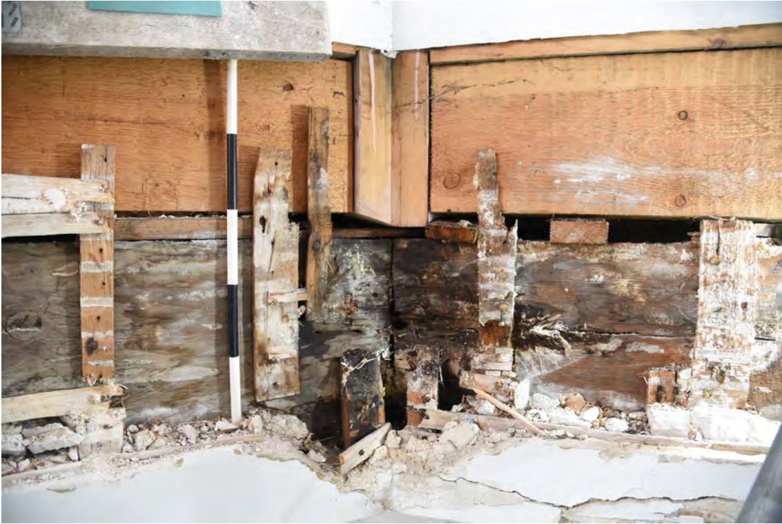
Plate E71 Detail of exposed timberwork of lantern base at junction between N and NE elevations showing decay, looking NE, scale 50cm (BRH053)
