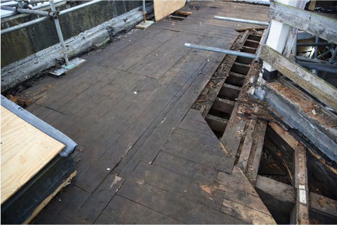
Plate E203 Flat-roof boards after removal of felt/bitumen, N side, looking NE (BRH113)
