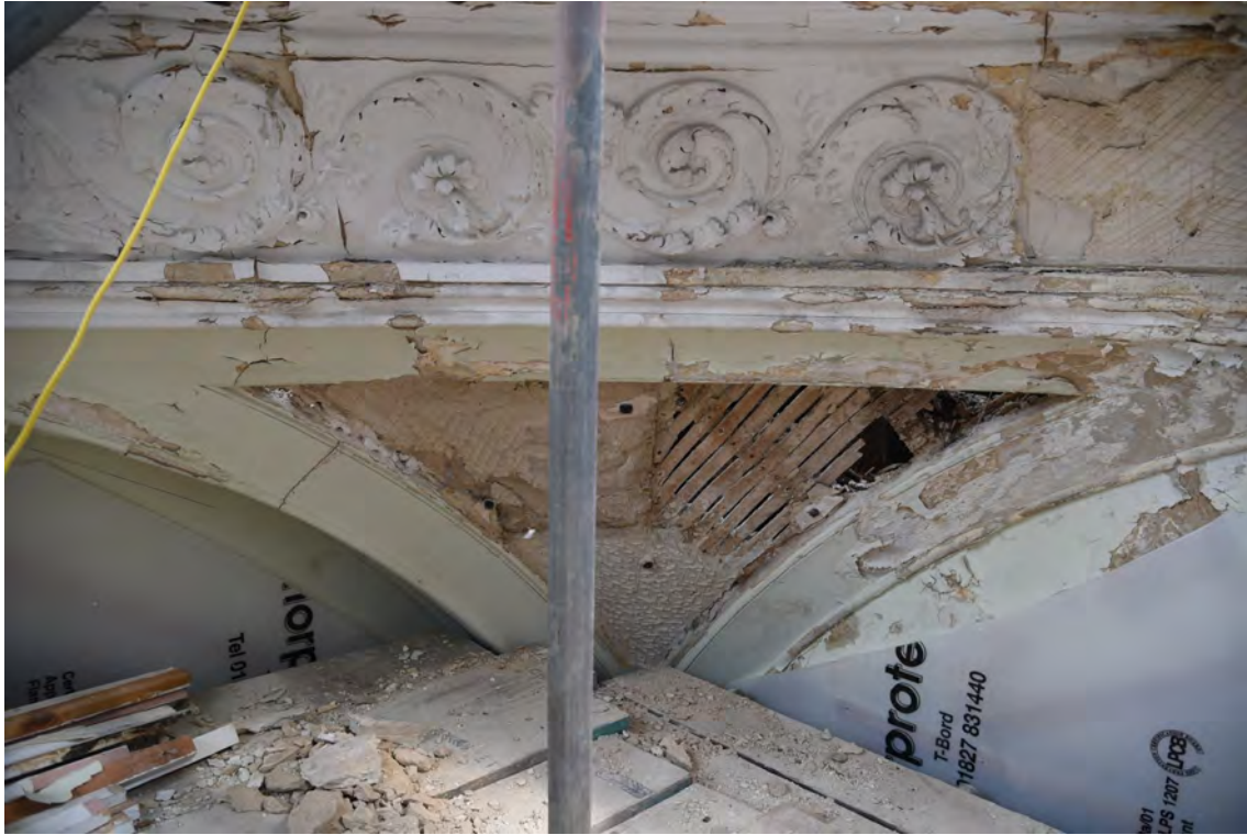
Plate E47 NE pendentive following removal of decorative plasterwork showing keying patterns and lathwork, looking NE (BRH157)
