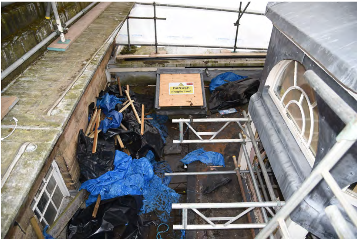
Plate E162 Vestibule flat roof and SW skylight before works, looking W (BRH018)
