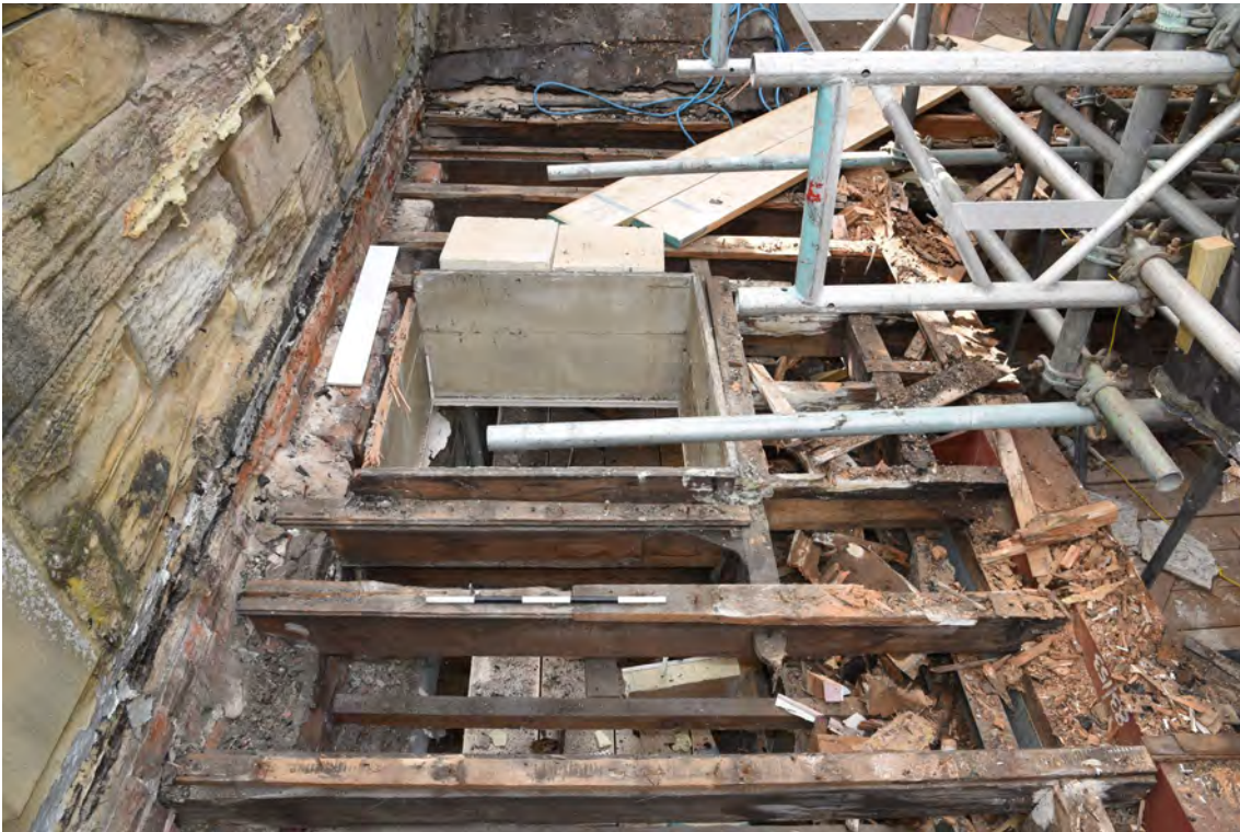
Plate E220 Eastern skylight following opening-up works, looking S, scale 50cm (BRH154)
