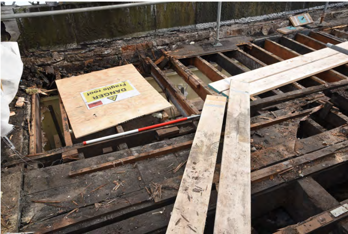
Plate E84 Roof construction following board lift, NW side, looking NE, scale 1.0m (BRH121)
