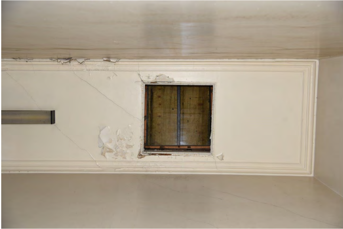
Plate E37 Internal view of vestibule roof SW skylight from the west corridor (BRH215)
