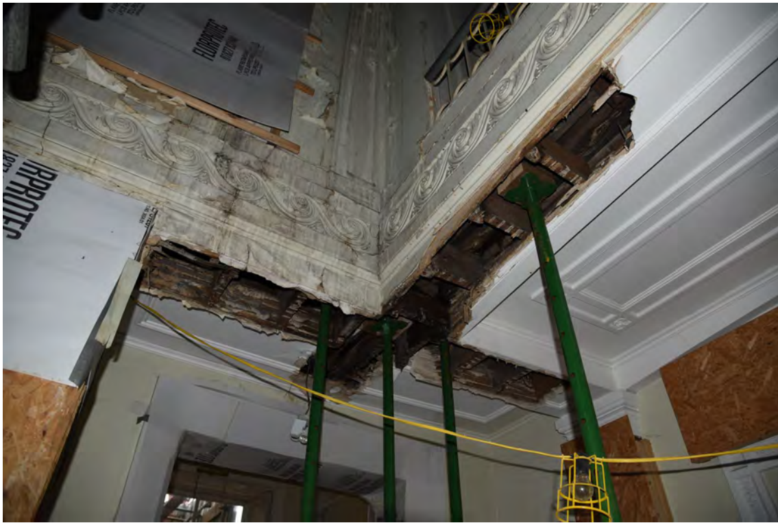
Plate E25 Detail of ground floor ceiling opening-up works, looking E (BRH203)
