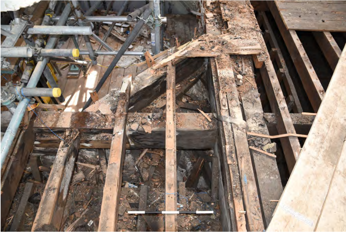
Plate E103 View showing roof construction SW pendentive, looking E, scale 50cm (BRH140)
