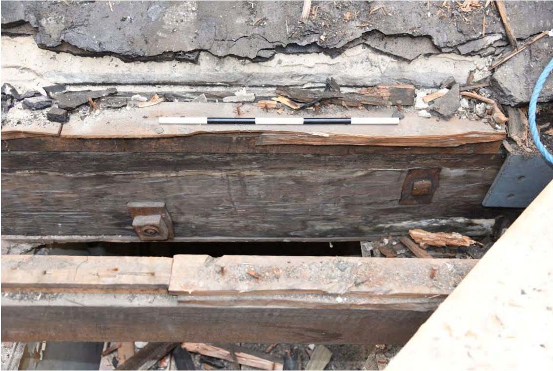
Plate E114 Iron bolt fastenings through double tie-beam in SE corner of the vestibule roof space, looking S, scale 50cm (BRH160)
