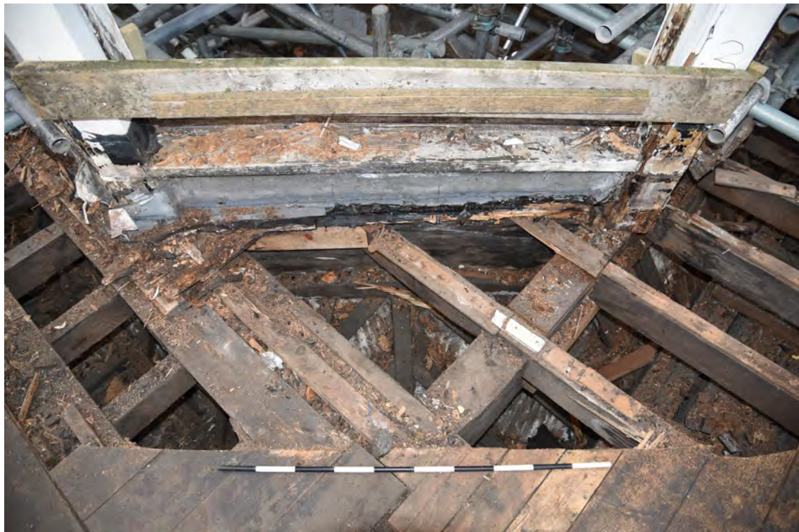
Plate E176 Lantern base, tie beams and roof joists, NW side, looking SE, scale 1.0m (BRH085)
