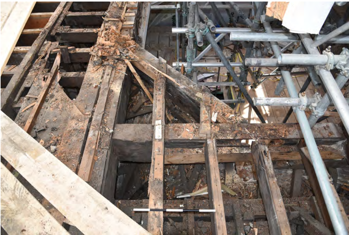
Plate E104 View showing roof construction NW pendentive, looking E, scale 50cm (BRH141)
