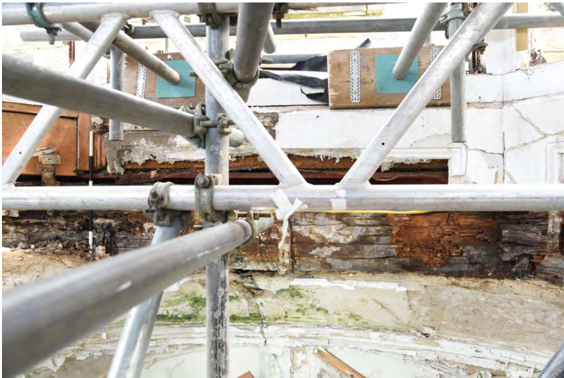
Plate E64 Interior view, exposed timbers of lantern base, looking E, scale 50cm (BRH037)
