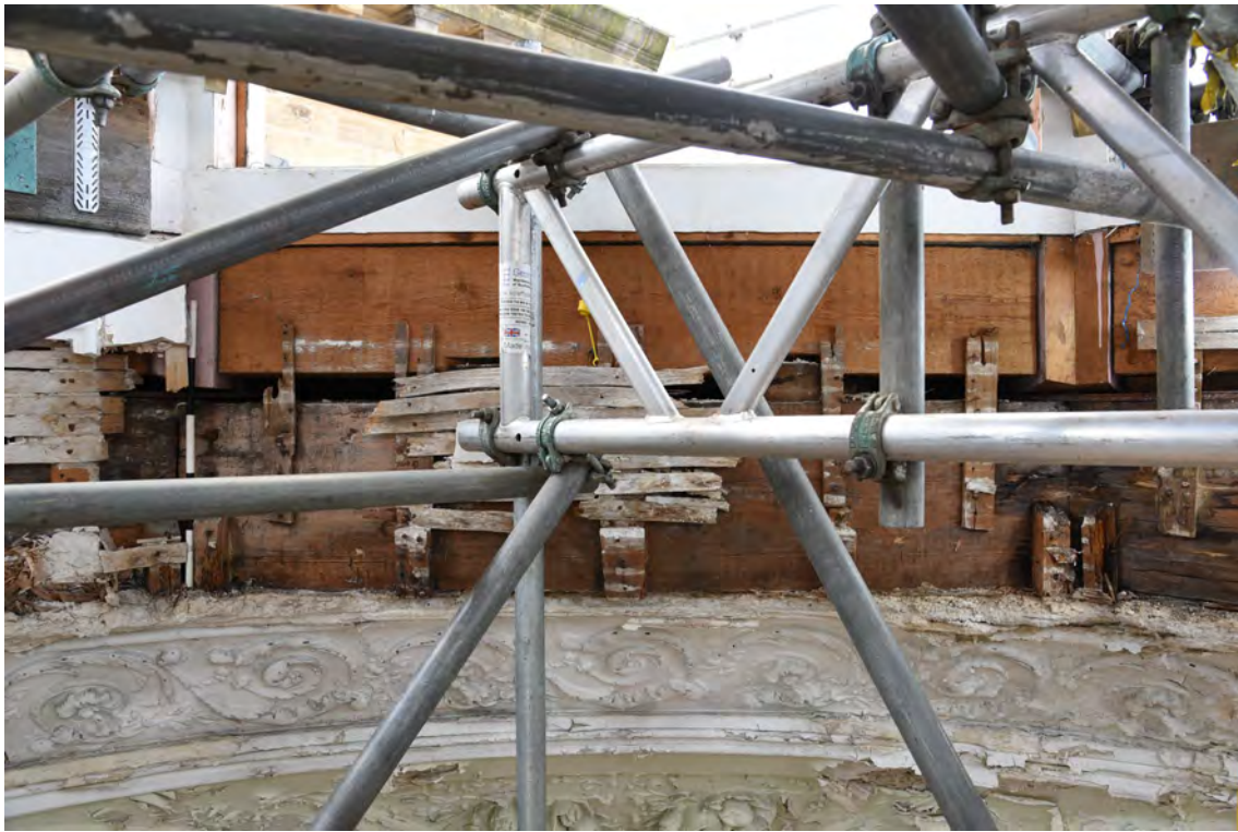
Plate E67 Interior view, exposed timbers of lantern base, looking SW, scale 50cm (BRH040)
