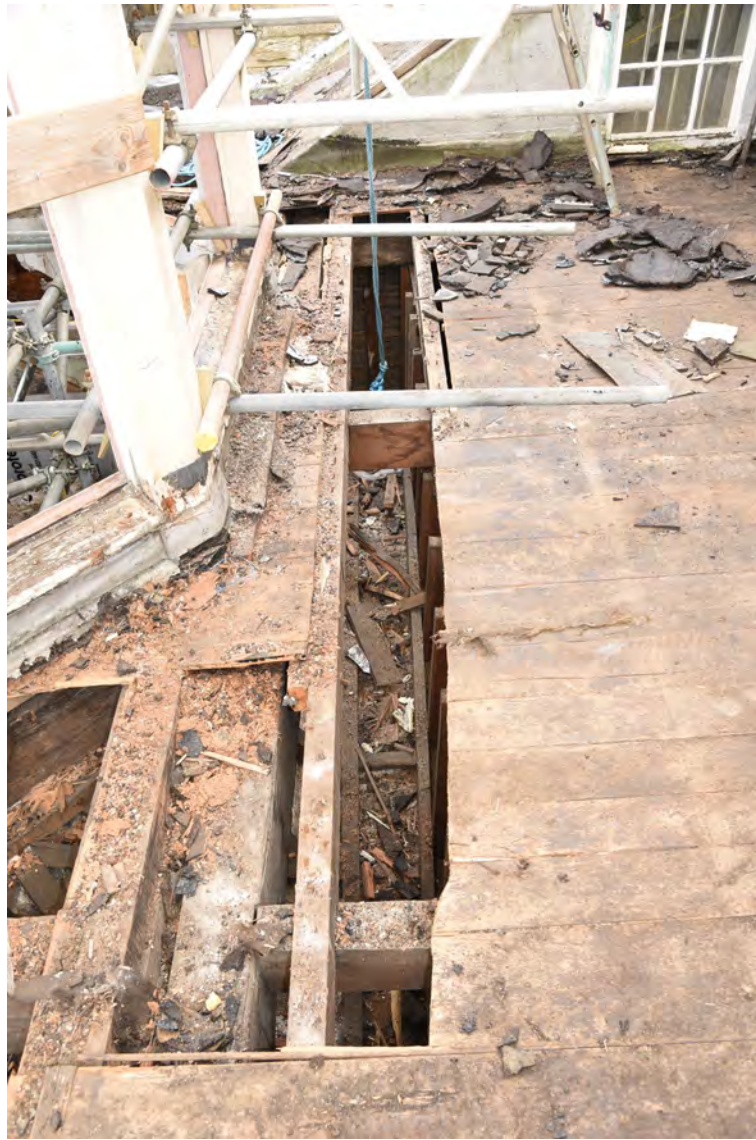
Plate E204 View into roof space showing arch construction, looking E (BRH114)
