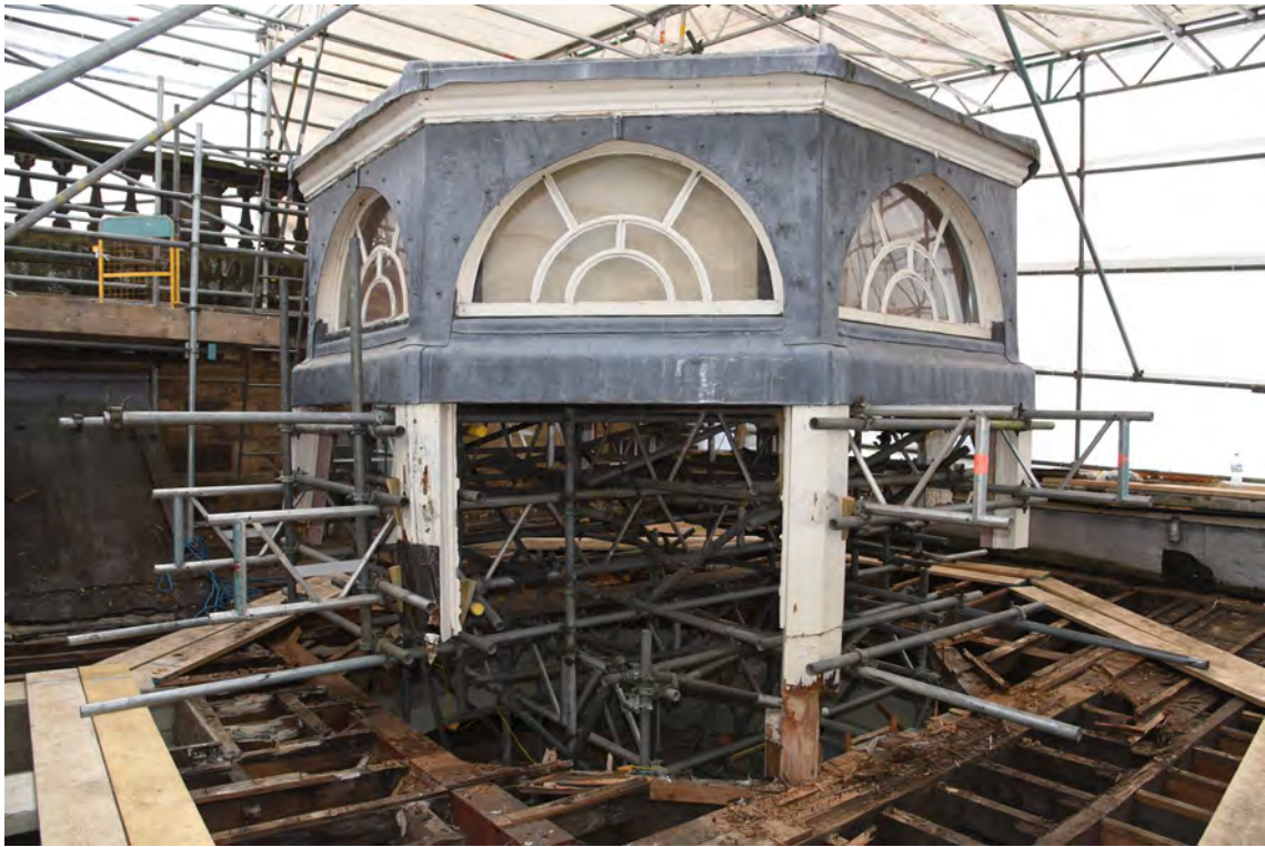
Plate E211 View of lantern and vestibule roof during works, looking SW (BRH167)
