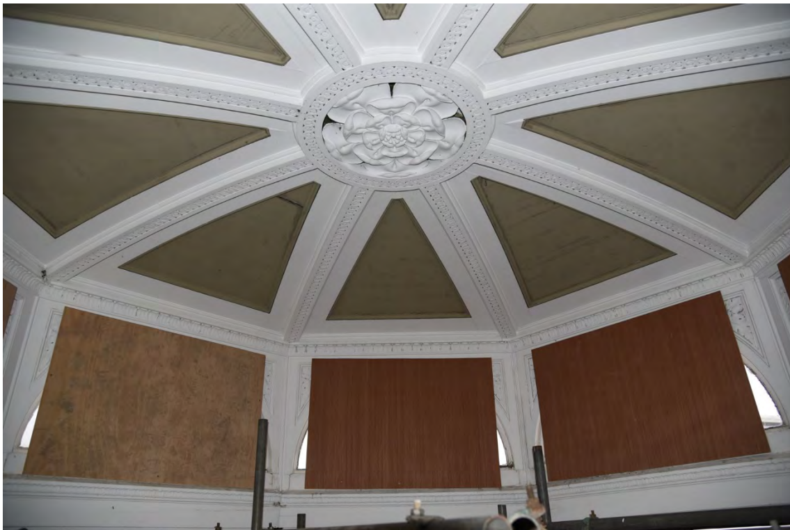
Plate E130 View into the lantern ceiling space looking W, looking W (BRH078)
