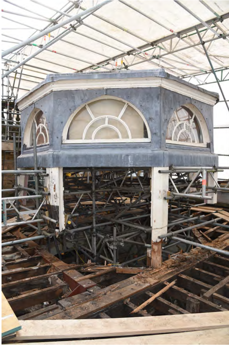
Plate E210 View of lantern and vestibule roof during works, looking SW (BRH166)
