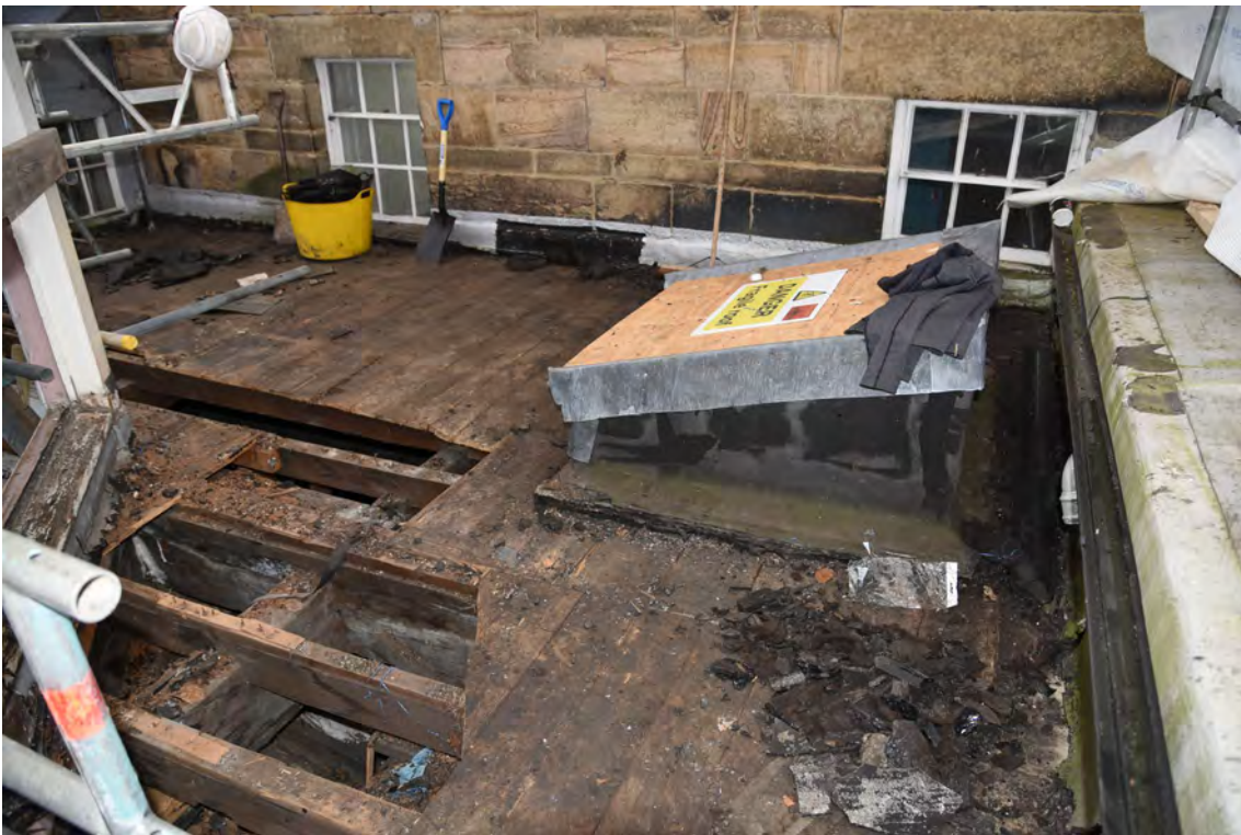
Plate E200 Flat-roof boards after removal of felt/bitumen, SW side, looking SE (BRH110)
