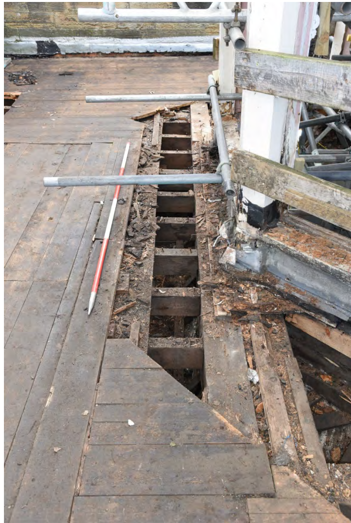
Plate E175 View of roof joists and tie beam following board lift, looking E, scale 1.0m (BRH084)
