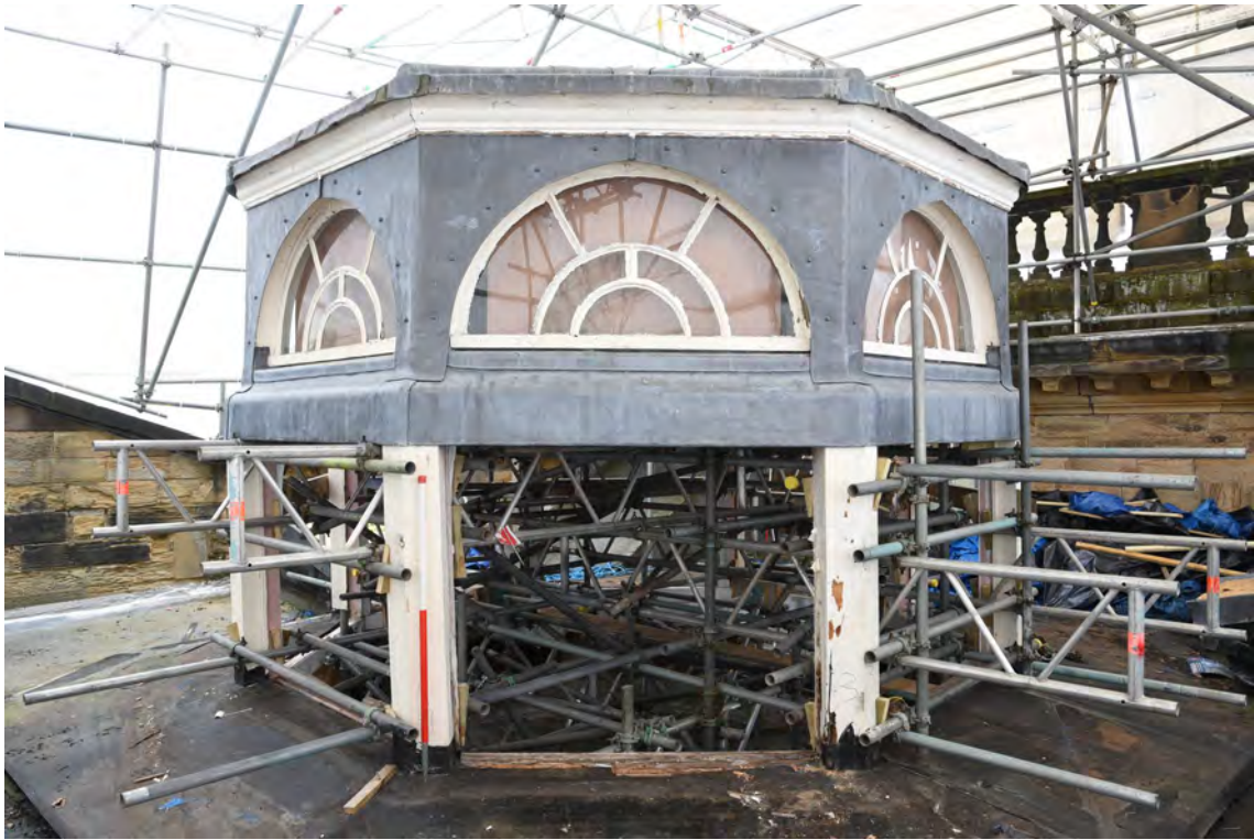
Plate E51 General view of lantern looking SE during works, looking SE, scale 1.0m (BRH007)
