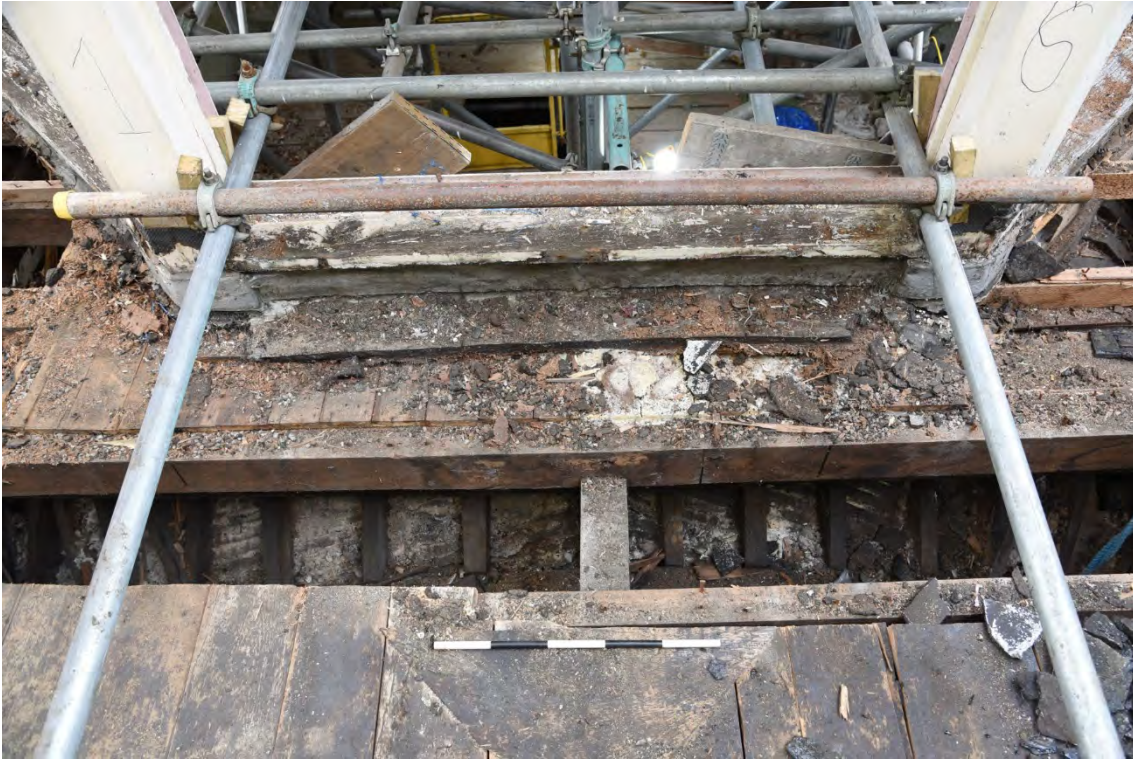
Plate E193 Lantern base, tie beam and roof joists, S side, looking N, scale 50cm (BRH103)
