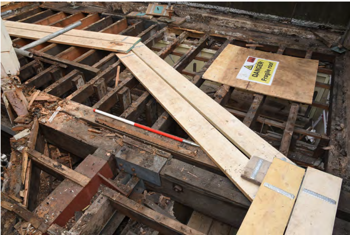
Plate E88 Roof construction following board lift, NE side, looking NW, scale 1.0m (BRH125)
