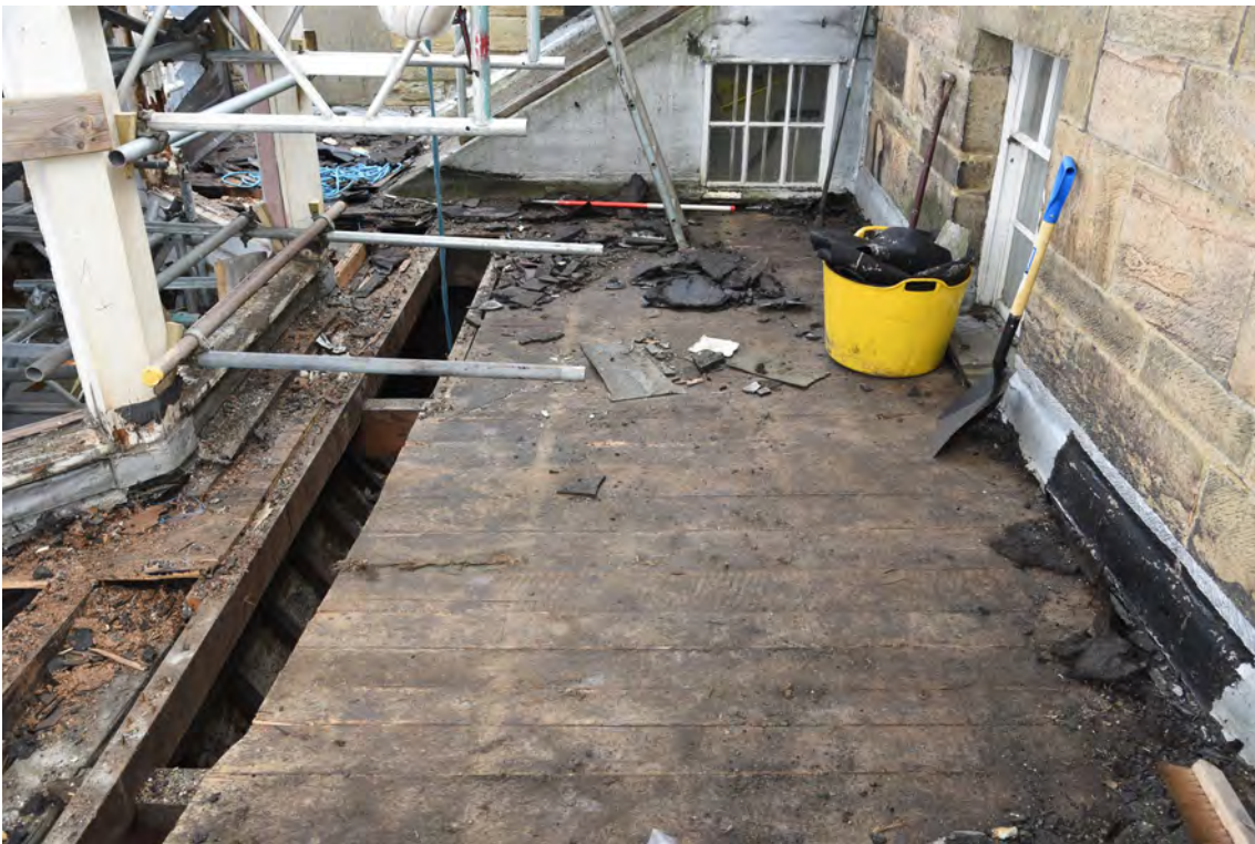
Plate E194 Flat-roof boards after removal of felt/bitumen, S side, looking E, scale 1.0m (BRH104)
