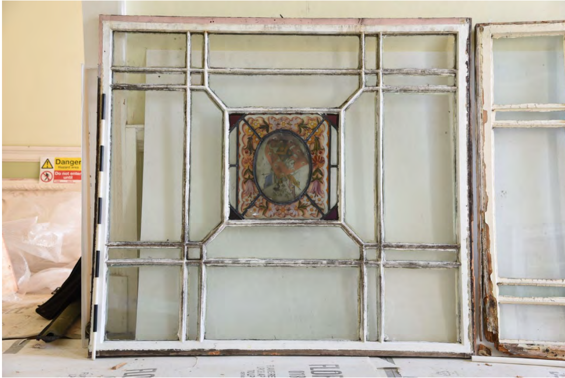
Plate E131 Window panel removed from the lantern's N elevation, interior view (BRH169)
