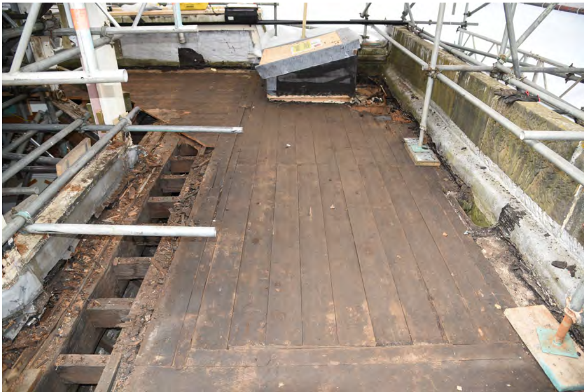
Plate E196 Flat-roof boards after removal of felt/bitumen, N side, looking W (BRH106)
