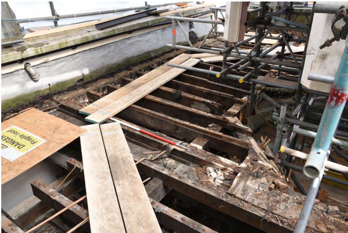
Plate E82 Roof construction following board lift, SW side, looking NW, scale 1.0m (BRH119)
