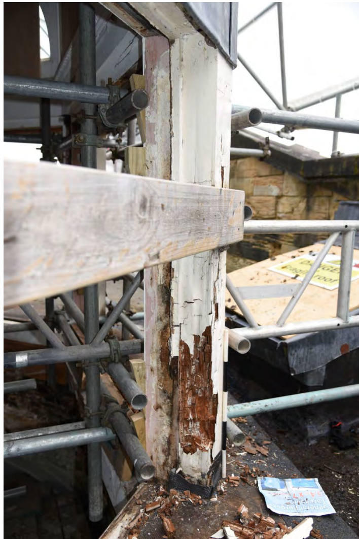
Plate E110 External window frame upright timber showing decay, looking NE, scale 50cm (BRH073)
