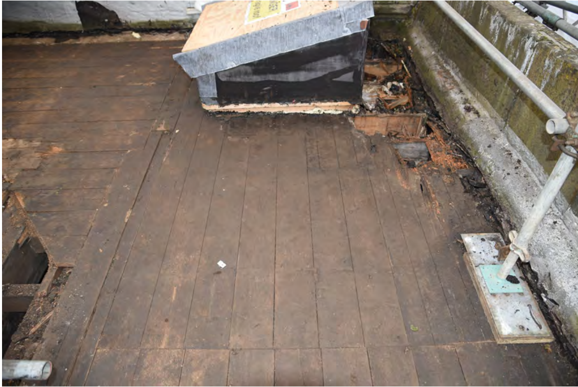
Plate E197 Flat-roof boards after removal of felt/bitumen, N side, looking W (BRH107)
