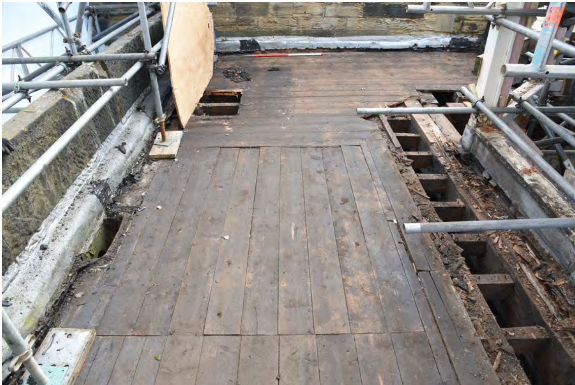
Plate E178 Flat-roof boards after removal of felt/bitumen, N side, looking E, scale 1.0m (BRH087)
