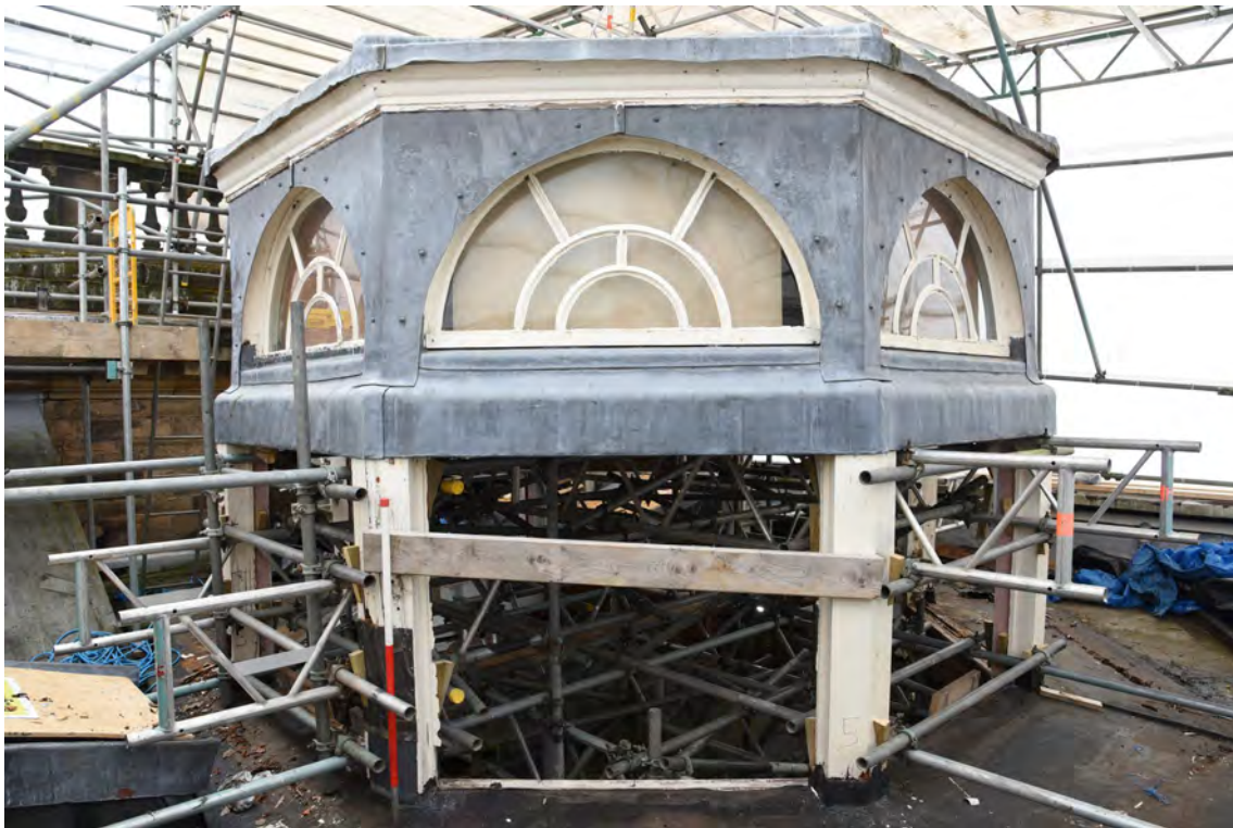
Plate E50 General view of lantern looking SW during works, looking SW, scale 1.0m (BRH006)
