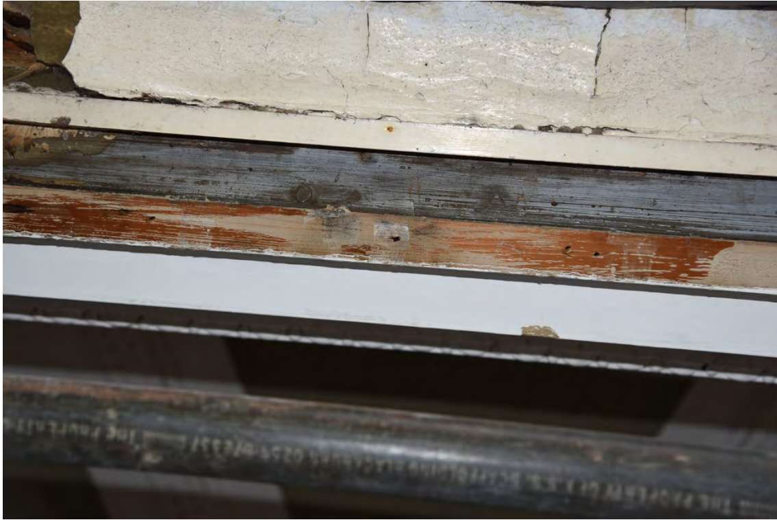
Plate E123 Lantern E elevation – Carpenters’ mark inside top of window frame = V (BRH069)
