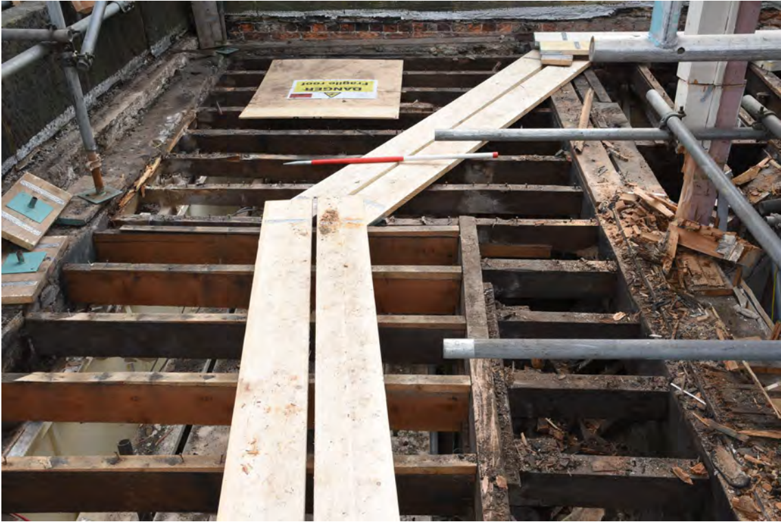
Plate E85 Roof construction following board lift, NW side, looking N, scale 1.0m (BRH122)
