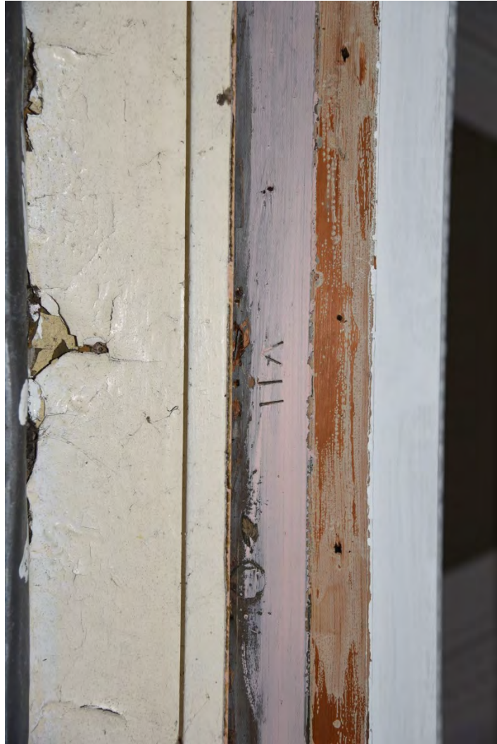
Plate E125 Lantern N elevation – Carpenters' mark inside top of window frame = VII (BRH071)
