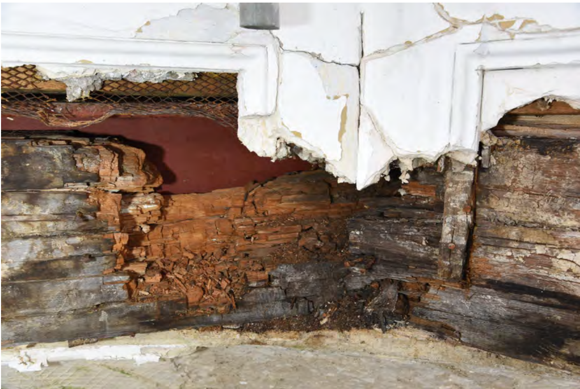
Plate E74 Detail of exposed timberwork of lantern base at junction between E and SE elevations showing decay, looking SE (BRH056)
