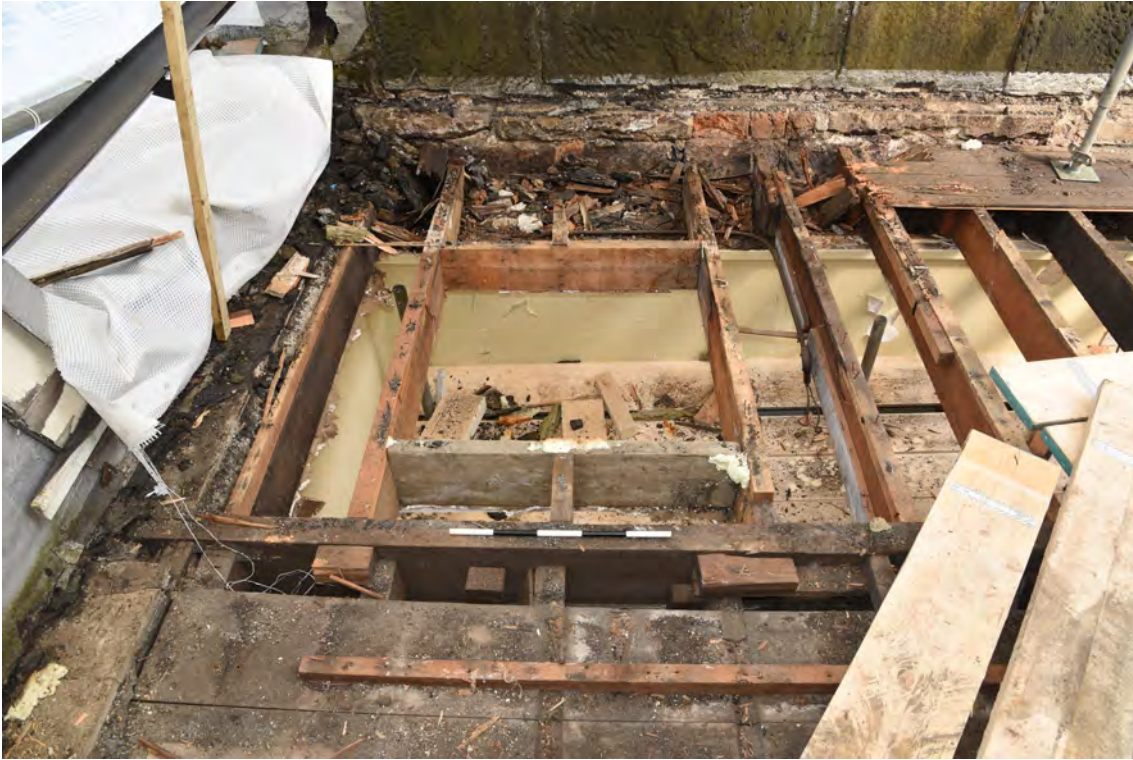
Plate E217 NW skylight following opening-up works, looking N, scale 50cm (BRH151)
