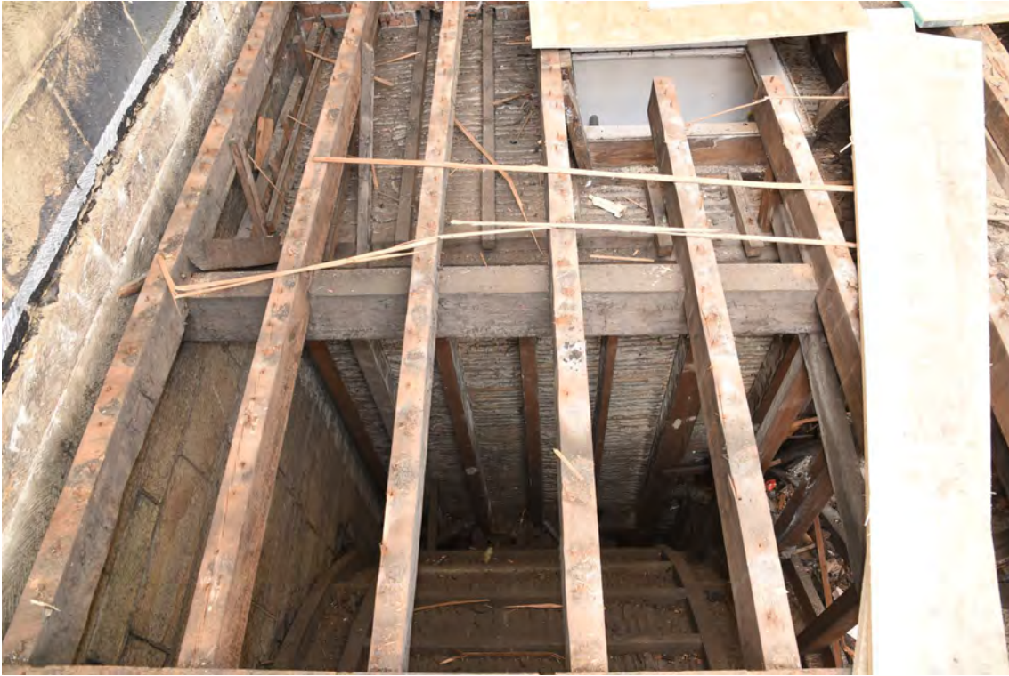
Plate E213 View into roof space overlying arch connecting vestibule with the staircase, looking W (BRH147)
