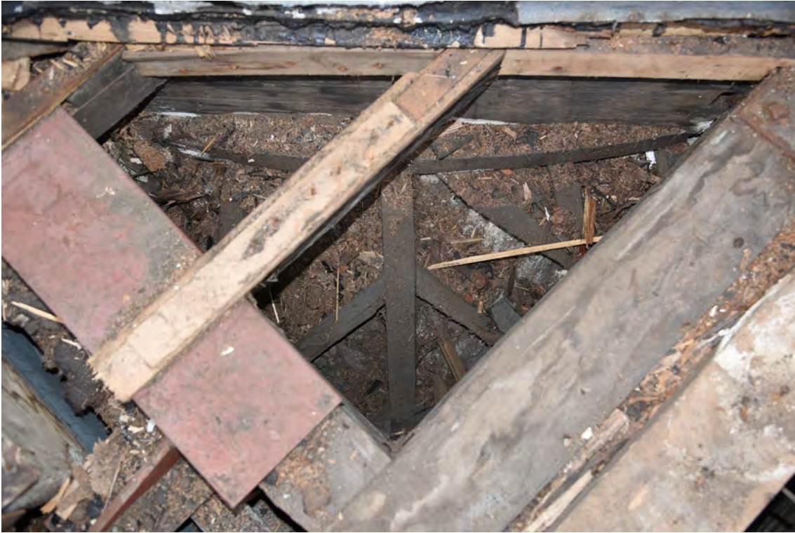
Plate E183 View into roof space overlying the NE pendentive illustrating construction, looking SW (BRH092)
