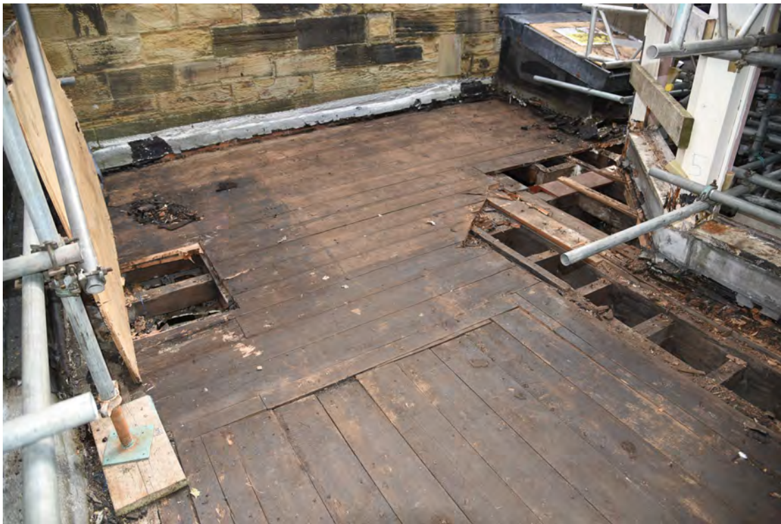
Plate E198 Flat-roof boards after removal of felt/bitumen, NE side, looking E (BRH108)
