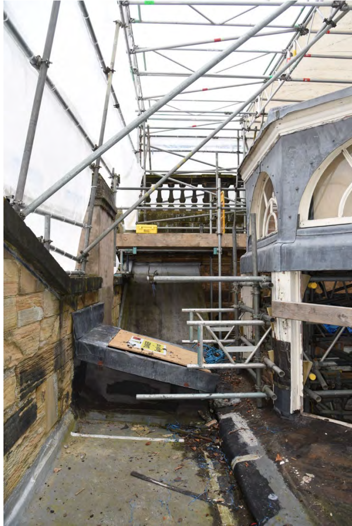
Plate E169 General view vestibule roof and E skylight, E of lantern, looking S (BRH025)
