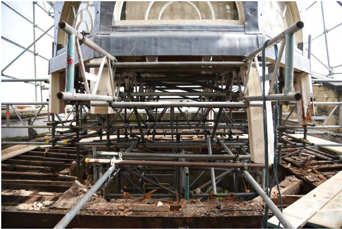
Plate E81 View of lantern following removal of rotten timbers, looking N (BRH118)
