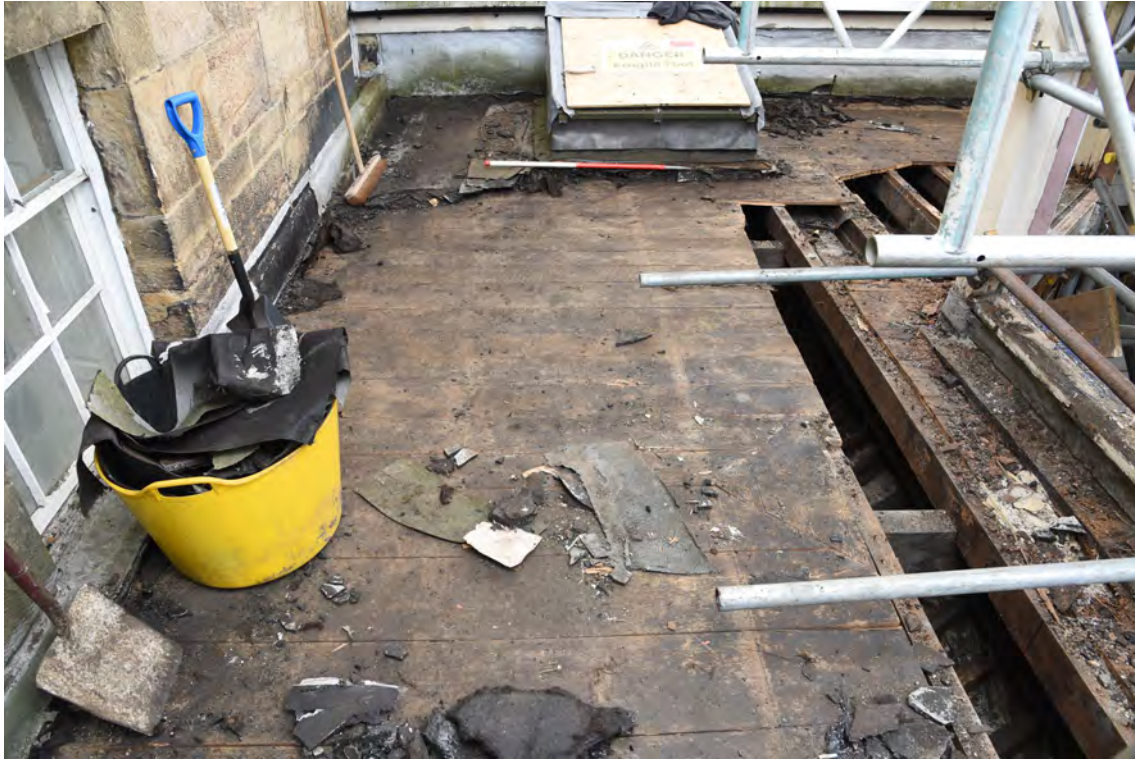
Plate E195 Flat-roof boards after removal of felt/bitumen, S side, looking W, scale 1.0m (BRH105)
