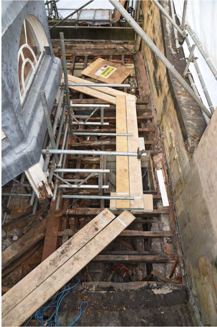
Plate E208 General view of flat roof following opening-up works, looking N (BRH164)
