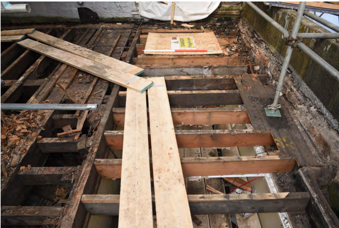
Plate E90 Roof construction following board lift, N side, looking W, scale 1.0m (BRH127)
