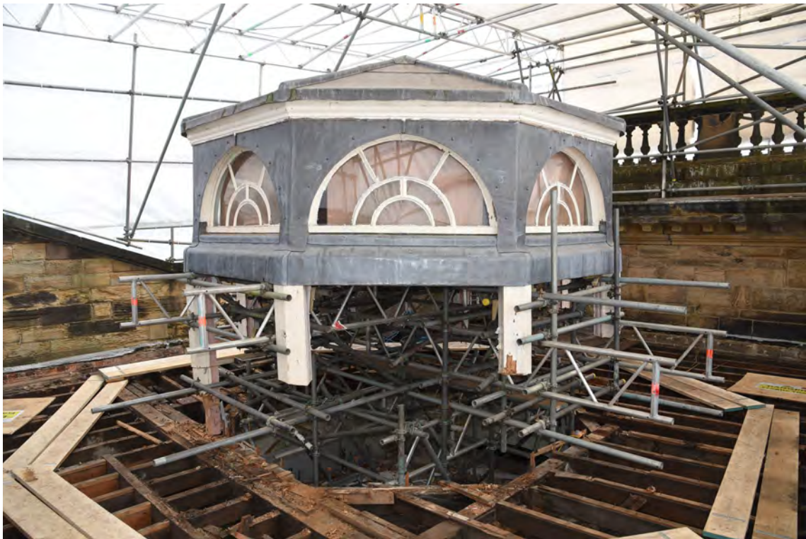
Plate E212 View of lantern and vestibule roof during works, looking SE (BRH168)
