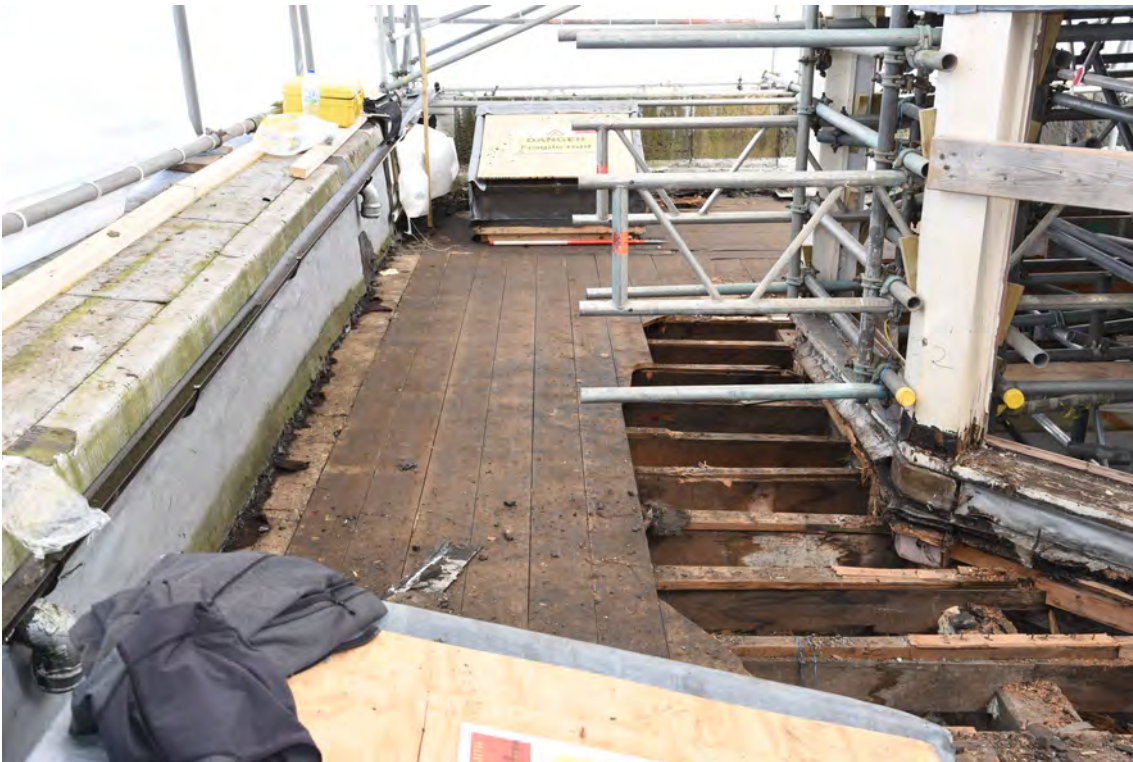
Plate E190 Flat-roof boards after removal of felt/bitumen, W side, looking N, scale 1.0m (BRH100)
