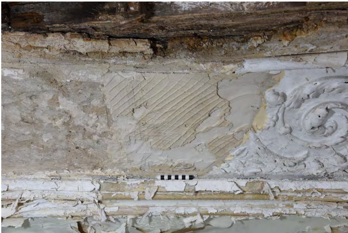
Plate E76 Detail - Removal of decorative plasterwork revealing keying pattern beneath, looking SE, scale 10cm (BRH058)
