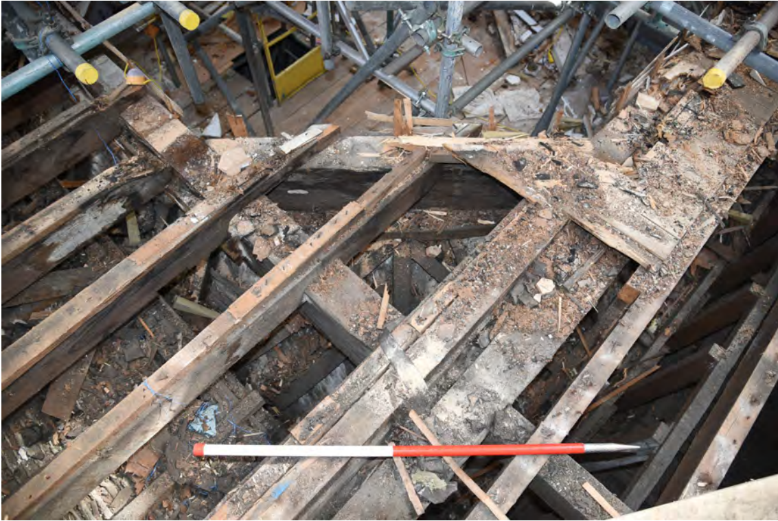
Plate E99 SW elevation lantern base and vestibule roof construction, looking NE, scale 1.0m (BRH136)
