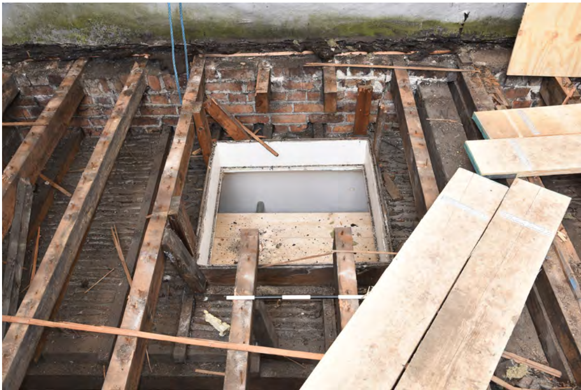
Plate E216 SW skylight following opening-up works, looking W, scale 50cm (BRH150)
