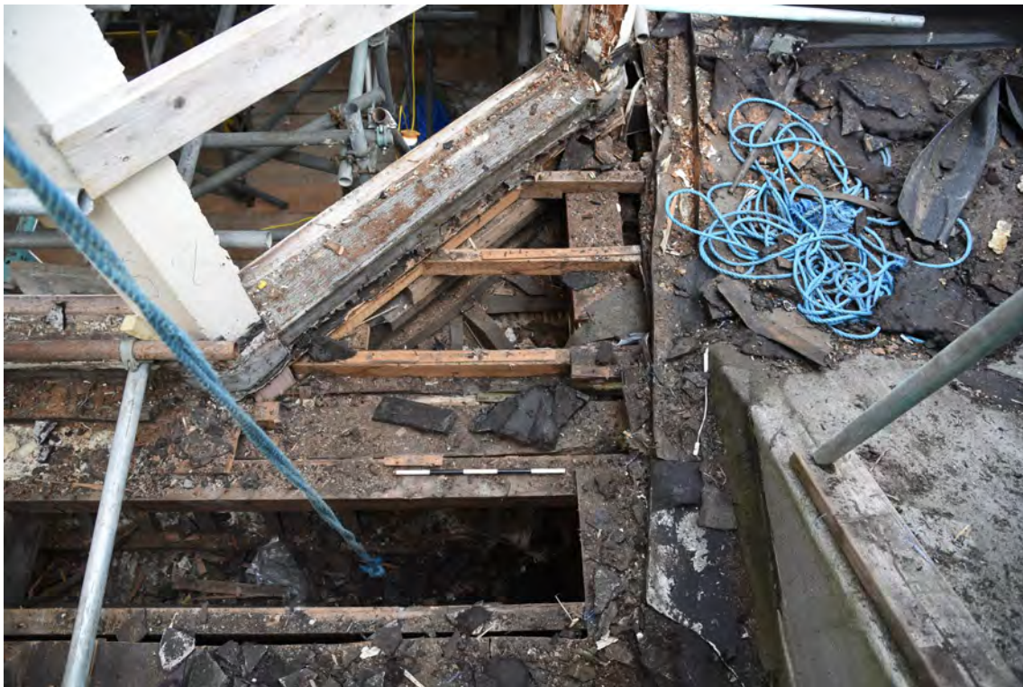
Plate E192 Lantern base, tie beam and roof joists, SE side, looking N (BRH102)
