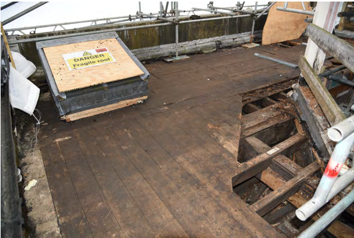
Plate E202 Flat-roof boards after removal of felt/bitumen, NW side, looking NE (BRH112)
