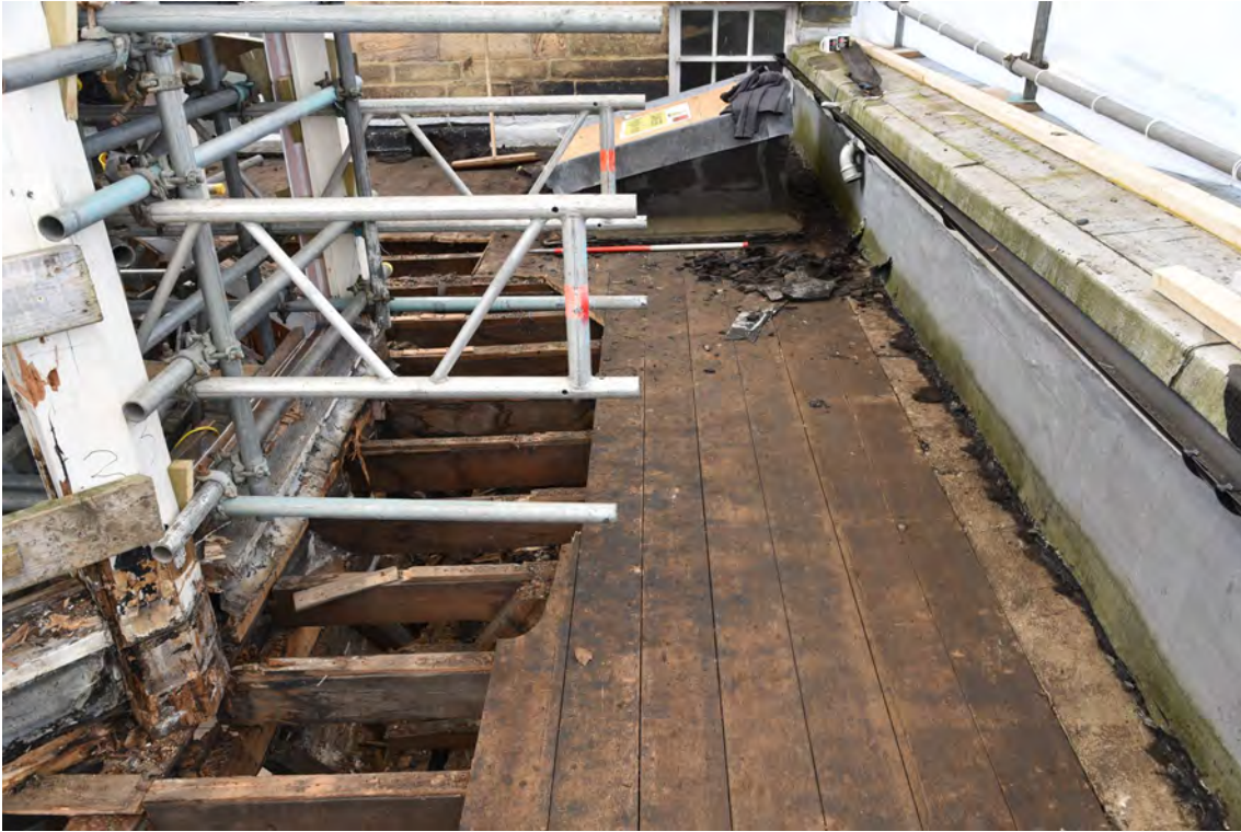
Plate E189 Flat-roof boards after removal of felt/bitumen, W side, looking S, scale 1.0m (BRH099)
