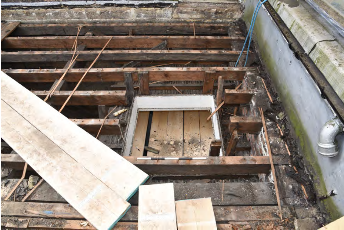
Plate E215 SW skylight following opening-up works, looking S, scale 50cm (BRH149)
