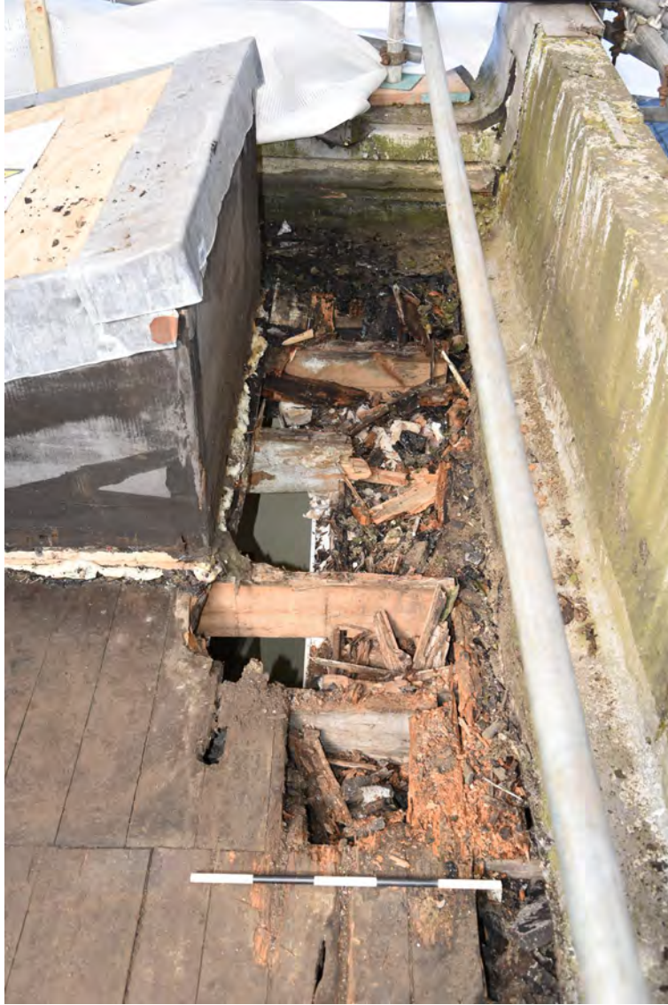
Plate E179 Flat-roof N of NW skylight showing timber decay, looking W, scale 1.0m (BRH088)
