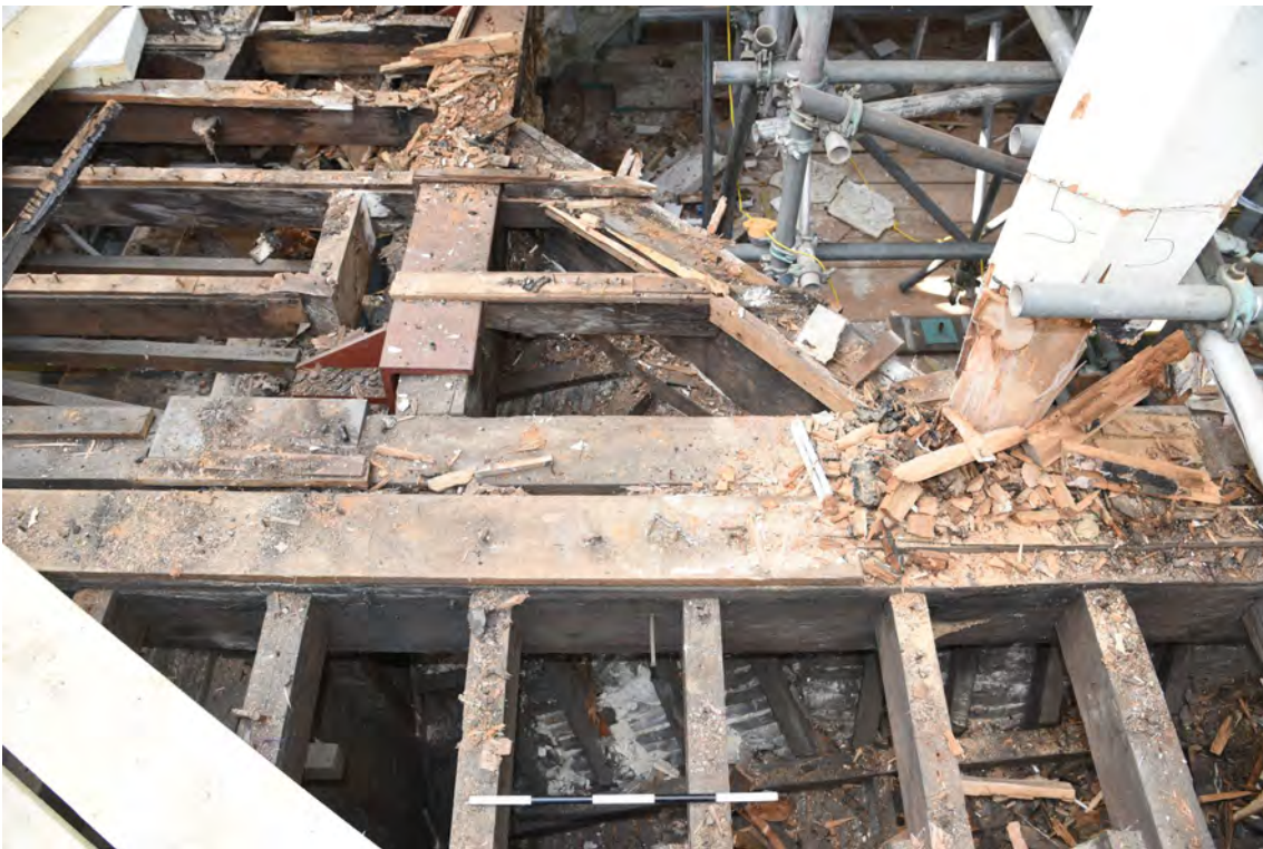
Plate E106 View showing roof construction NE pendentive, looking S, scale 50cm (BRH143)
