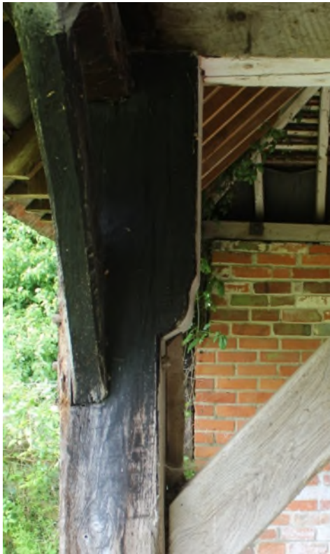
Figure 11 Post of Truss V showing the cyma recta moulding to the jowl.
