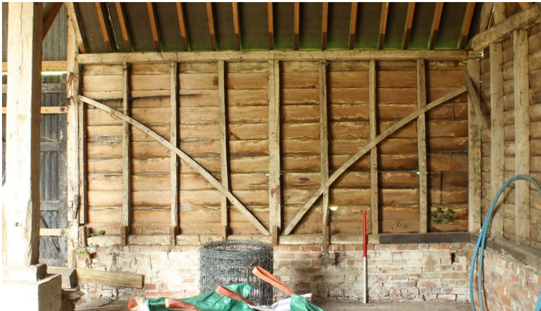
Figure 5 The wall framing to the aisle in Bay 1 showing the curved shores.
