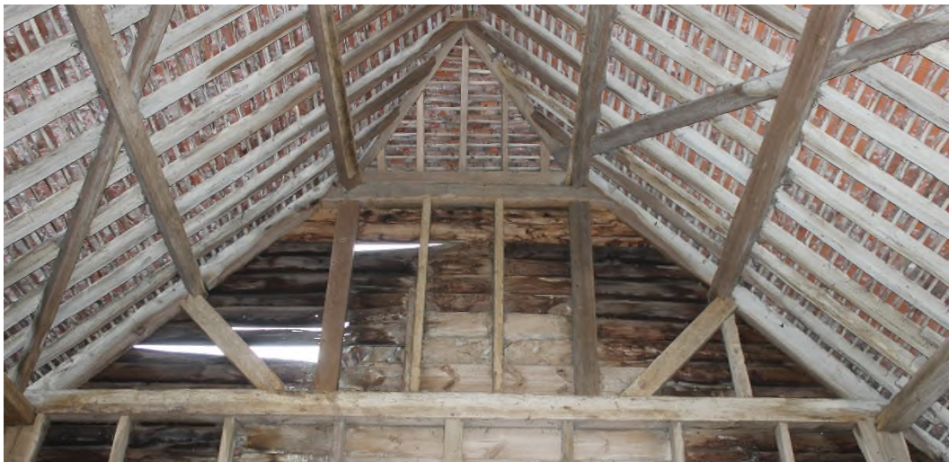
Figure 6 The roof truss of Truss I at the north end of the barn with queen and raking struts.
