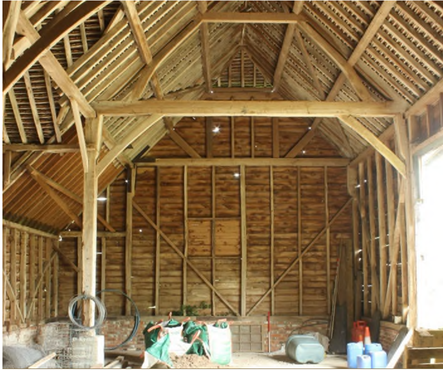
Figure 4 Barn interior facing north showing the wall framing of thin studs and long, raking shores.
