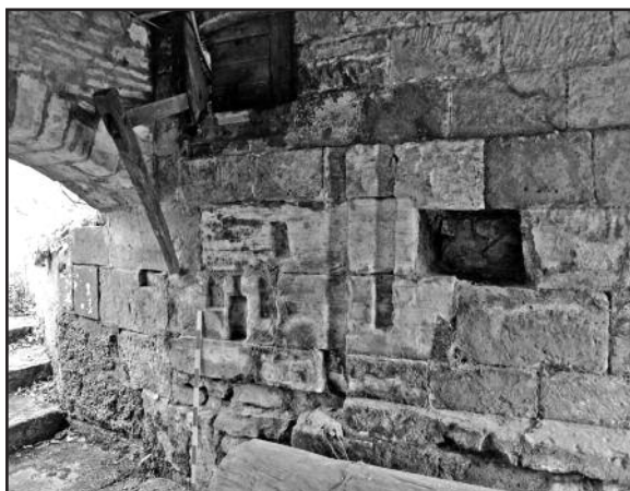
Internal view of the wheelhouse at Water Mill, Stone, showing re-used ashlar blocks © AS - WYAS
