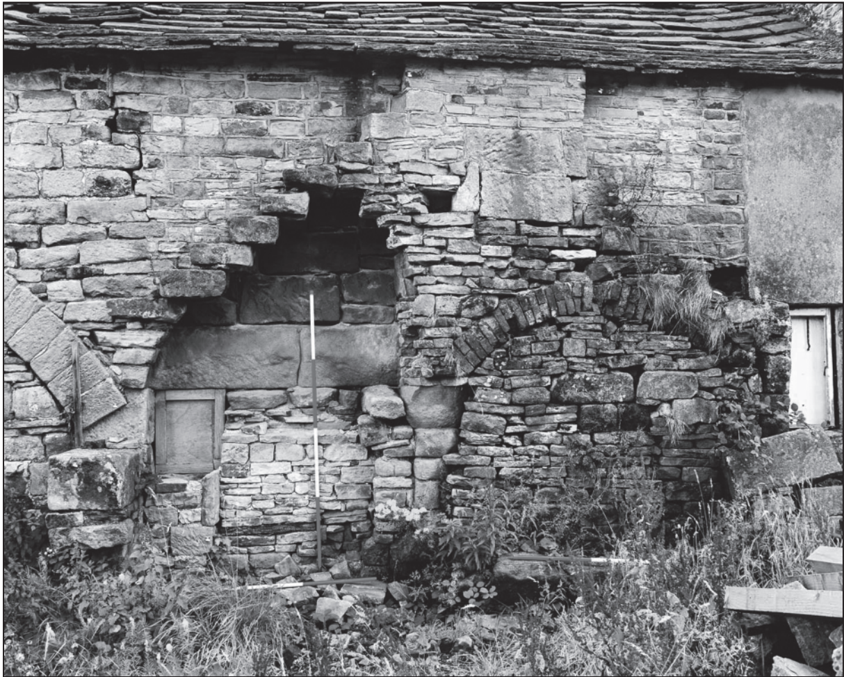
Exposed flue of annealing oven (lehr) chimney in west elevation of Bolsterstone glasshouse
