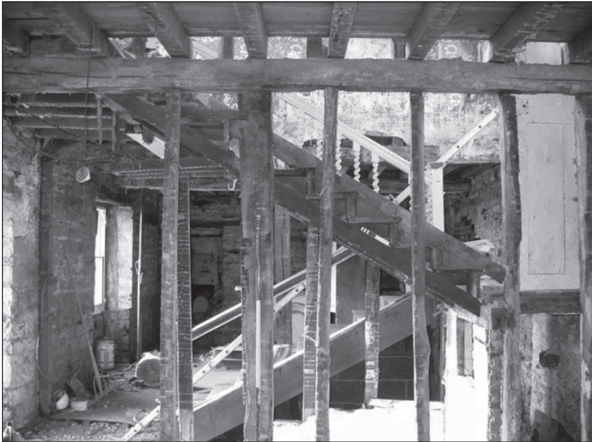
View of original staircase from the hall, following internal stripping, Grange Farm © Chris Scurfield
