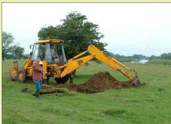
Undertaking excavations through the alluvial floodplain of the River Ure. Thick deposits of sands and silts bury older peaty sediments in many places
