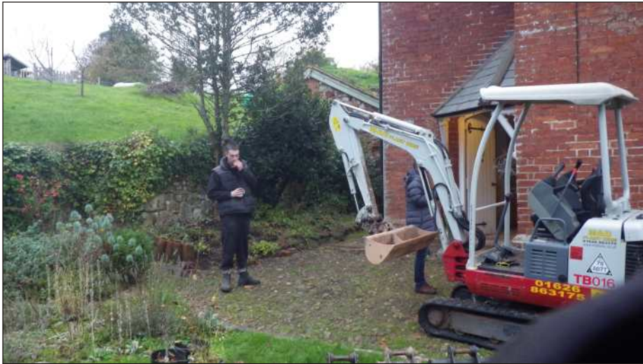
Plate 1: View of the site prior to the beginning of groundworks, view from the southeast
