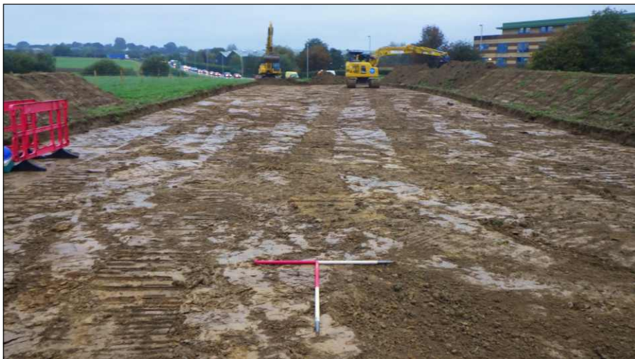
Plate 2: Area 2, work in progress, looking to the northwest (1m and 1m scale)
