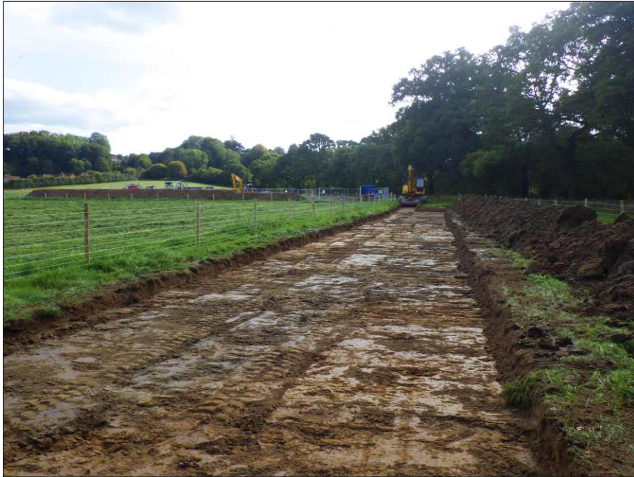
Plate 1: Area 1a, compound access track, work in progress, looking to the south
