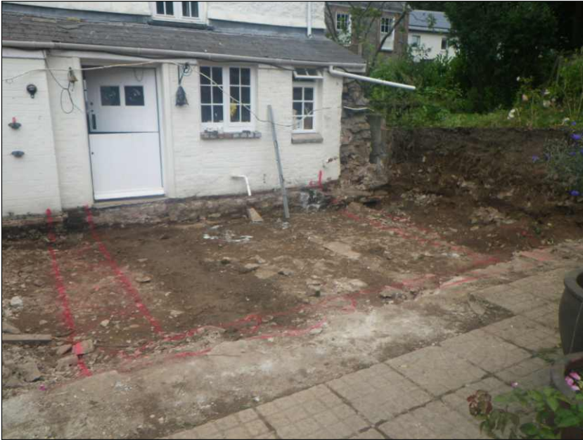
Plate 1: General view of site showing footing trench outline with demolished retaining wall in background. View to northeast
