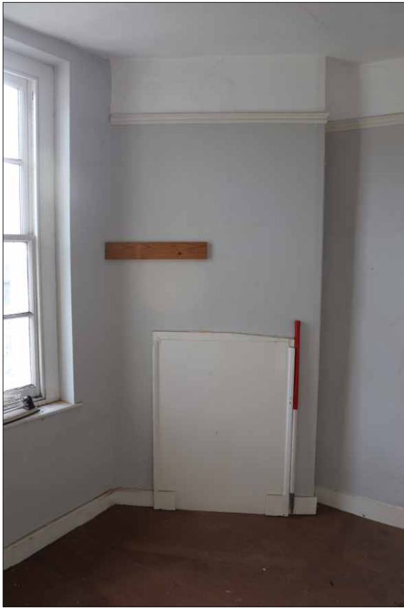
Plate 18: Southeast room on the second floor of No. 29, looking south (1m scale)
