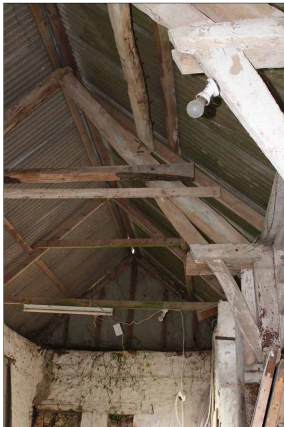
Plate 9: North side of truss 5 showing how the rafters are supported on this side, looking west
