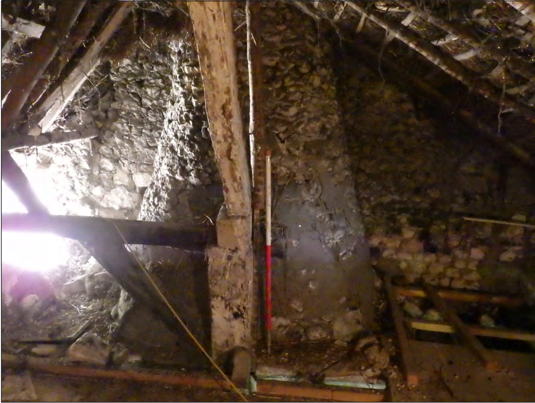
Plate 5: Truncated tie beam and brace of Period I building with inserted conical Phase III stack (scale 1m)
