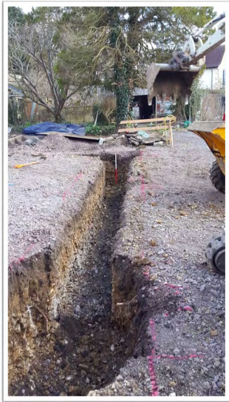
Plate 2: Excavated footing trench with expanded pad-base in foreground. View from the W
